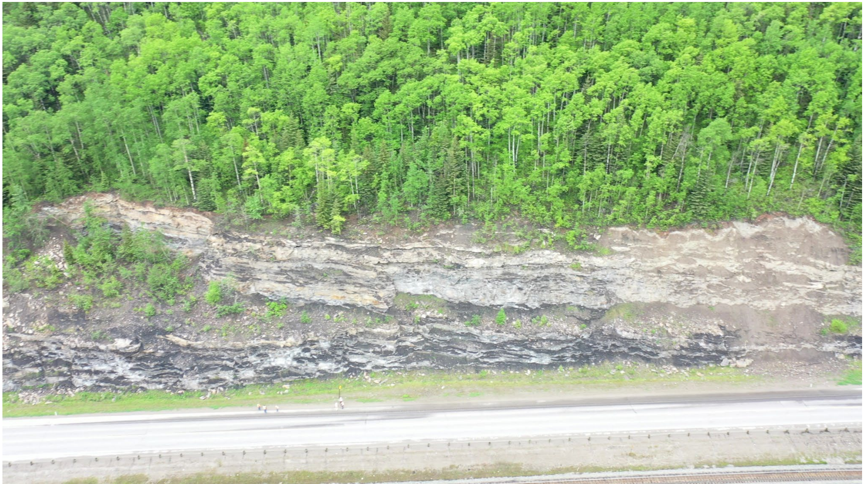
Photo 2 Rock cut slope along west side of Hwy 40:36. Note mid-slope bench and talus cones/slopes could potentially bounce/launch/roll rockfall particles out onto highway. Photo taken June 14, 2022, facing west.
