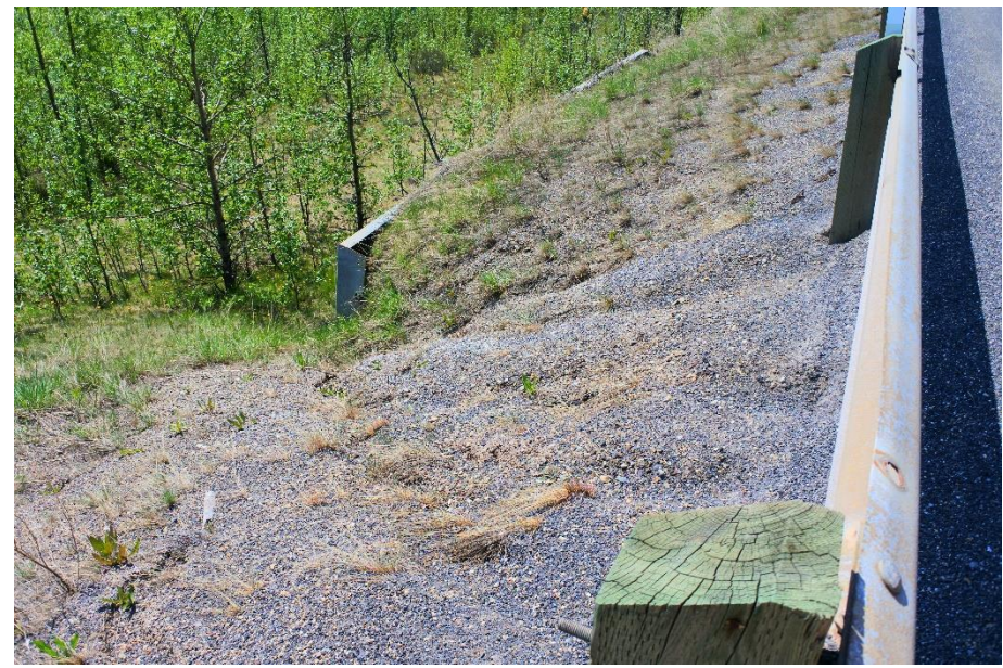
Photo 6. Looking at some surficial erosion that occurred above bin wall on north side.
