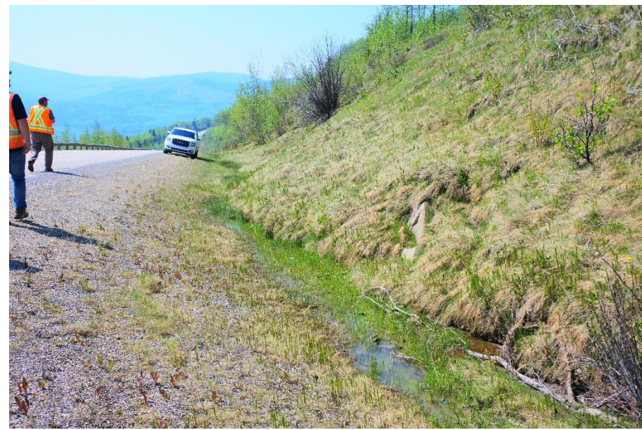
Photo 7. Looking south at the backslope ditch with water ponding.
