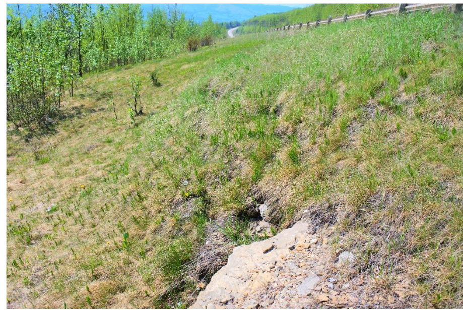
Photo 1. Looking south at subdued scarp slightly west of the main scarp.
