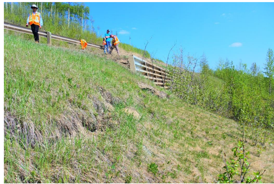
Photo 3. Looking north at scarp extending towards the bin wall.
