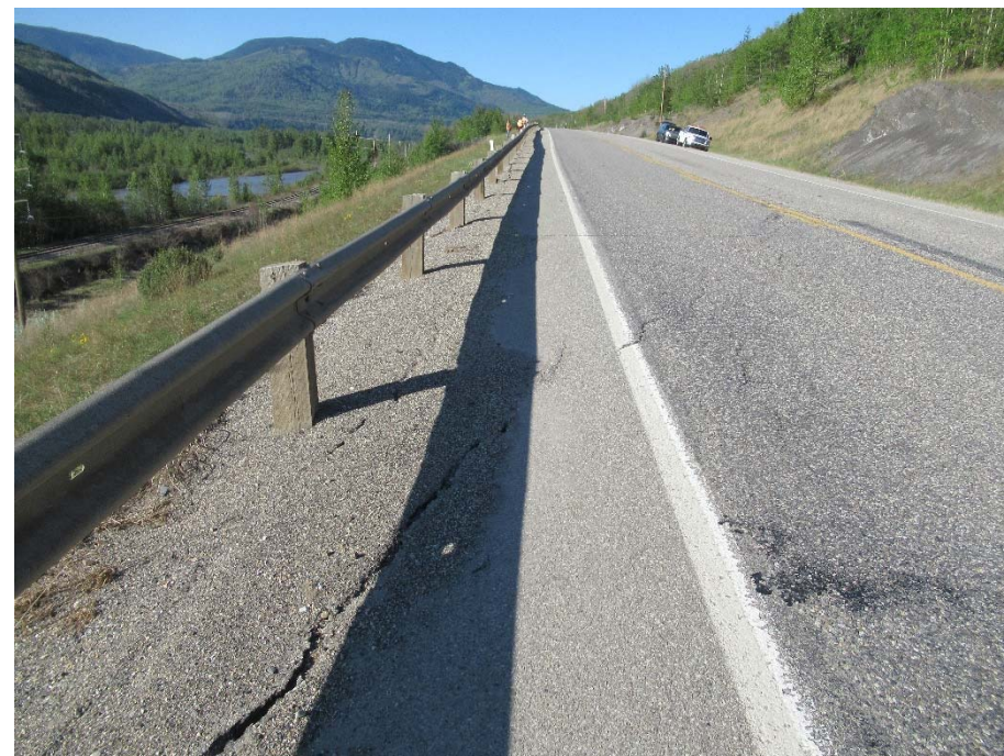
Photo 7. Looking south along the long scarp crack in the highway from near the center of the site.
