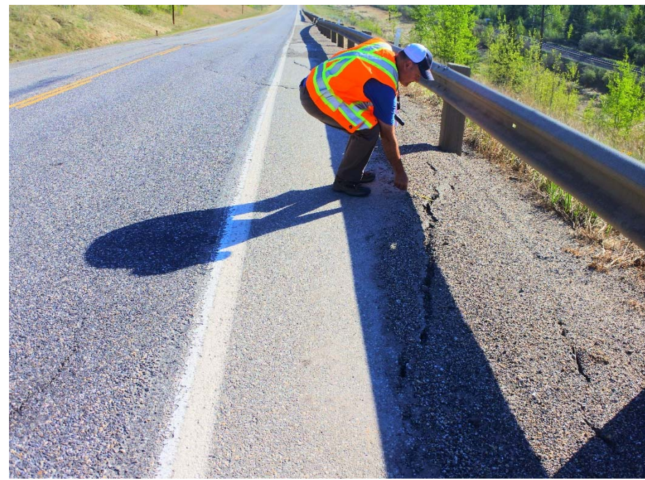
Photo 5. Looking north along the northbound lane shoulder at where northern portion of scarp enters back into shoulder. Larger cracks observed open to 40 mm.
