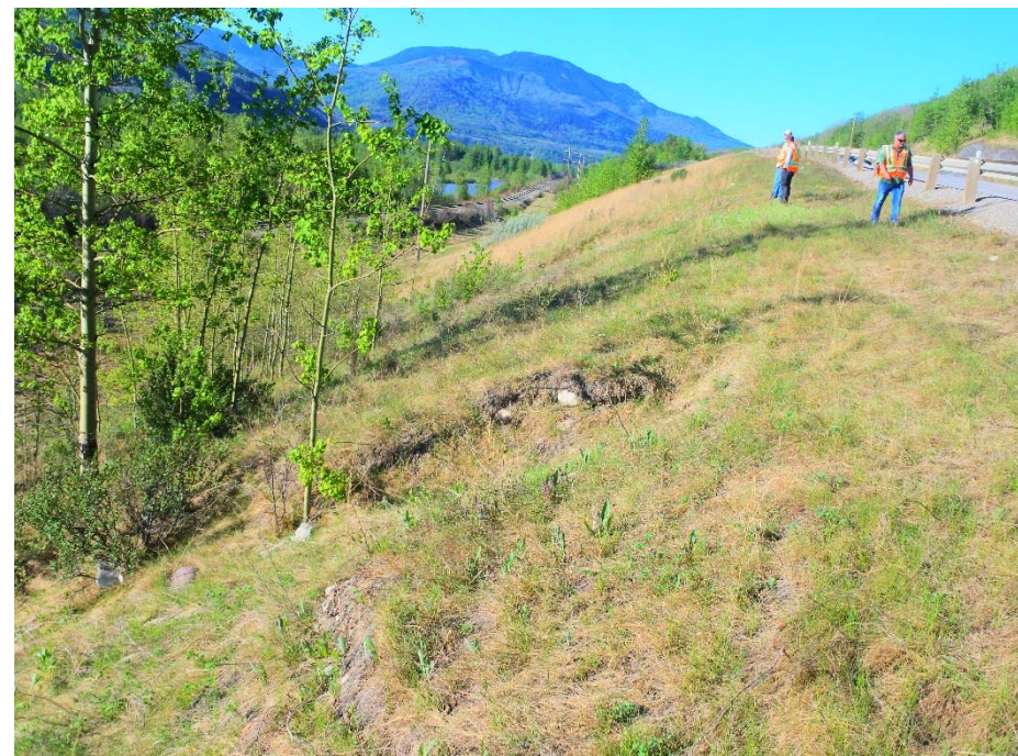
Photo 10. Looking south along the east embankment at teardrop slide failures.
