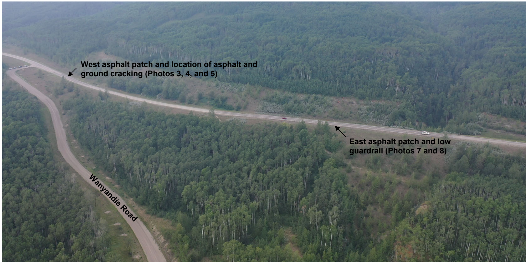
Photo 1 Overview of the GP007 site, highlighting the east and west patches, and areas of asphalt cracking and settlement. Photo taken July 20, 2021 facing northwest.
