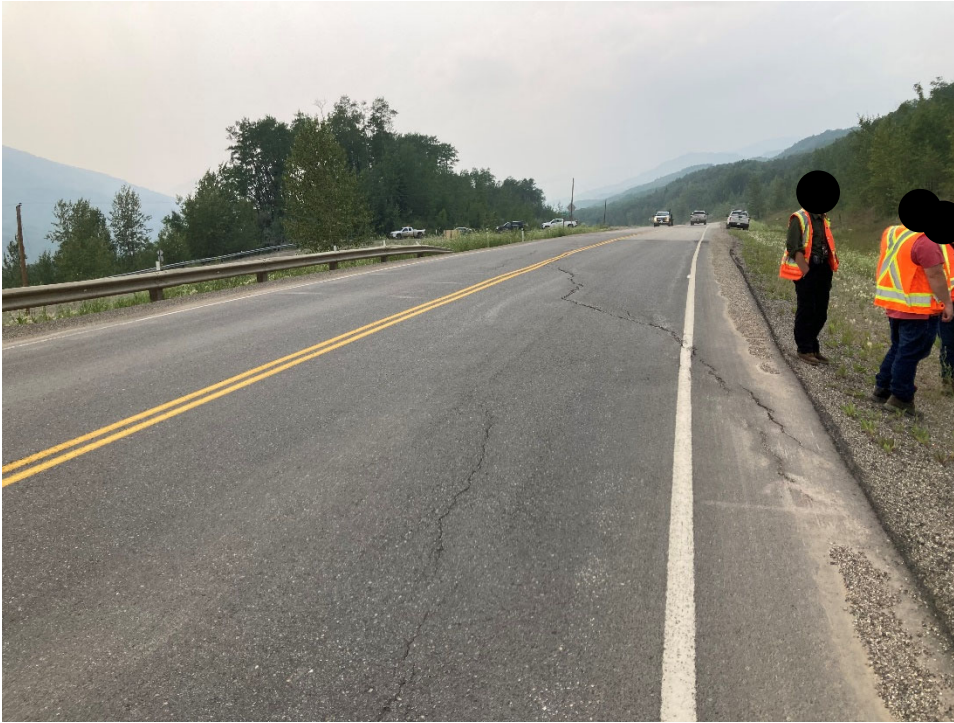
Photo 4 Asphalt cracking at the west flank of the slide in the north (southbound) lane that extends from the edge of the asphalt to the centreline. Photo taken July 20, 2021 facing southwest.
