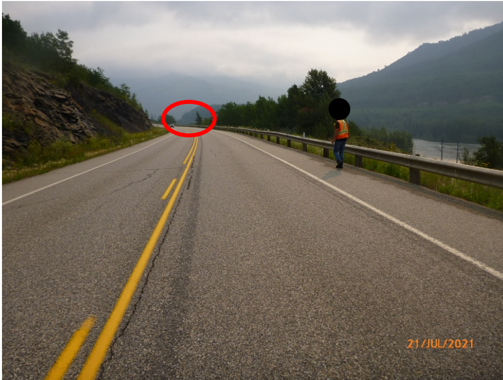
Photo 9 Location of pavement cracking caused by ATCO temporary excavation 50 m to east of North Slide. Photo taken July 21, 2021 facing east. Red circle shows approximate location of pavement cracking in shoulder.
