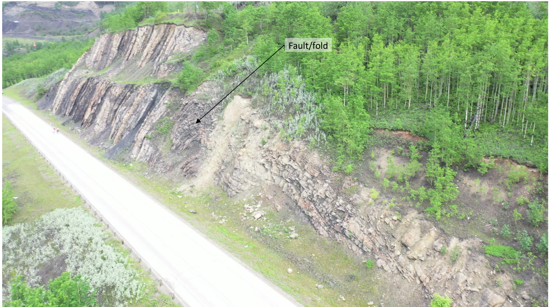
Photo 2 Rock cut slope along west side of Hwy 40:36 between WP190 and WP191 at south/western site limit. Note talus (coal) deposits and rockfall particles in upslope/north highway ditch. As well as change in orientation of bedrock discontinuities mid-photo (near vertical bedding to left/south transitioning at a fault/fold to gently inclined from horizontal on right/north). Photo taken June 14, 2022, with UAV facing northwest.
