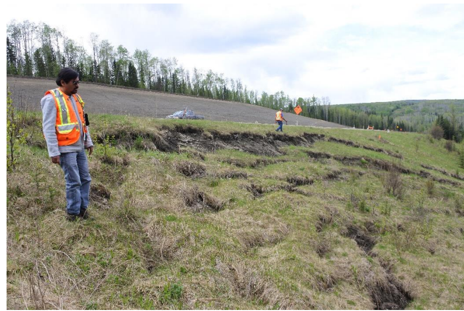
Photo 1. Looking north at active scarp inside slope of southern portion of the site.
