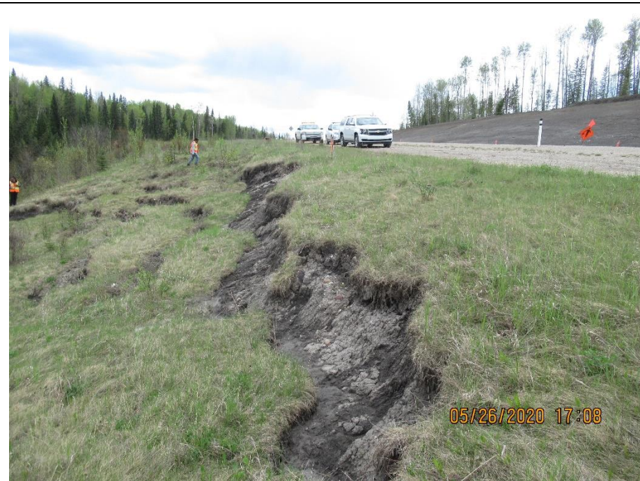
Photo 4. Looking south at long scarp in sideslope at middle of the site.
