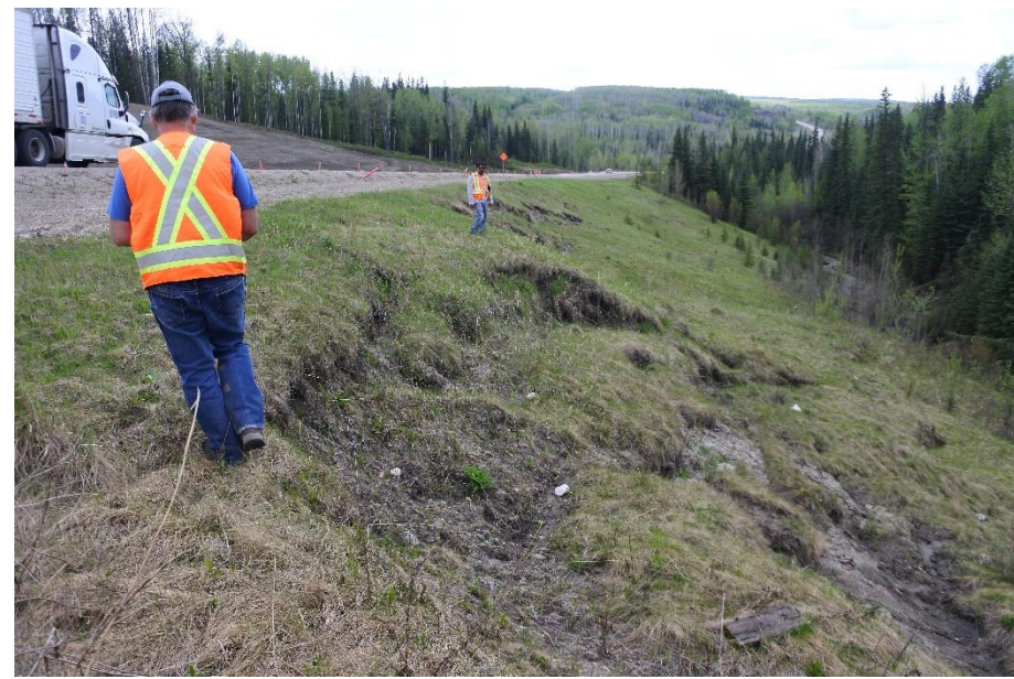
Photo 7. Looking northwest up at the sideslope slumping that extends close to the highway near the north end of the site.
