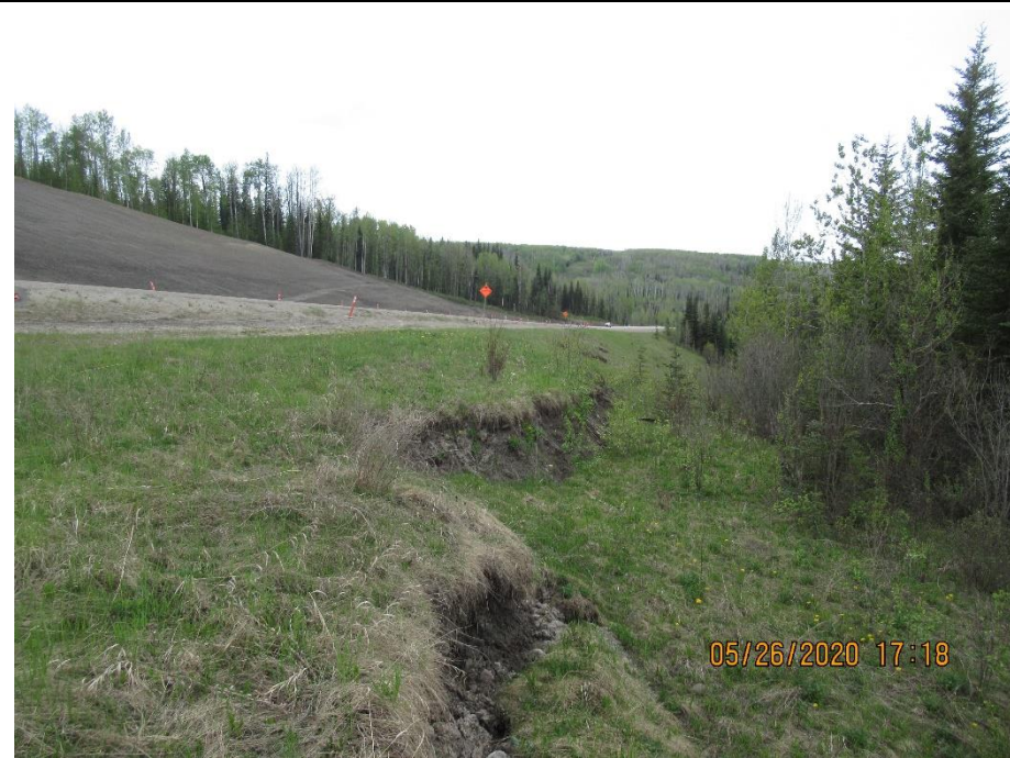
Photo 3. Looking northwest along the top of the embankment fill where fresh slumping has retrogressed close to the highway.
