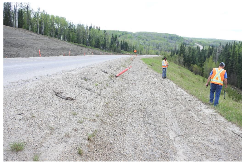
Photo 5. Looking north at where there was previously some erosion rilling observed at the north end of the site but has been filled in.
