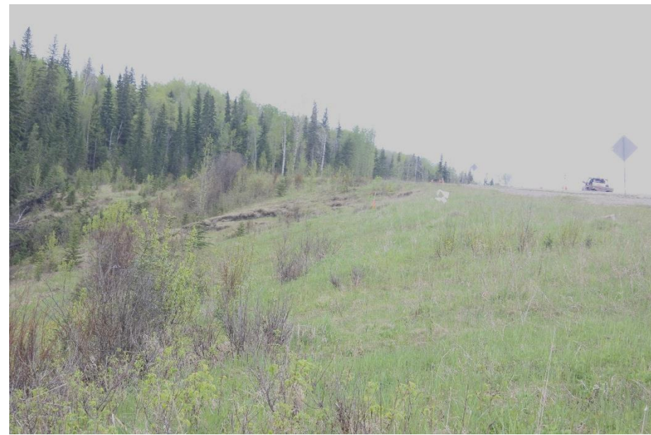
Photo 2. Looking south at active scarp on side slope of southern portion of the site.
