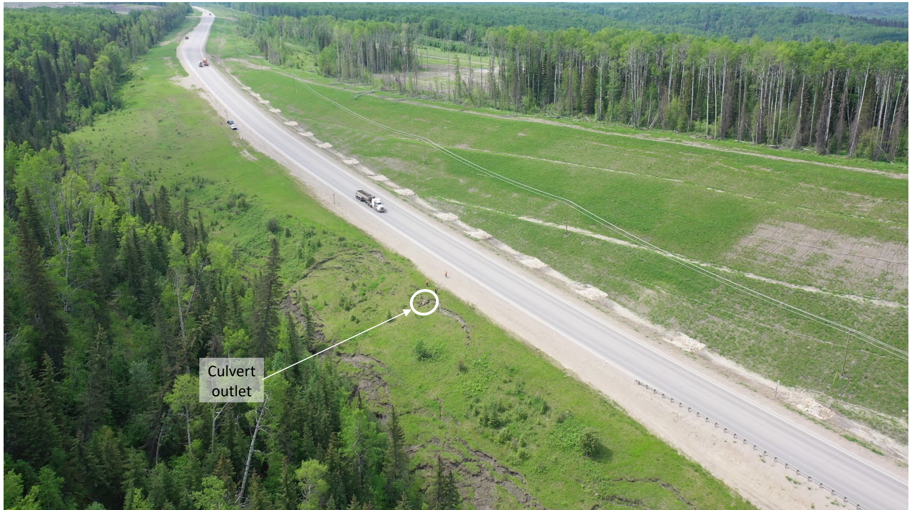
Photo 2 Series of slides between Hwy 40:38 and Roseham Creek. Culvert outlet (circled in white) on downslope/east side of highway at WP218 blocked with soil, inlet not visible in upslope/west highway ditch. Photo taken June 15, 2022, with UAV facing southwest.
