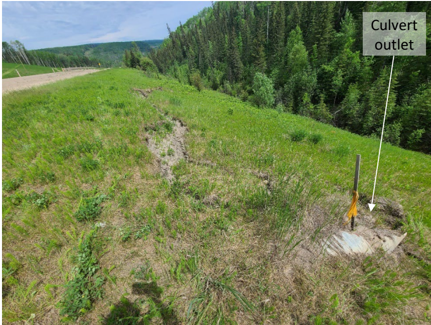
Photo 9 Culvert outlet on east side of Hwy 40:38 at WP218 blocked with soil, inlet not visible in west highway ditch. Some seepage around outlet. Photo taken June 15, 2022, facing north.
