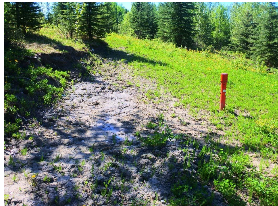
Photo 3. Looking at SI17-6 at the toe of the west embankment where the ground was wet.
