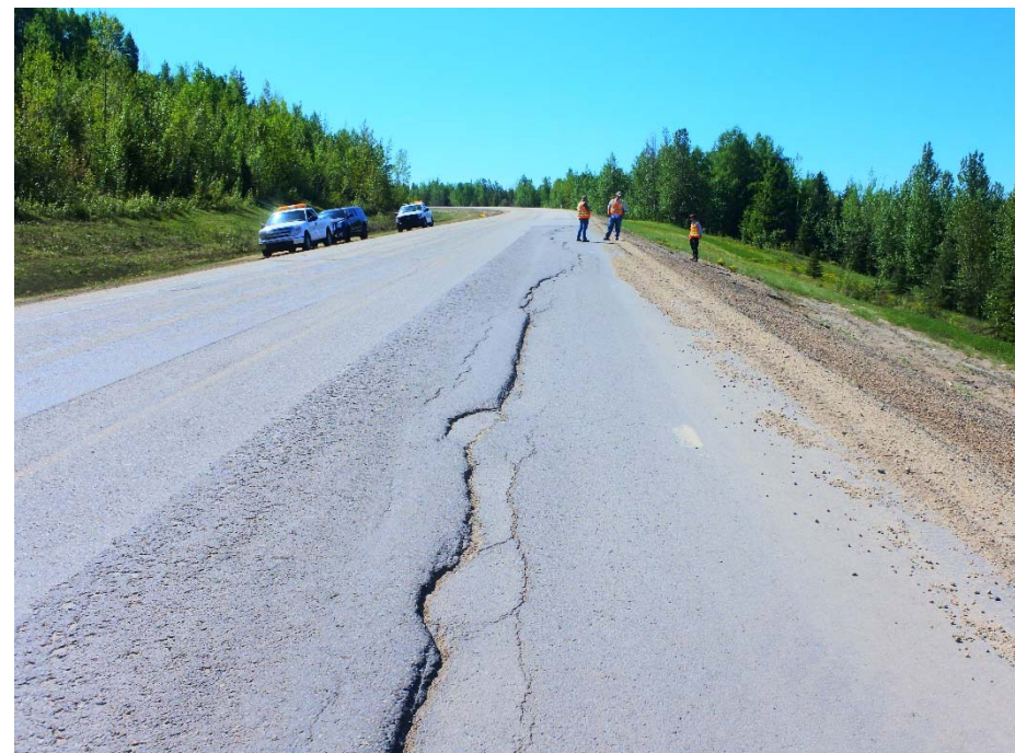
Photo 4. Looking south at scarp crack where the deepest drop exists.
