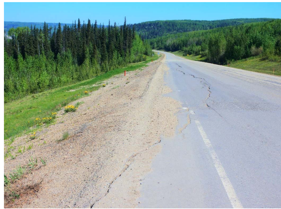
Photo 1. Looking north at the patched southbound lane and reflective scarp crack from the south end of the patch.
