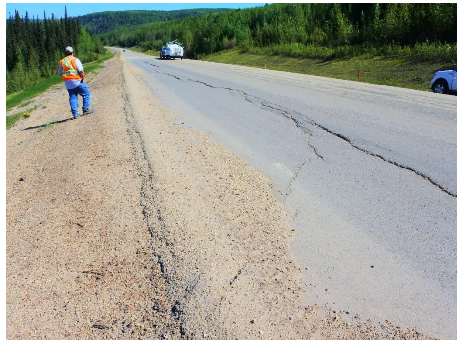
Photo 2. Looking north at scarp crack from the south end of the patch.
