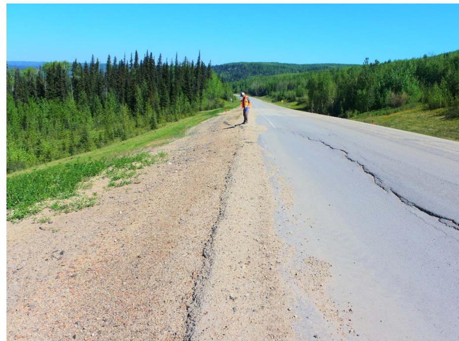
Photo 7. Looking north towards the north end of the scarp crack and patch, with SI17-2 in the background.
