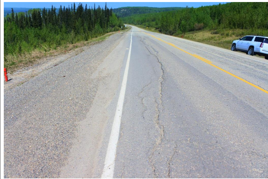
Photo 7. Looking north towards the north end of the scarp crack and patch, with SI17-5 on the left
