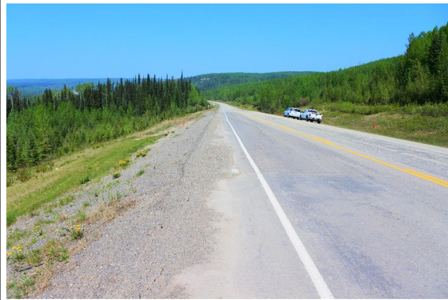
Photo 1. Looking north at the patched southbound lane and reflective scarp crack from the south end of the patch.
