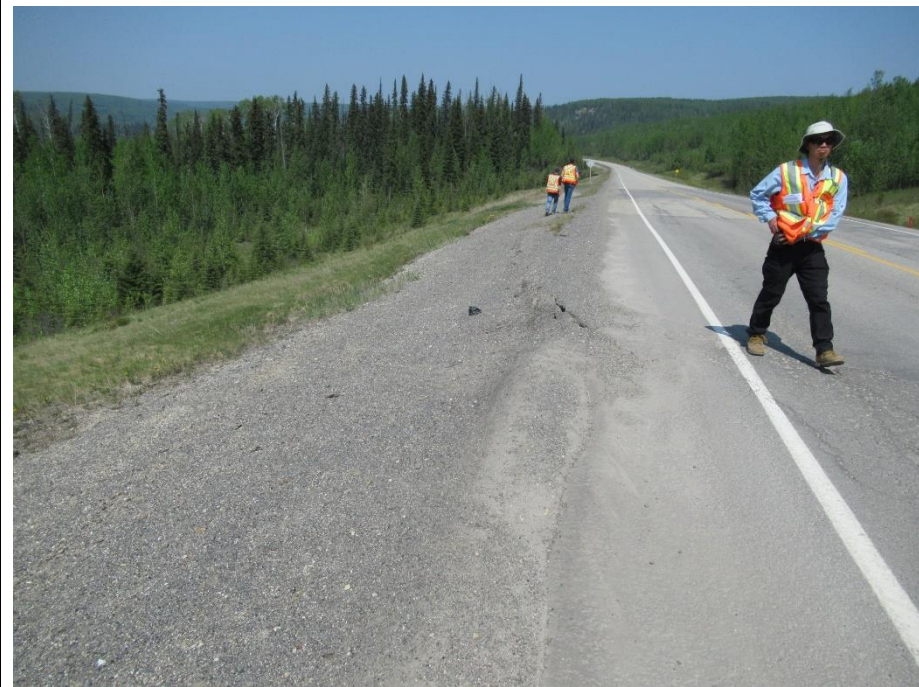
Photo 6. Looking north at where the scarp crack extends off of the shoulder and into the embankment.
