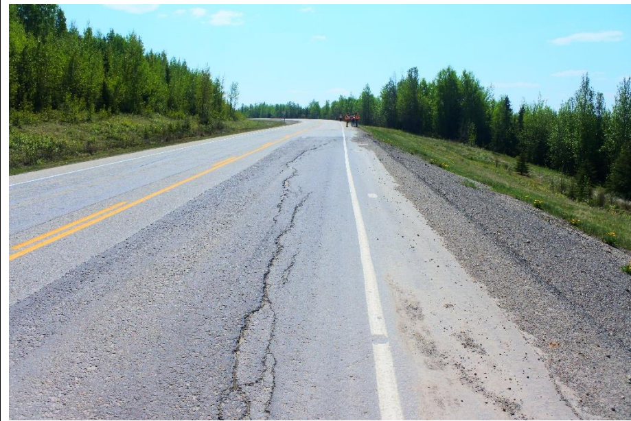
Photo 4. Looking south at scarp crack where the deepest drop exists.
