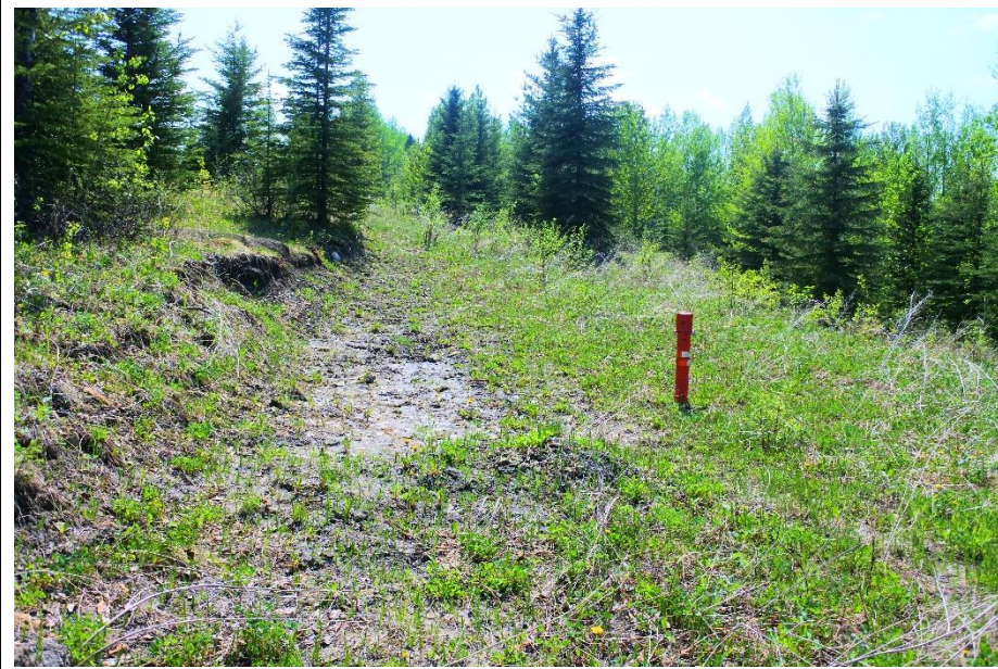
Photo 3. Looking at SI17-6 at the toe of the west embankment where the ground was wet.
