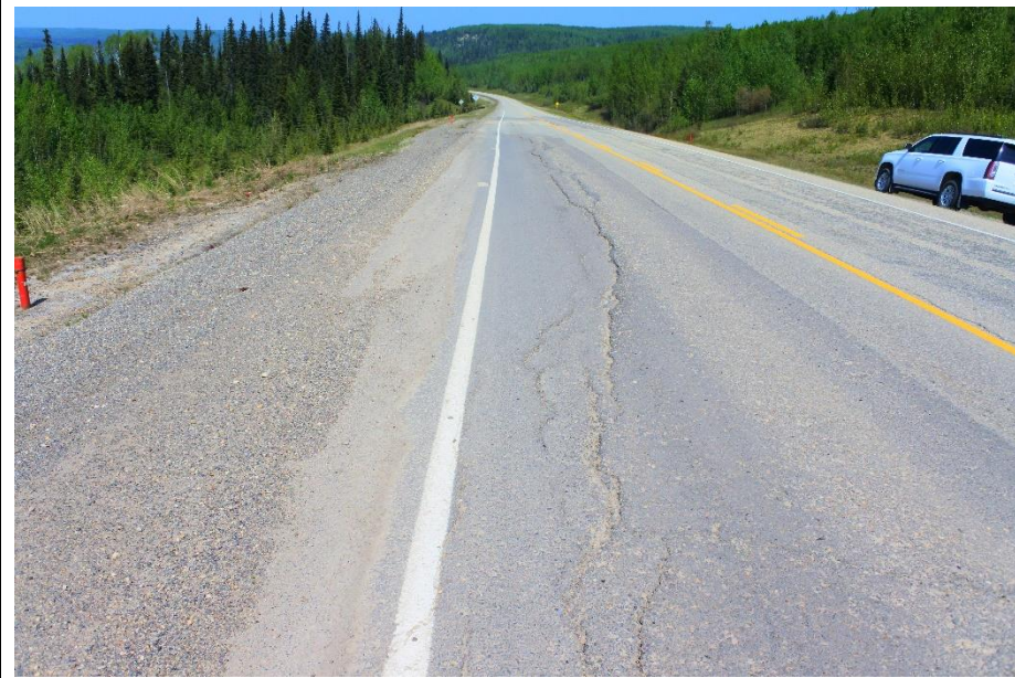
Photo 2. Looking north at scarp crack from the south end of the patch.
