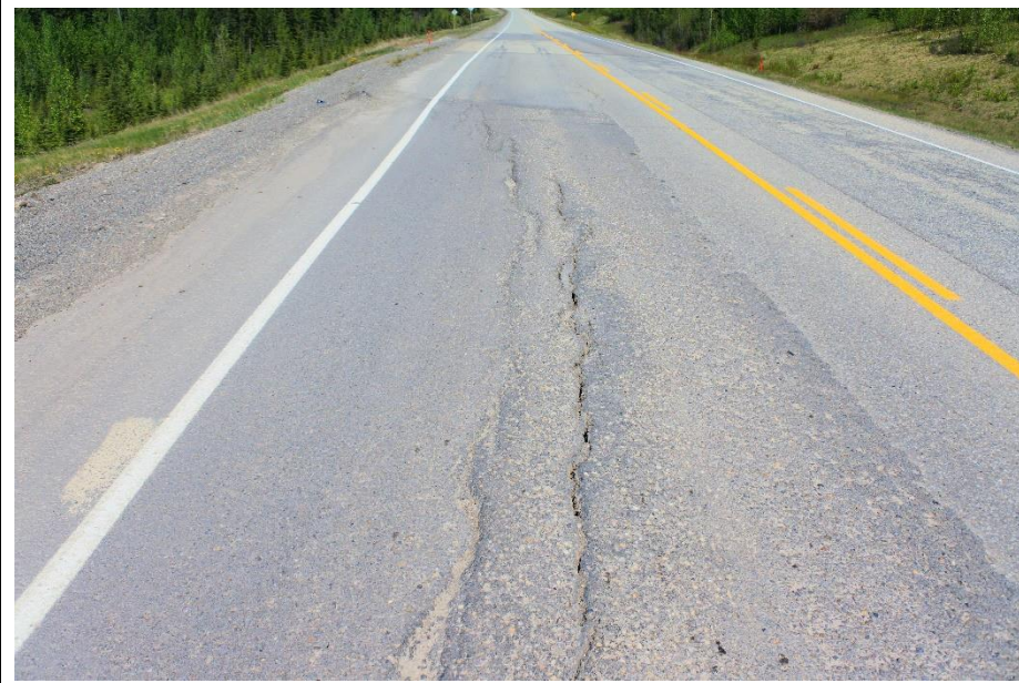
Photo 5. Looking north at the north end of the scarp crack.
