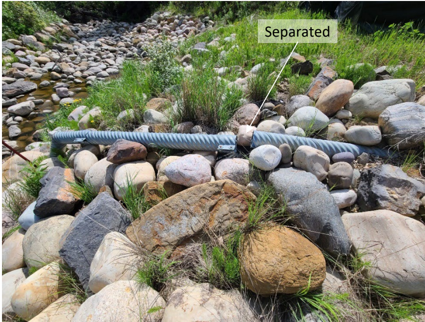
Photo 13 Subdrain outlet at GP038-II separated and not flowing. Photo taken June 15, 2022, facing east.
