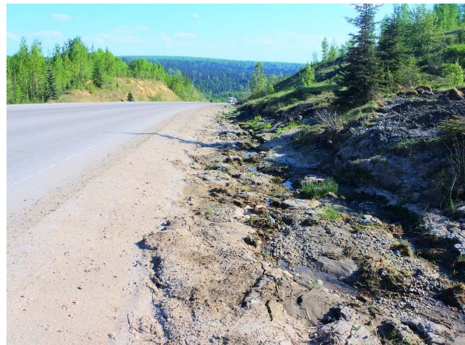
Photo 1. Looking south along at seepage into the west ditch at the north end of the site.
