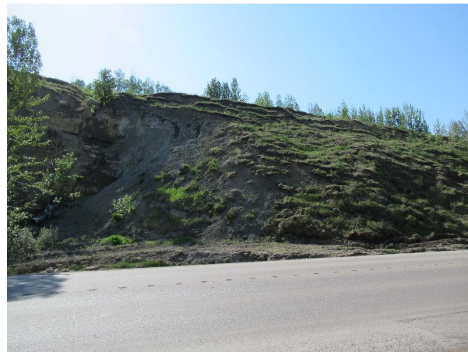
Photo 6. Looking west at erosion caused by a broken 600 mm CSP exposed in the slumping backslope.
