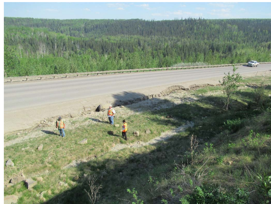
Photo 12. Looking southeast down at erosion gully that runs along the west ditch/shoulder.
