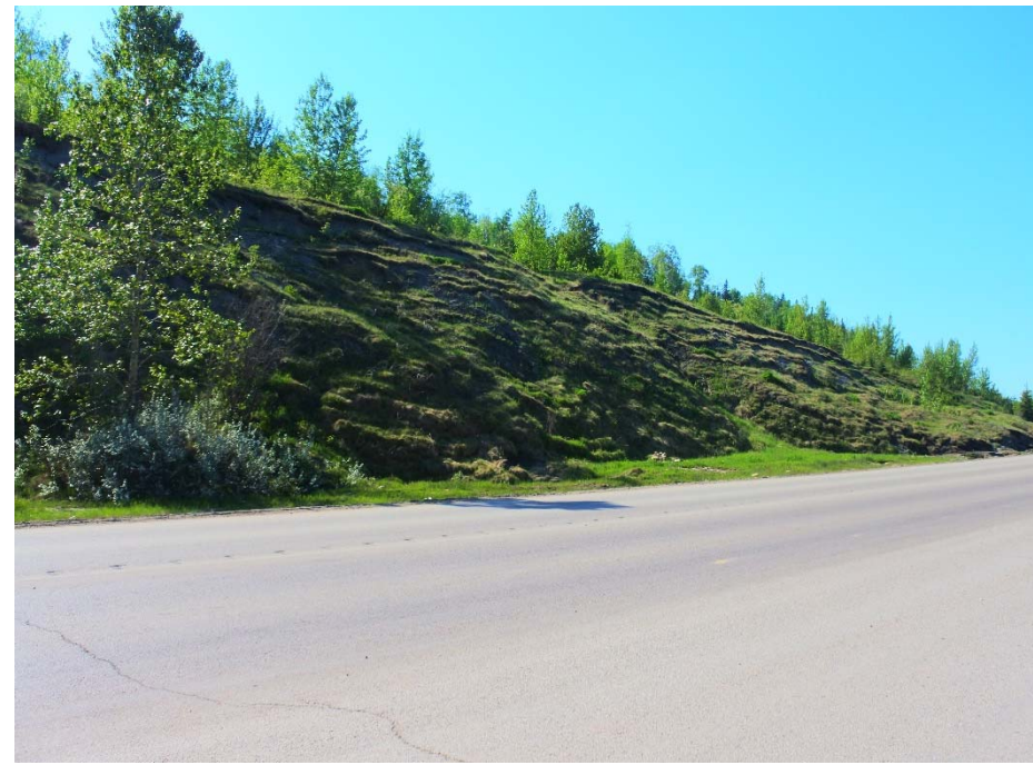
Photo 4. Looking north at the toe slumping into the west ditch.
