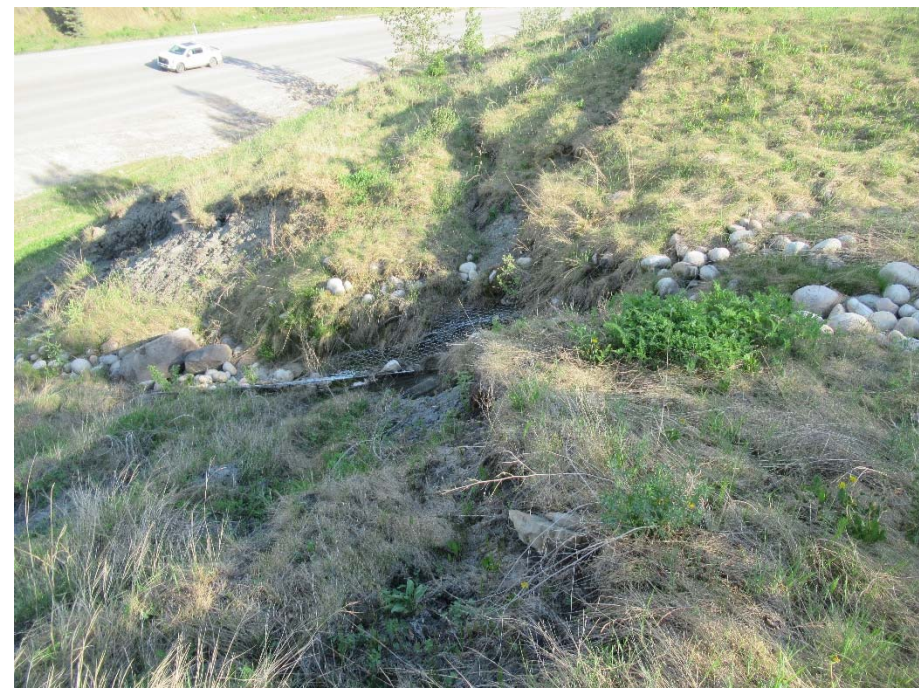
Photo 3. Looking south at the deteriorated gabion armour.
