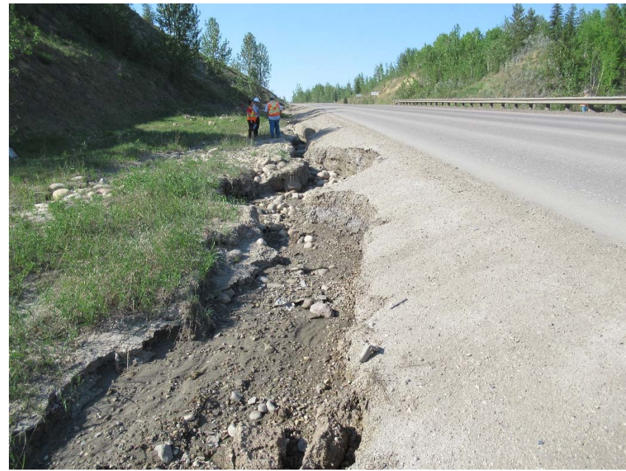
Photo 10. Looking north at the west ditch erosion gully which has formed around the toe of slide encroaching against the highway embankment near middle of site.
