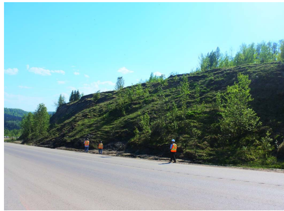
Photo 5. Looking north at the north end of the scarp crack.
