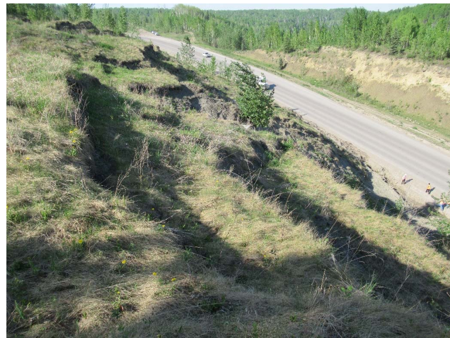
Photo 14. Looking north at sloughed material just north of photo 13.
