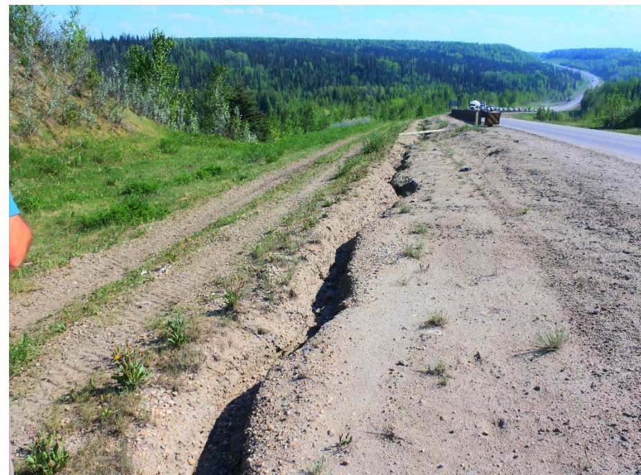
Photo 7. Looking south at new erosion observed on the east side of the highway.
