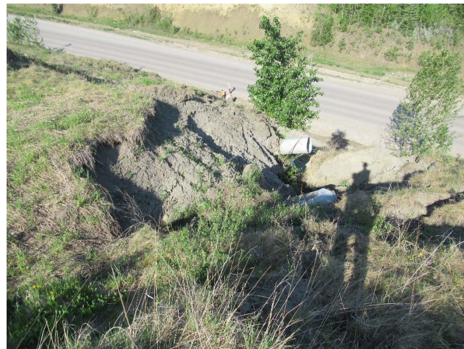
Photo 11. Looking down towards road from the slope crest at the eroded gully caused by the broken 600 CSP.
