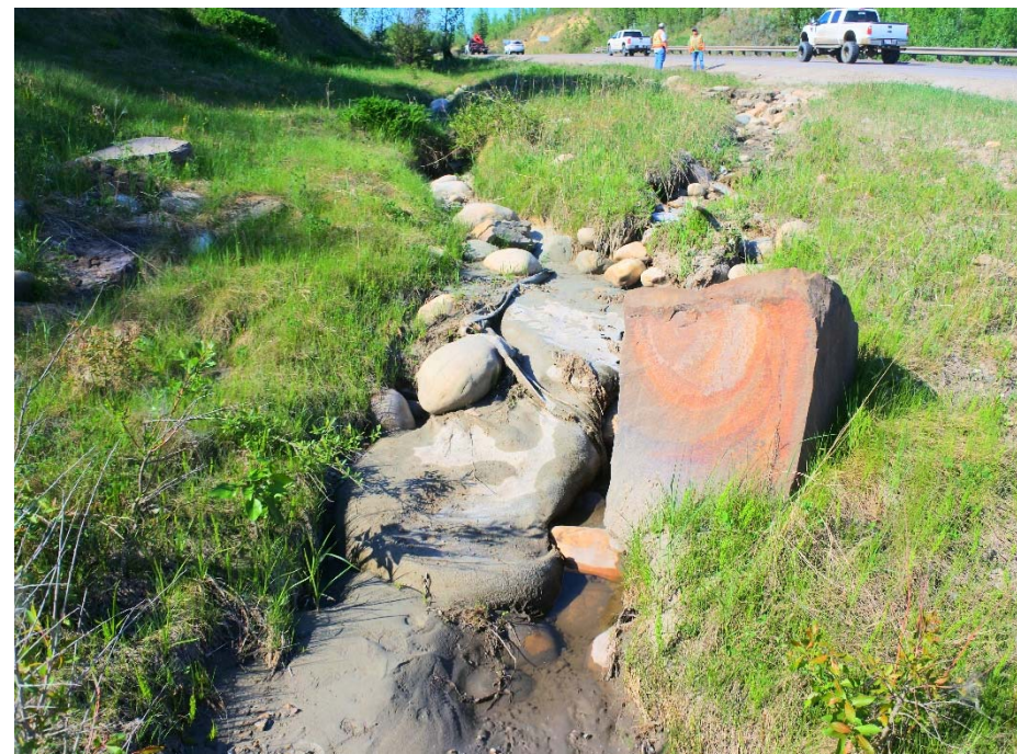
Photo 8. Looking north at large fallen boulder in erosion gully.
