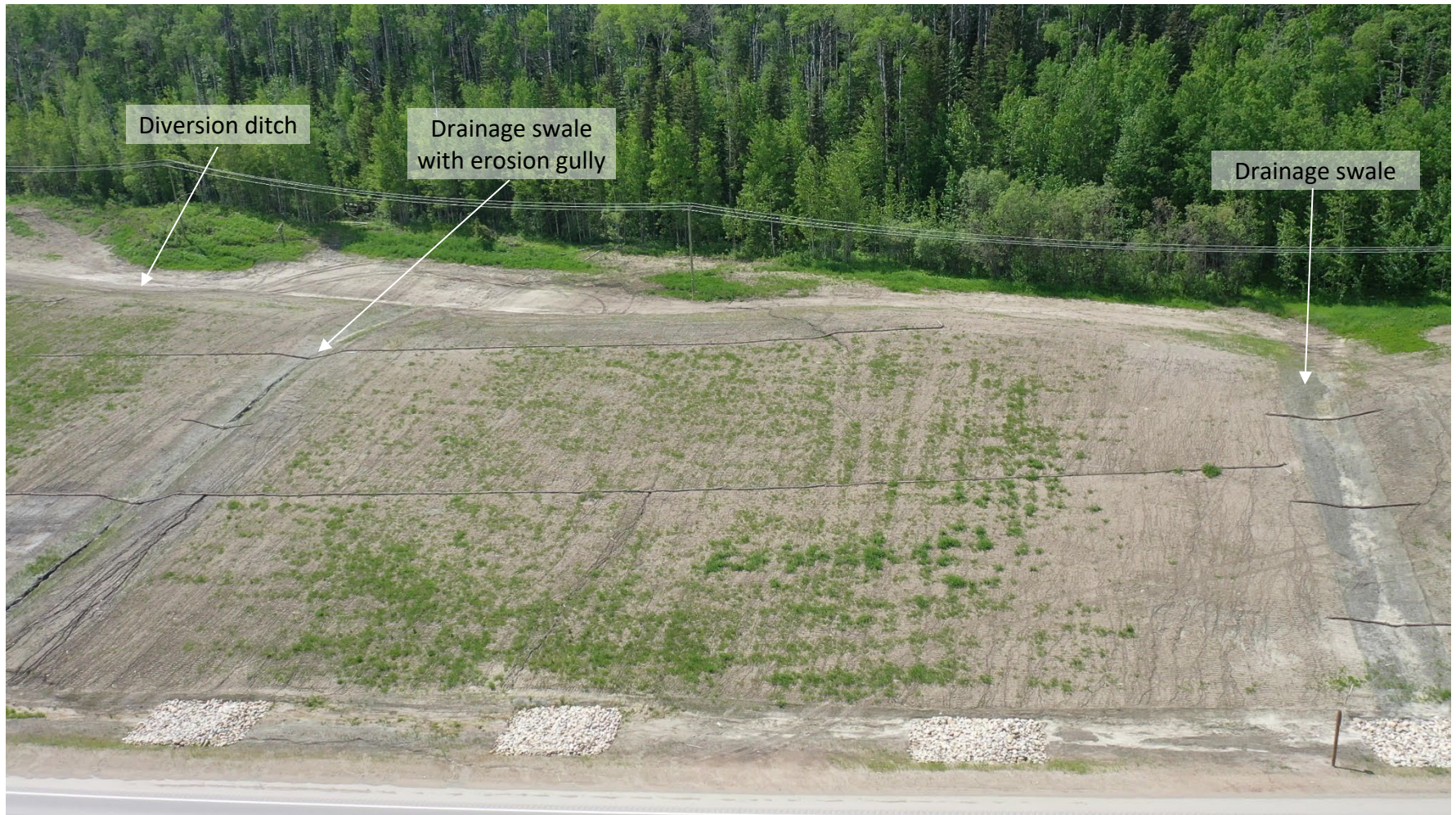
Photo 3 Backslope along west side of Hwy 40:40. Note rill and small gully erosion on backslope, and small gully eroded down south drainage swale. Photo taken June 15, 2022, facing north.
