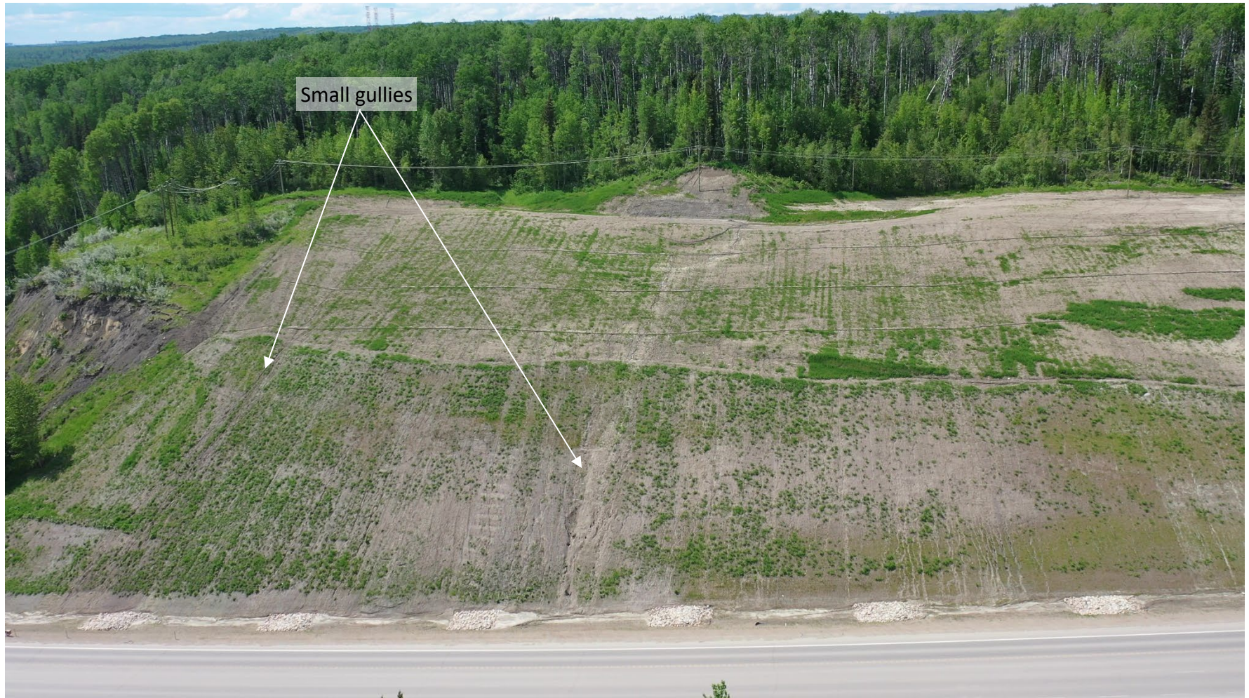
Photo 5 Backslope along west side of Hwy 40:40. Note rill and small gully erosion on backslope. Photo taken June 15, 2022, facing north.
