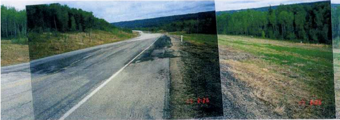
Looking towards Grande Prairie, headscarp crack and settlement transgressed past centreline to backslope ditch.
