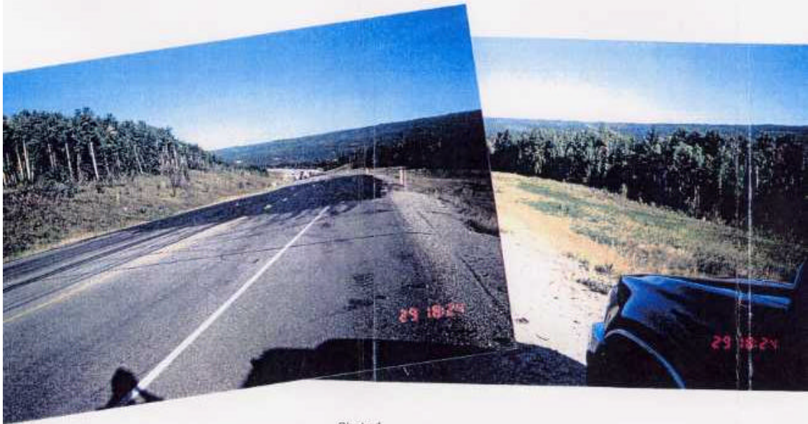
Photo 1 Slide head scarp (pavement cracking) across centerline (looking north towards Grande Prairie). Photo taken August 30, 1998.
