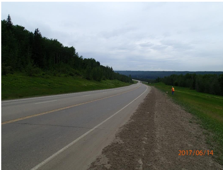
Photo 8. Looking northwest at km 25.75 along the NBL shoulder at cracks in the roadway shoulder.
