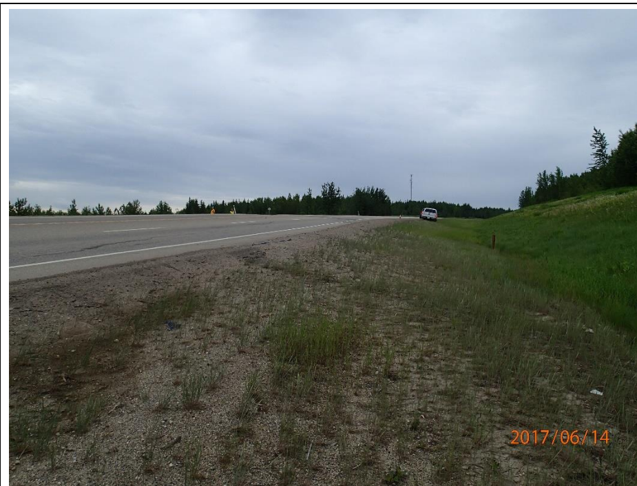
Photo 9. Looking southeast at km 25.8 along the SBL shoulder at longitudinal cracks in the SBL ACP.
