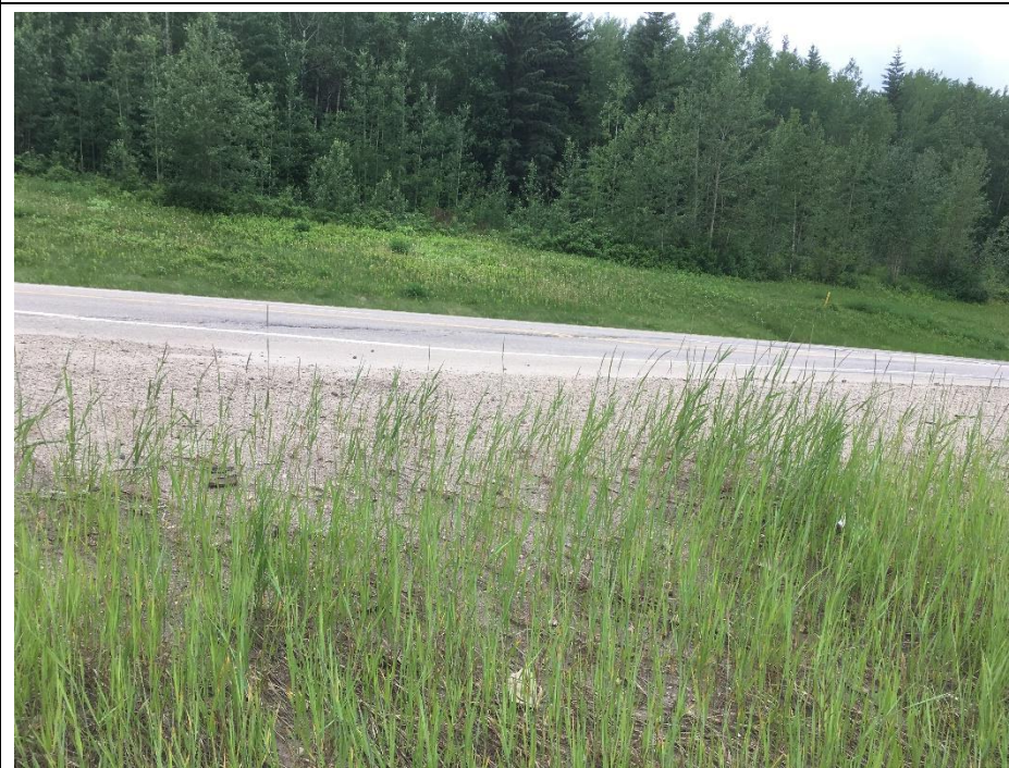
Photo 4. Looking west towards dip in the roadway at km 25.51.
