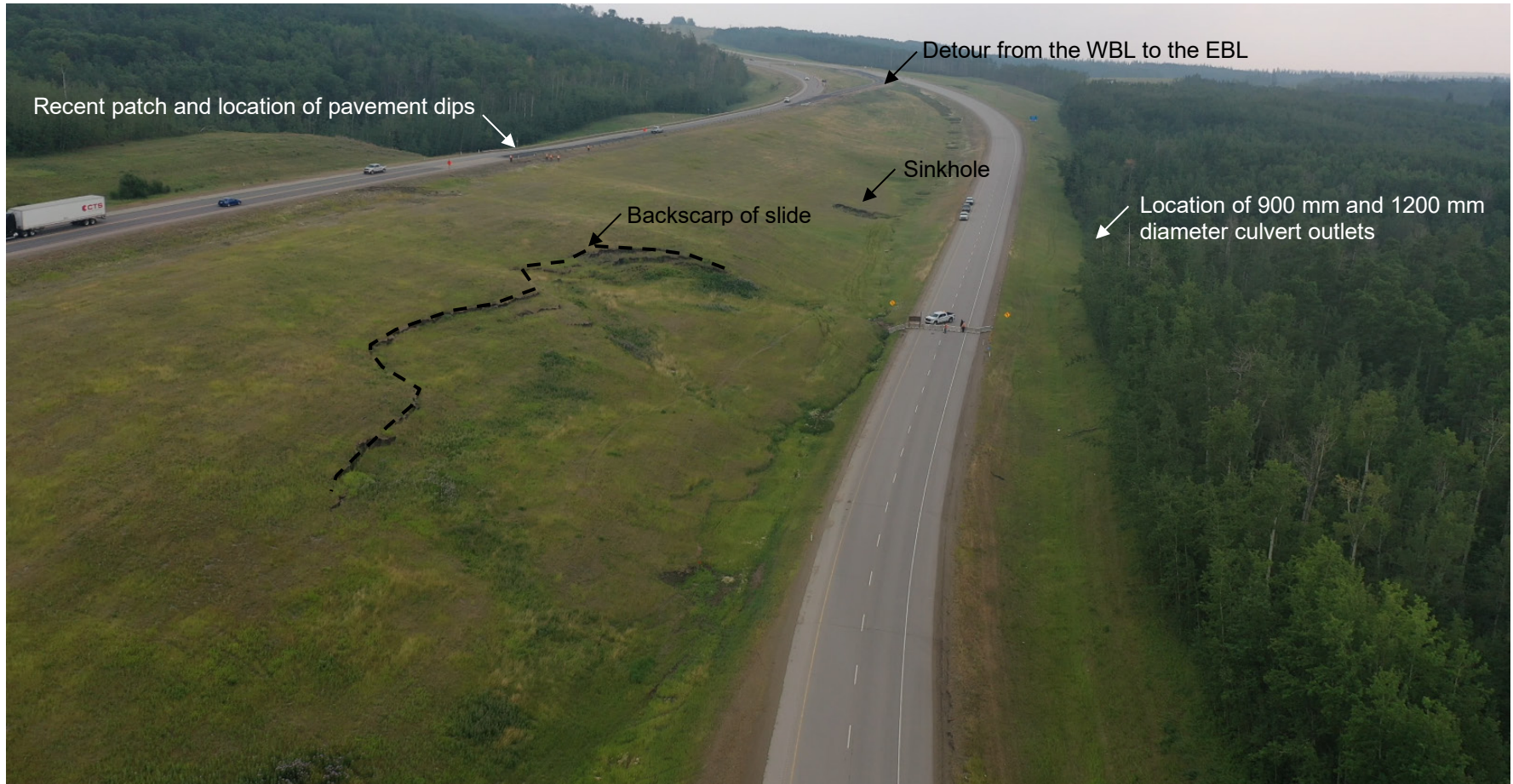
Photo 1 Overview of the GP045 site, highlighting the slide, sinkhole, culvert outlet location, and recent asphalt patching. Photo taken July 19, 2021 facing east.
