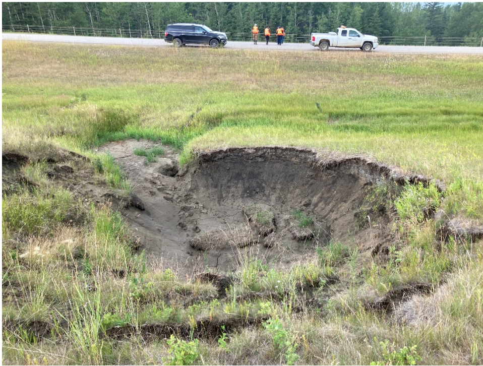
Photo 2 Sinkhole located on the north side of the EBL lanes of Hwy 43. Photo taken July 19, 2021 facing south.
