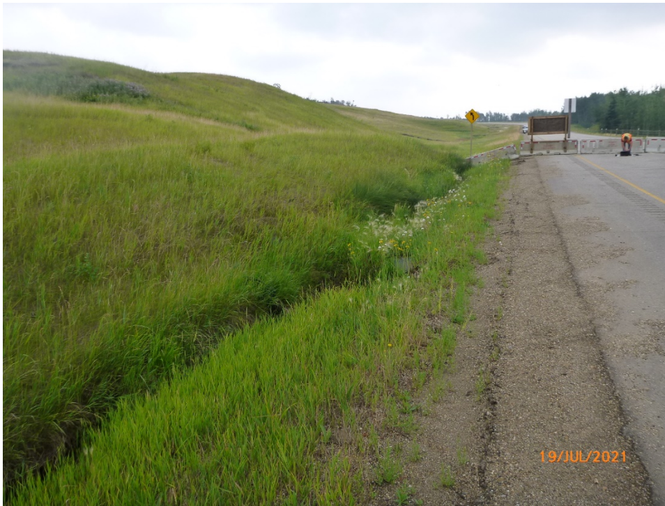
Photo 4 Toe bulge in the north (eastbound) ditch of Hwy 43. Photo taken July 19, 2021 facing east.
