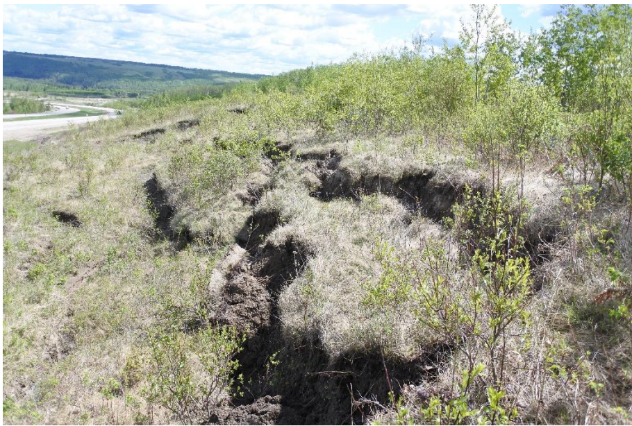
Photo 10. Looking east along the backscarp of Slide 3 from near the center of the slide. The height of the drop along the backscarp varies from 1.5 m to 3.0 m in the eastern half of the slide.
