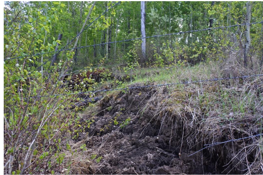
Photo 14. Looking southeast at Slide 4 backscarp extending beyond the fence 6-7 m.
