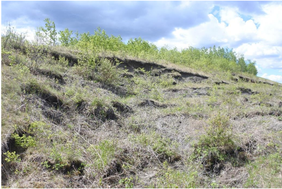
Photo 9. Looking south at the backscarp of Slide 3 from near the middle of the slide. Slide 3 is about 100 m in width and extends about 35 m down the slope. The height of the drop along the backscarp is of about 1.5 m here.
