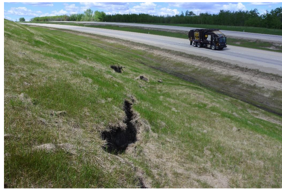
Photo 5. Looking north at small erosion gully that is forming from surface flow above Slide 1.
