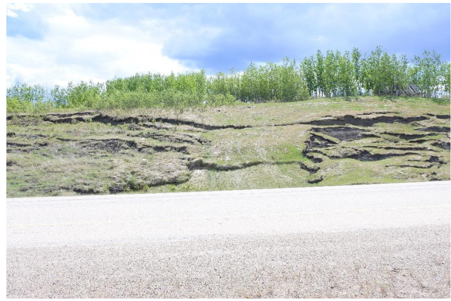
Photo 16. Looking south where Slide 2 now connects to Slide 3.
