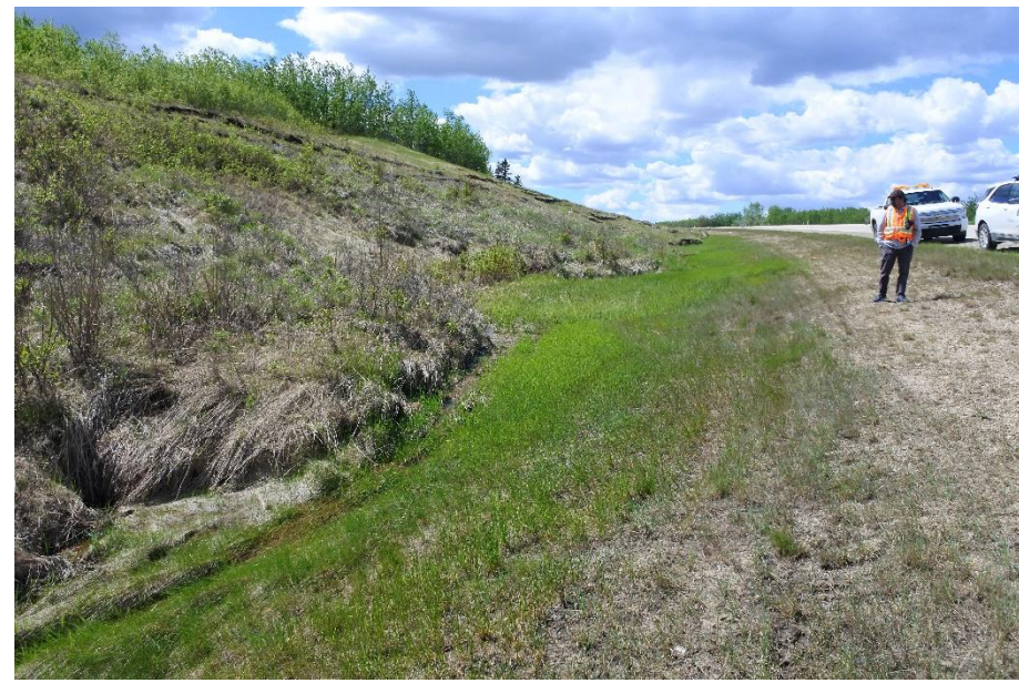
Photo 6. Looking southwest from the EBL of Hwy north shoulder 43:04 at Slide 2.
