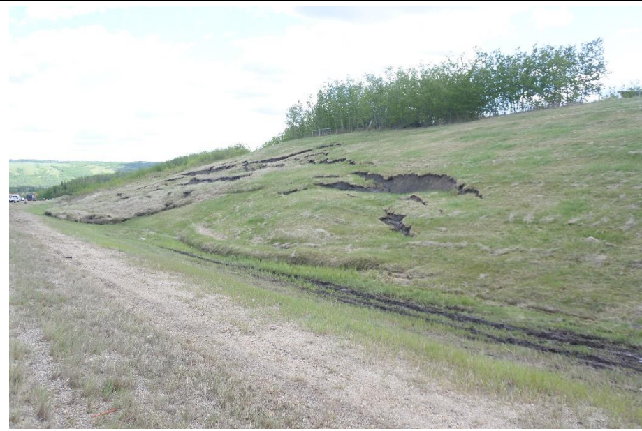
Photo 2. Looking southeast from the edge of the EBL shoulder towards Slide 1 and 2 which are now one slide. The backscarp has a 2.1 m drop, is about 125 m in width and extends about 32 m down the slope.
