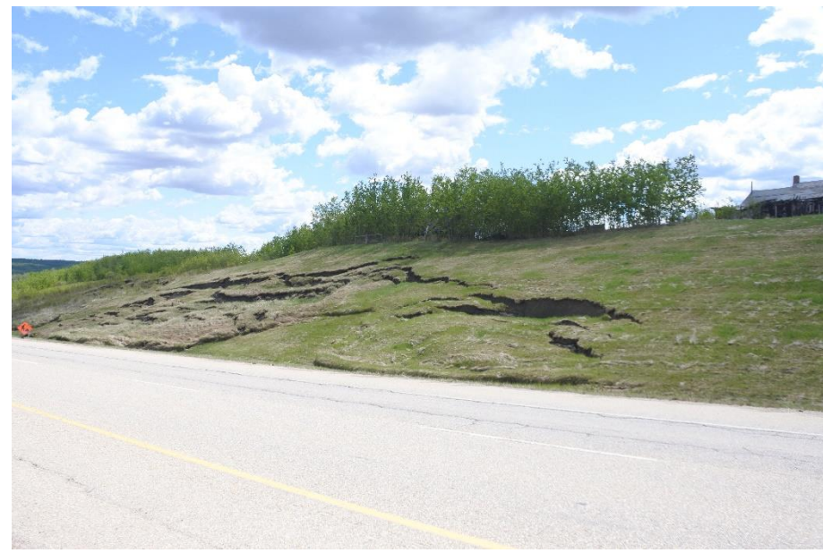
Photo 1. Looking southeast from the median of Hwy 43:04 towards the slides in the backslope above the EBL. The slides are identified from right to left as Slides 1 to 2 which have now become one slide.
