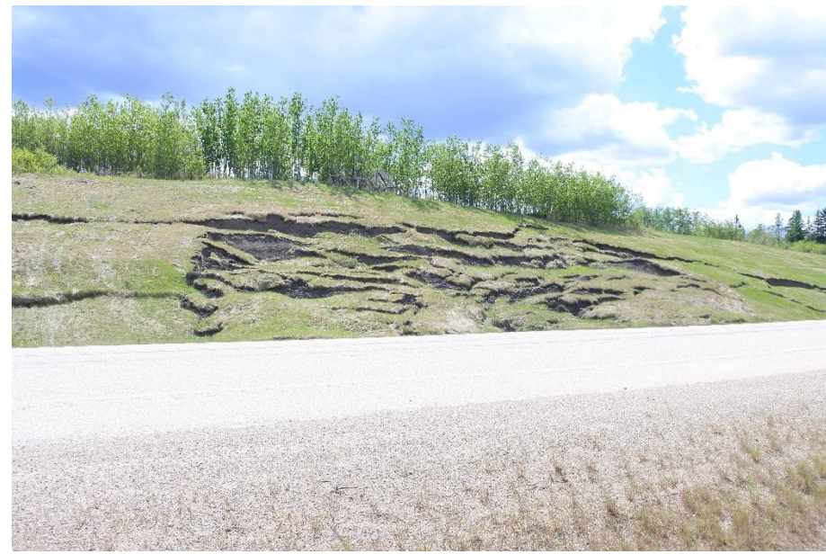
Photo 4. Looking south from the middle of Slide 1 & 2 at the scarp cracks. The ditch flow of the EBL is impeded by the accumulation of slide debris at the toe.
