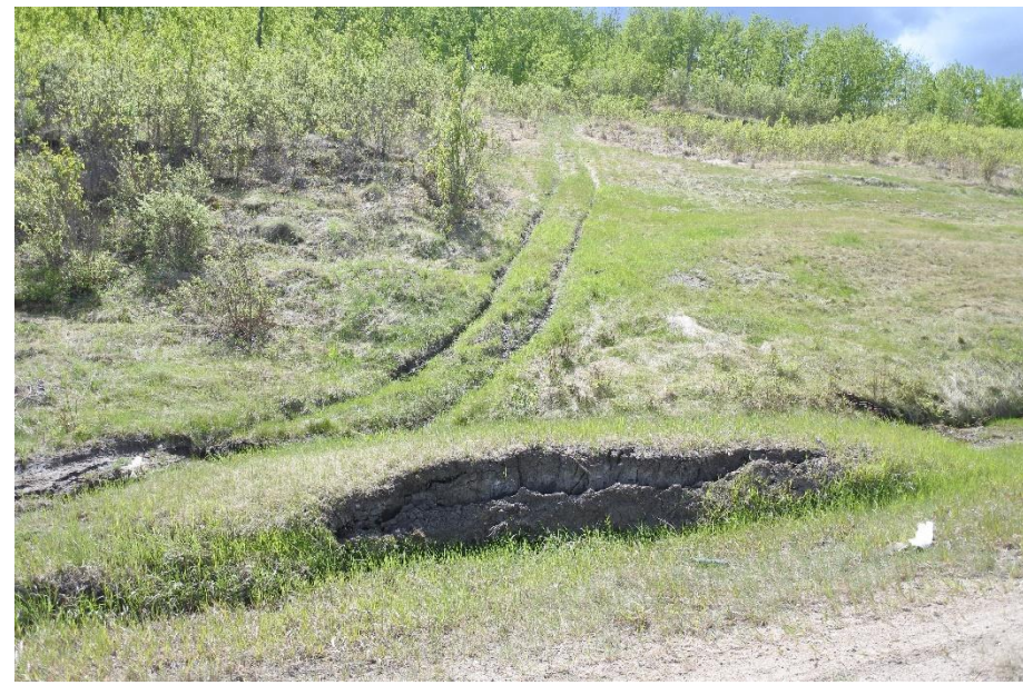
Photo 12. Looking south from the EBL ditch of Hwy 43:04 at Slide 4. Slide 4 is now about 115 m in width and extends 32 m from the crest of the slope to the level of the ditch south side bottom of the EBL. Slide 4 is now more active than the other 3 slides with a bulge and erosion at the toe.
