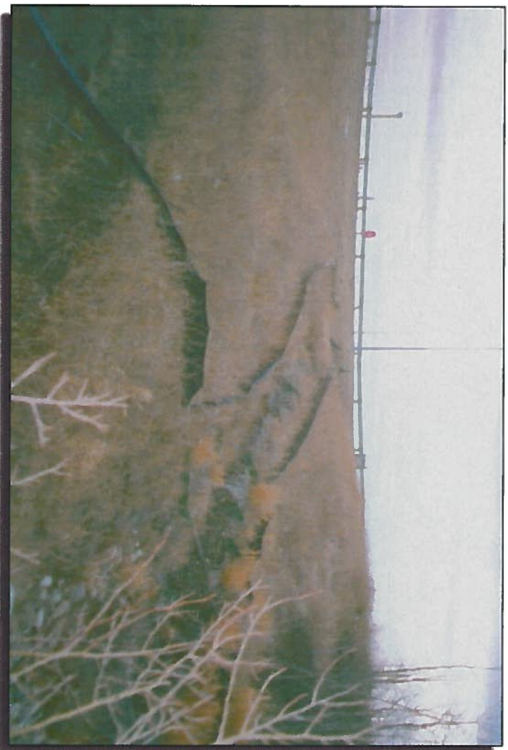
Photo 7 Looking south up headslope at west ditch. -Outfall and erosion of ditch down headslope.
