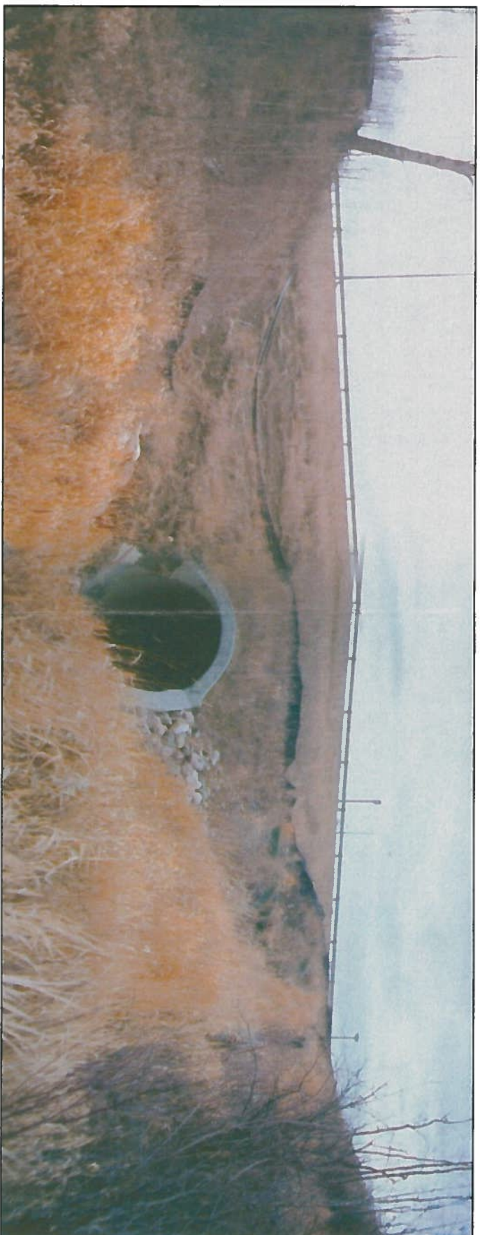
Photo 6 Looking south at inlet and headslope. -East ditch outfall (on left) with headslope sloughing. -West ditch outfall (on right).
