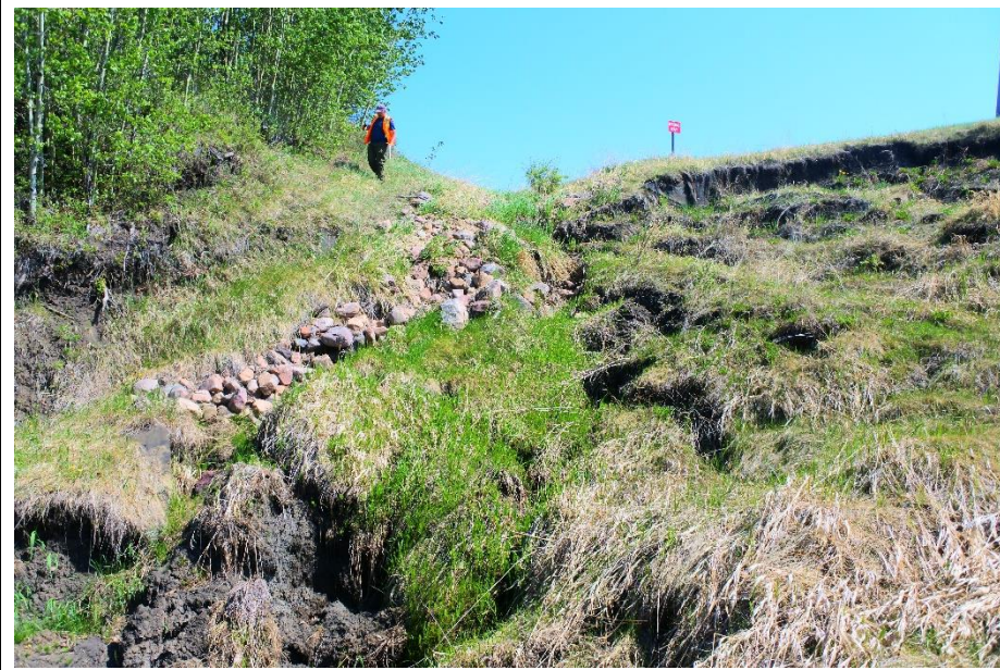
Photo 9. Looking east at slide scarp and at disturbed swale and riprap.
