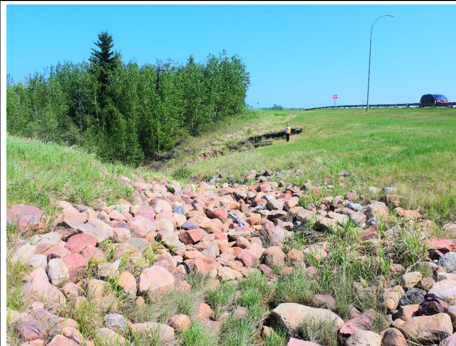
Photo 1. Looking east from 800 mm CSP culvert towards slide.
