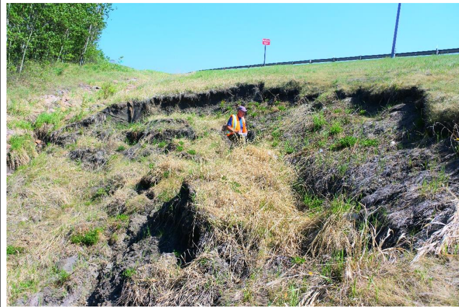
Photo 8. Looking southeast at slide scarp.
