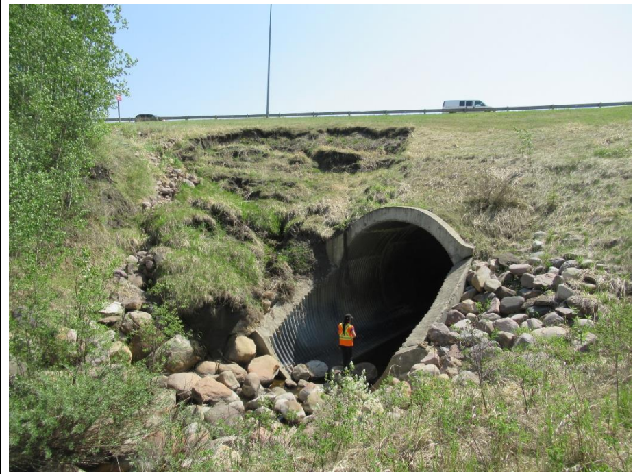
Photo 6. Looking south towards culvert inlet and slide on the left side of it.
