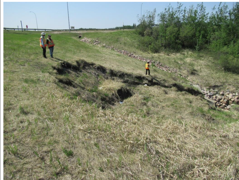
Photo 3. Looking west at slide backscarp.
