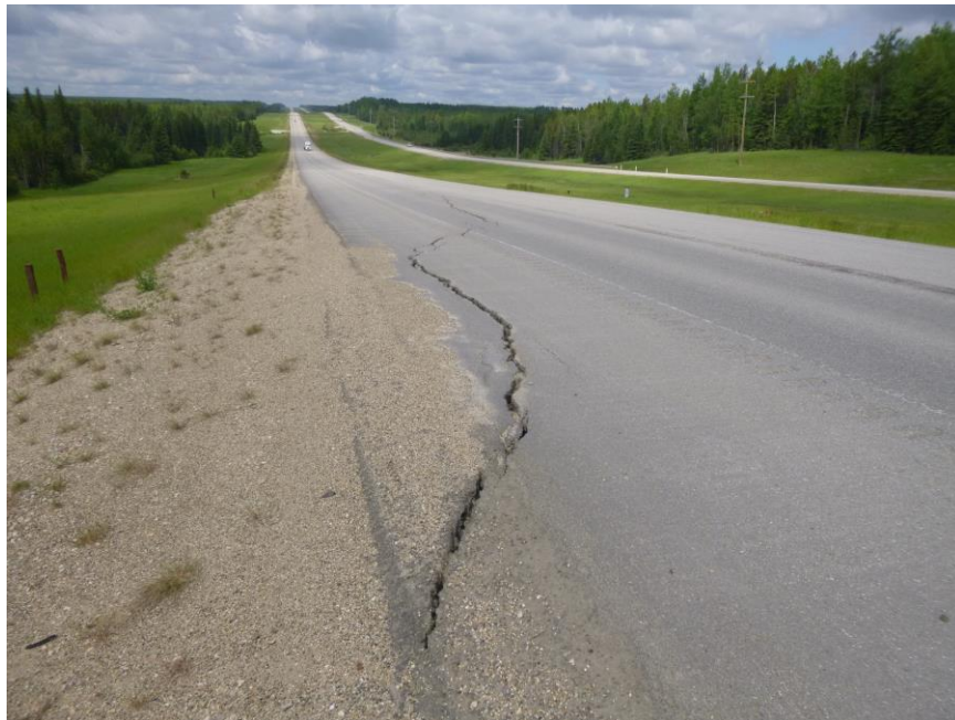
Photo 8 - Looking west along the open slide crack in the highway eastbound lanes. Note the slight dip in the highway south of this crack.
