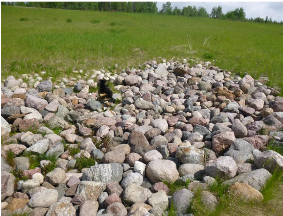
Photo 14 - Looking north at the subdrain outlet and riprapped drainage channel south of the highway.
