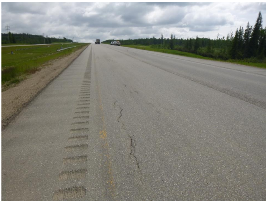
Photo 10 – Looking east at the crack along the outside edge of the EB driving lane.
