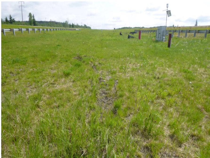
Photo 6 – Looking east along the median at a minor erosion gully. Note the silt fence still remaining east of the central monitoring station.
