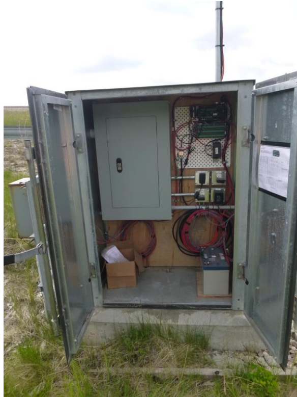
Photo 7 – Looking south at the inside of the CMS (control panel door closed).
