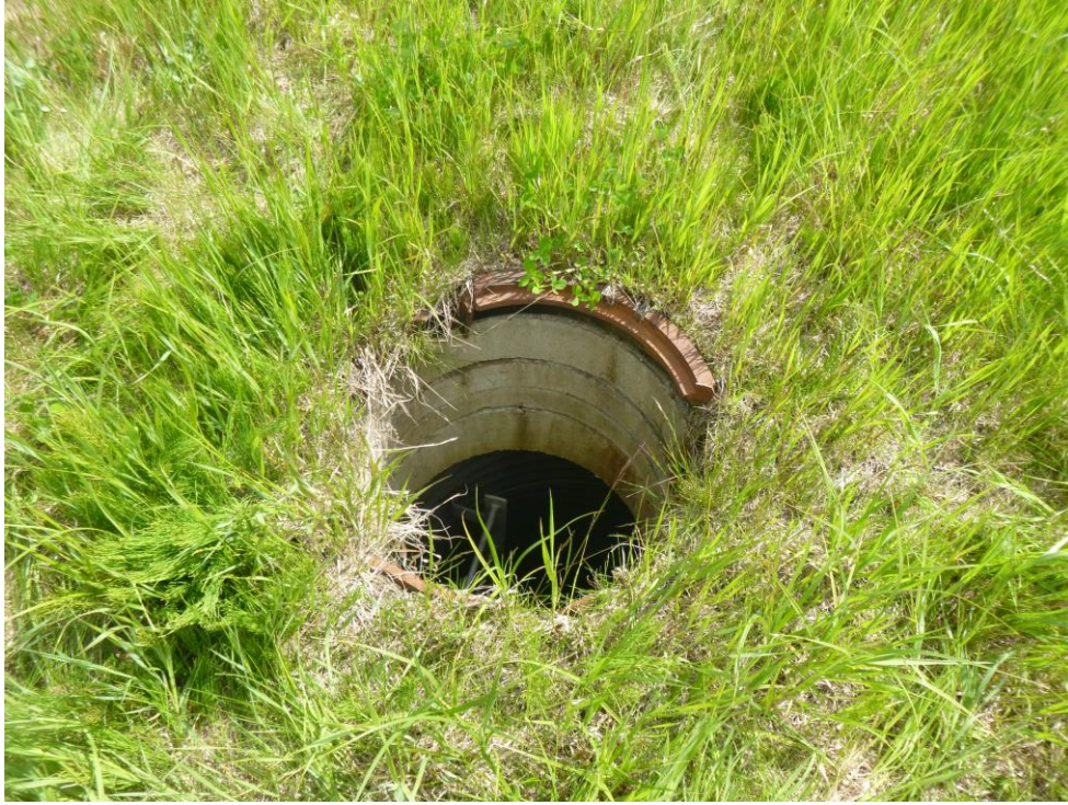
Photo 3 – Looking at a missing lid overtop of the manhole west of the instrumentation that directs water southwards beneath the hwy.
