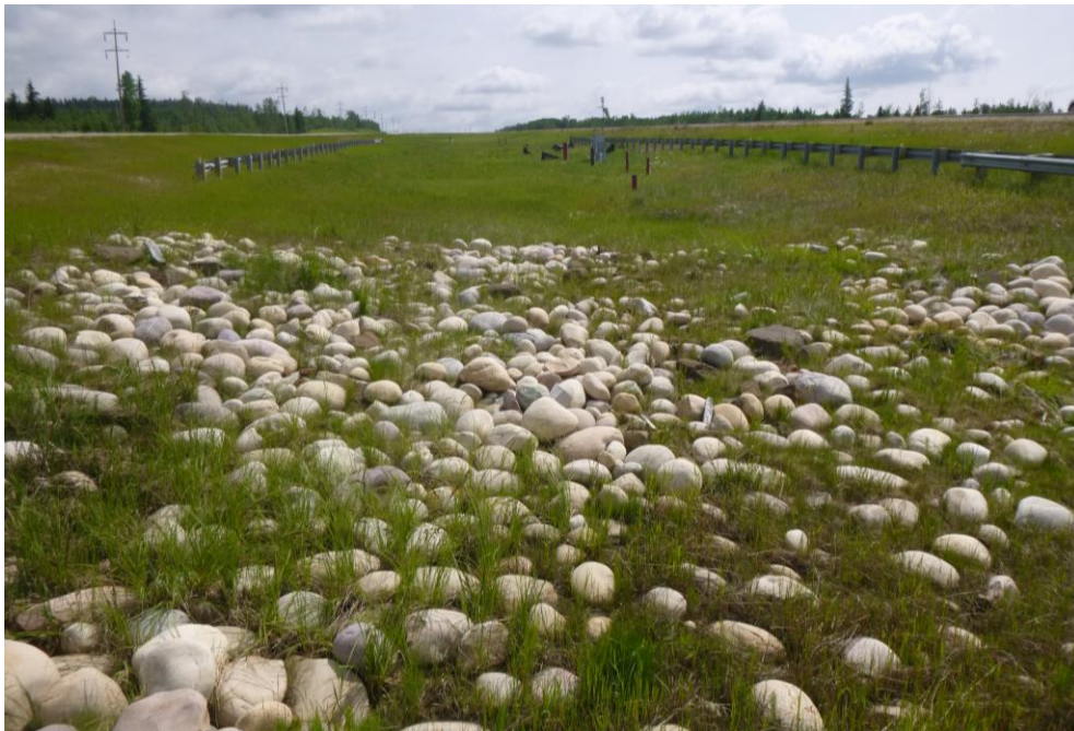
Photo 4 – Looking east along the median at the instrumentation and guardrails from the highway cross culverts.
