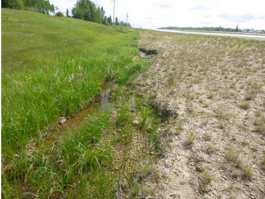
Photo 1 – Looking east at some fresher erosion, caused by flow coming from the bush and bypassing the culvert inlets, and flowing westwards along the south highway ditch.
