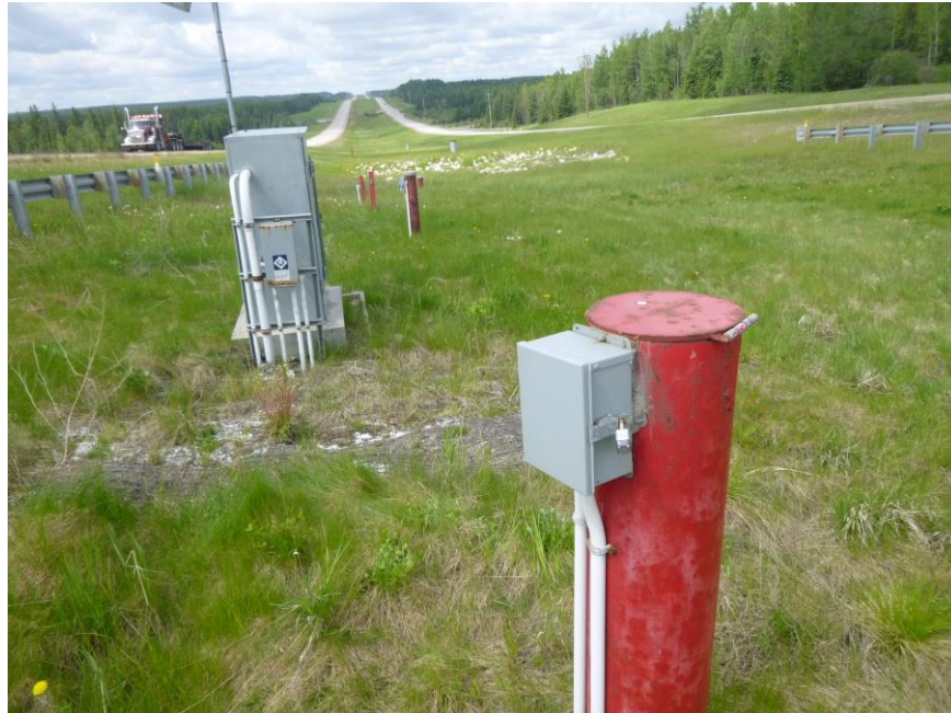
Photo 5 – Looking west along the median at the two pump wells and the Central Monitoring Station (CMS). There are still a couple of small sparsely grassed areas beside the CMS.
