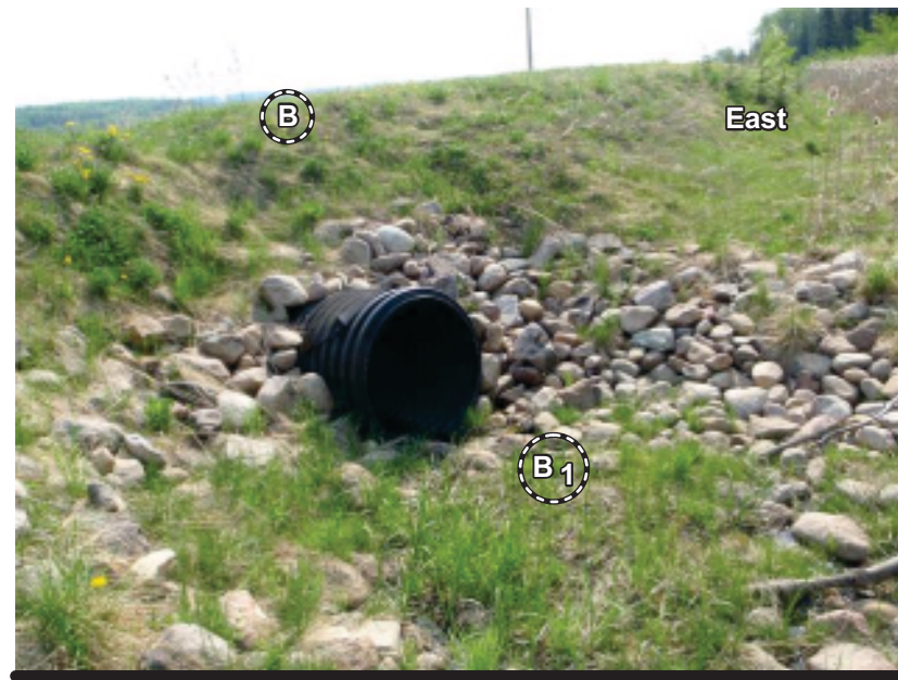
Photo 2 Top of backslope and catchwater ditch • Inlet of buried big “O” for inflow from catchwater ditch
