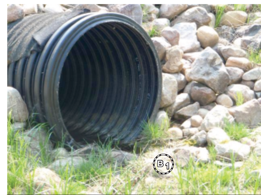
Photo 2c Top of backslope and catchwater ditch • Inlet of buried big “O” for inflow from catchwater ditch
