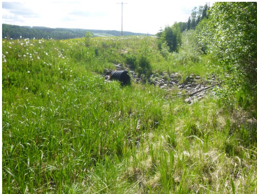
Photo 6 – Looking east along the catch water ditch towards the inlet of the Big O pipe (the inside is squashed on top).
