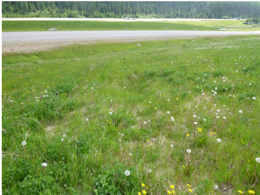
Photo 10 – Looking northeast downslope from ~mid-slope along the settled area and erosion overtop the culvert alignment. Note the settling ponds in the median in the photo background.
