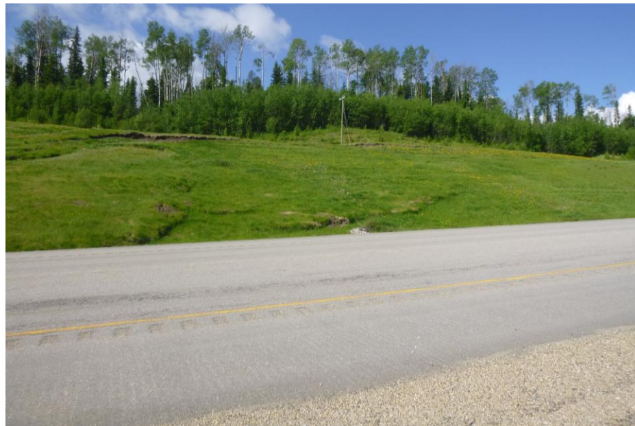
Photo 2 – Looking southeast (upslope) from the highway at the enlarged west side of the embankment slide.
