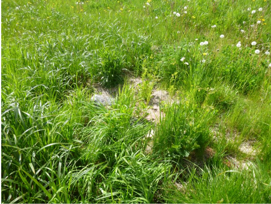
Photo 9 – Looking at a puddle of water on some riprap west of the new slide toe. This may be a possible subdrain outlet.
