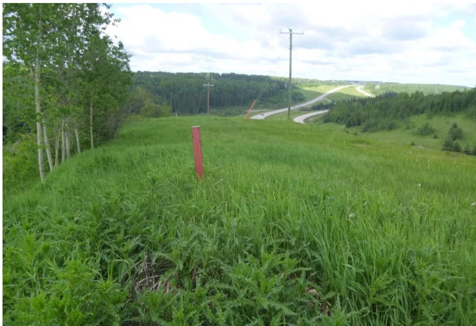
Photo 12 – Looking west along the top of the south cut backslope east of the river. Note the inclinometer casing, which was put in as an early warning indicator of potential movement adjacent to a pipeline if the slump below enlarges.
