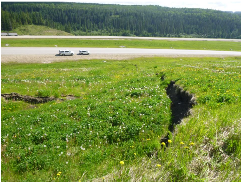
Photo 4 – Looking north downslope along the east edge of the fresh slide.
