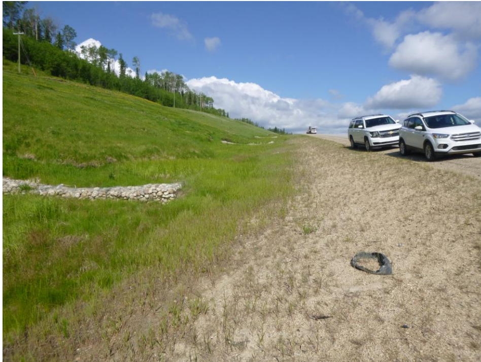
Photo 3 – Looking west at the fresh slide toe encroaching into the south hwy ditch.
