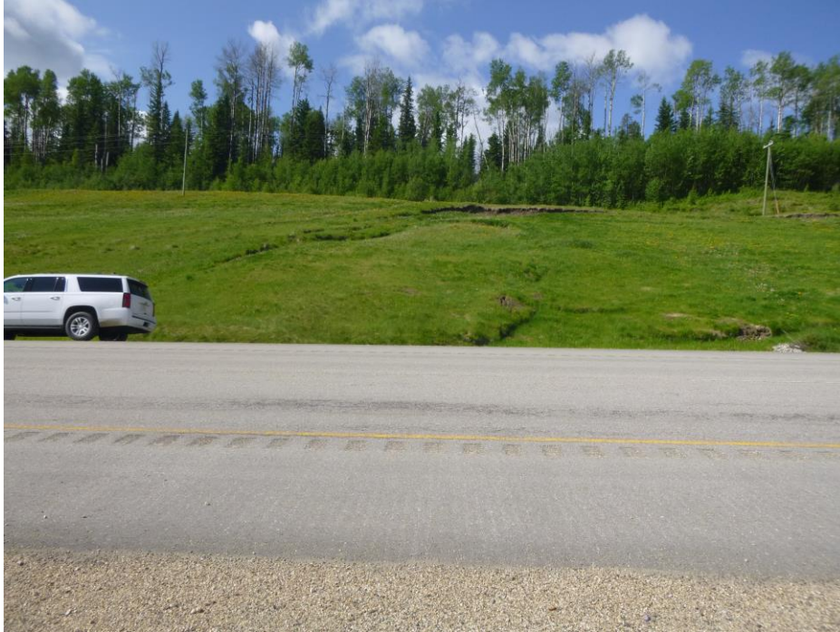
Photo 1 – Looking south (upslope) at the east side of the embankment slide that has fresh movement adjacent to the buried 960 mm diameter “Big O” pipe alignment just east of the slide.
