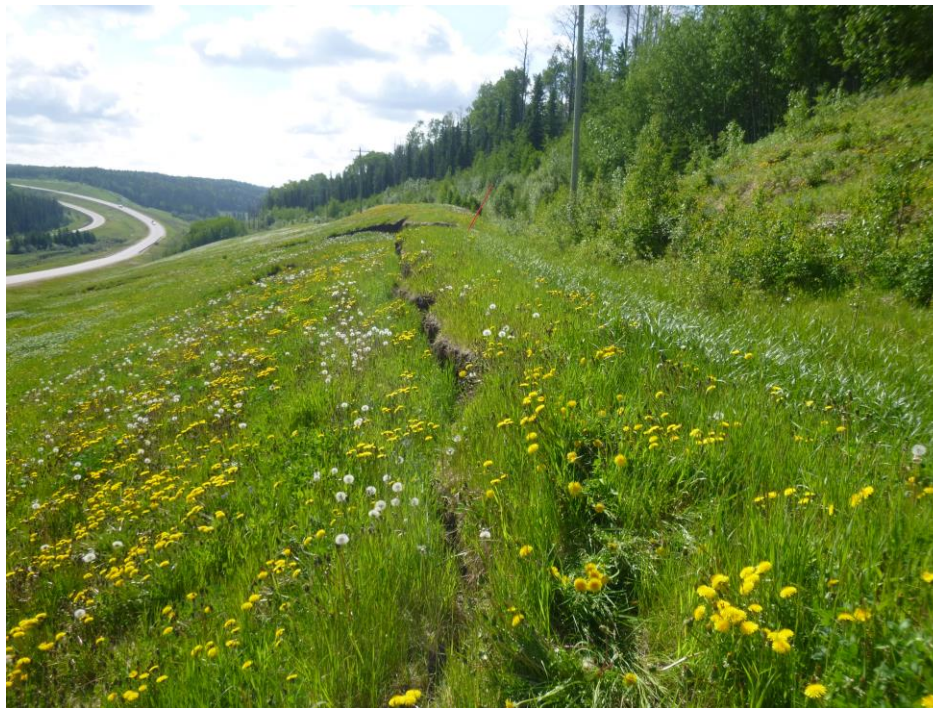
Photo 8 – Looking east along the catchwater ditch and the top of the new slide scarp from the west end.
