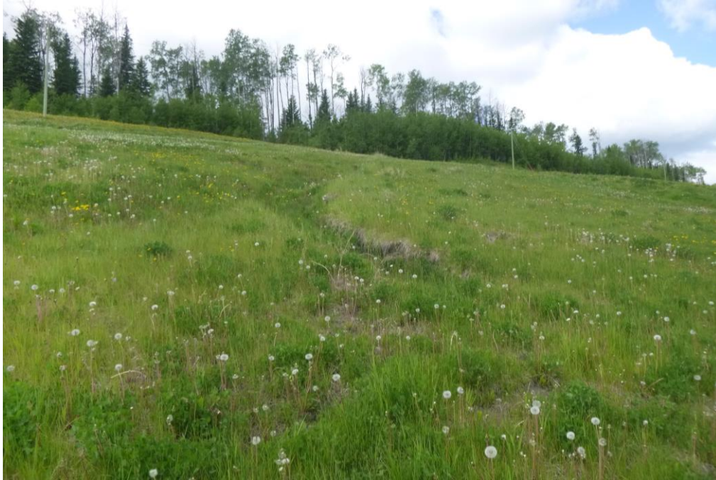
Photo 11 – Looking southwest (upslope) at the sunken depression and erosion overtop the culvert alignment.
