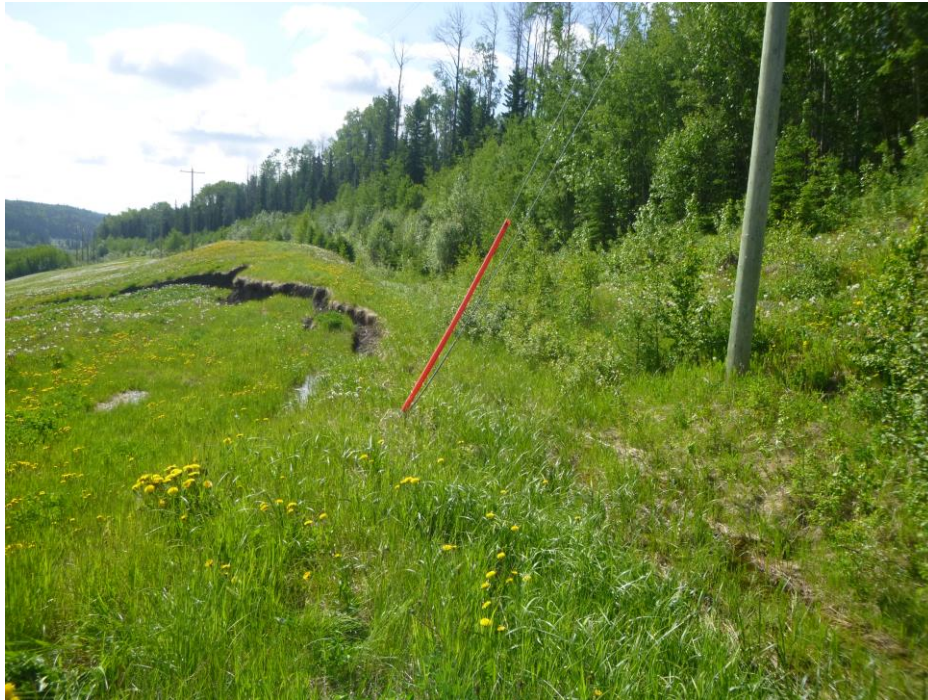
Photo 7 – Looking east along the new slide scarp at the power pole, anchor, and the point where the catchwater ditch breached a short distance east of the power pole anchor.
