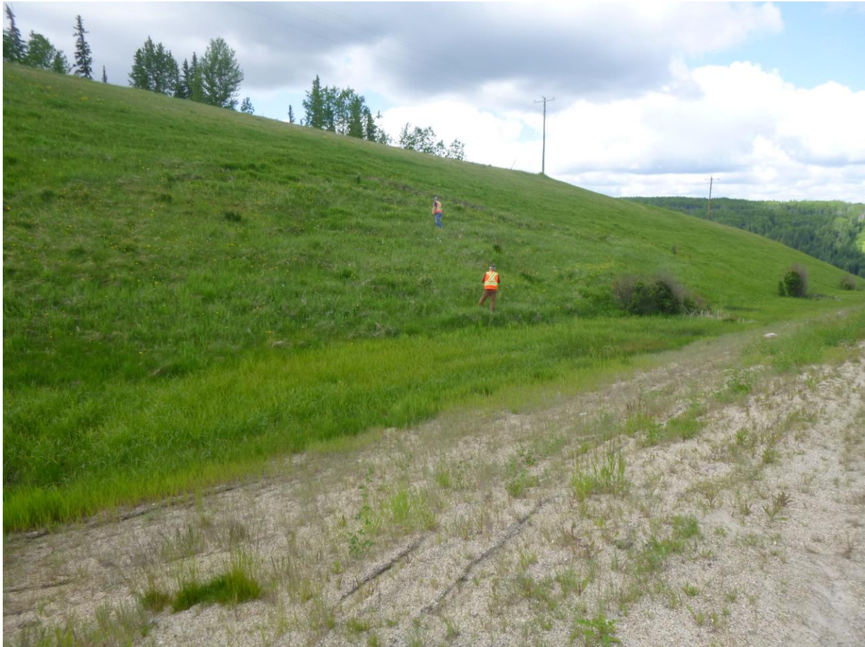
Photo 13 – Looking southwest towards the south cut backslope slide east of the river from the eastbound lanes.
