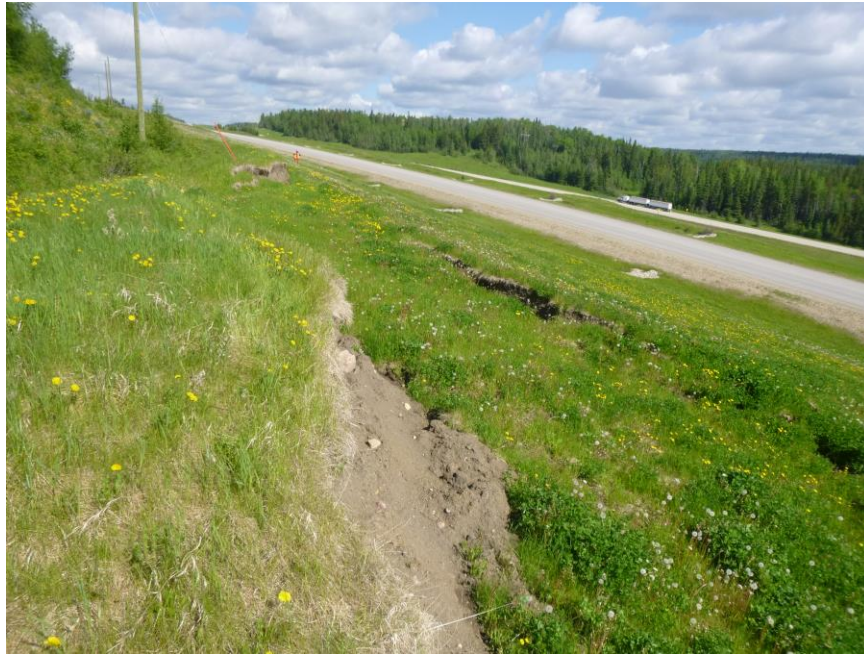
Photo 5 – Looking west along the top of the fresh slide scarp just below the catch water ditch. Note the power pole anchor in the background still intact in a mound of soil but which could soon lose support.
