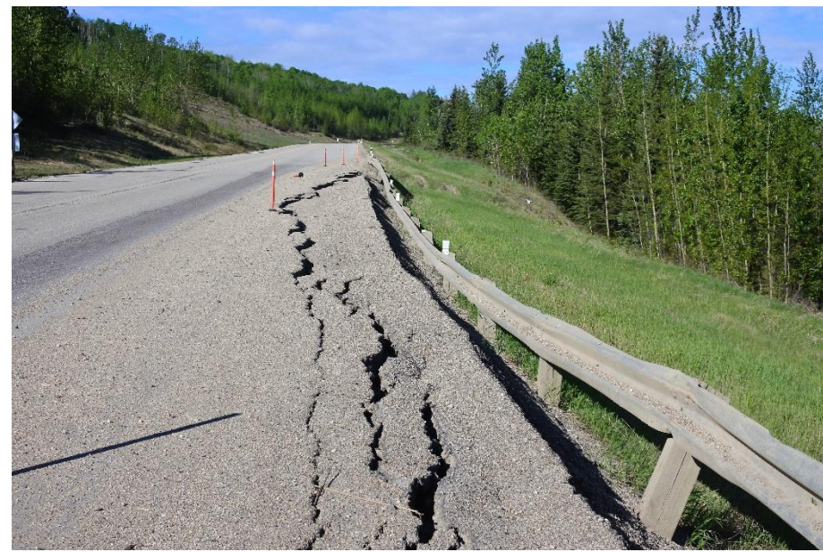
Photo 11. Looking southwest along WBL at the west extent of Lower Valley Landslide (Site 2). The crack is open to 80 mm and drops 90 mm.
