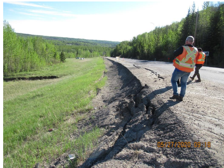
Photo 10. Looking east at overly steep drop off from several layers of ACP patching near the east portion of the Lower Valley Landslide (Site 2).
