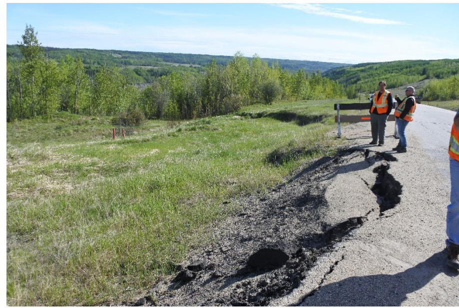
Photo 24. Looking northeast along backscarp near the middle of the Valley Top Landslide (Site 3).
