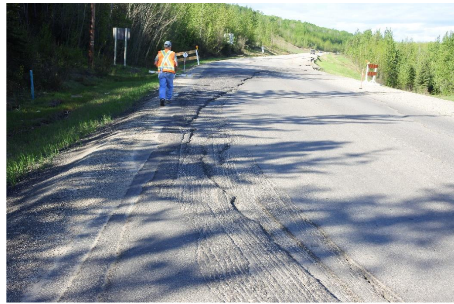
Photo 4. Looking southwest along Hwy 666 at middle portion Lower Valley Landslide (Site 2). The drop along the scarp in the ACP in this section in the roadway surface was up to about 80 mm.
