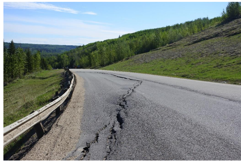
Photo 17. Looking northeast at backscarp in the WBL at Mid-Valley/" Old Major" Landslide (Site 1). The scarp crack is now 100 m wide with a 70 mm drop in the ACP.
