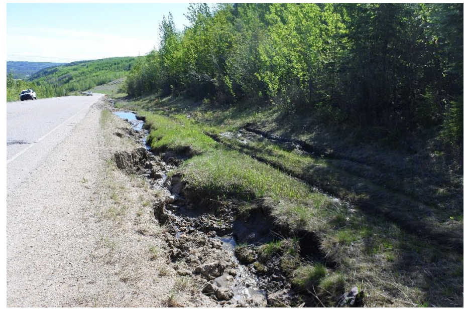
Photo 26. Looking northeast at ditch erosion along the south ditch near the Valley Top Landslide (Site 3).
