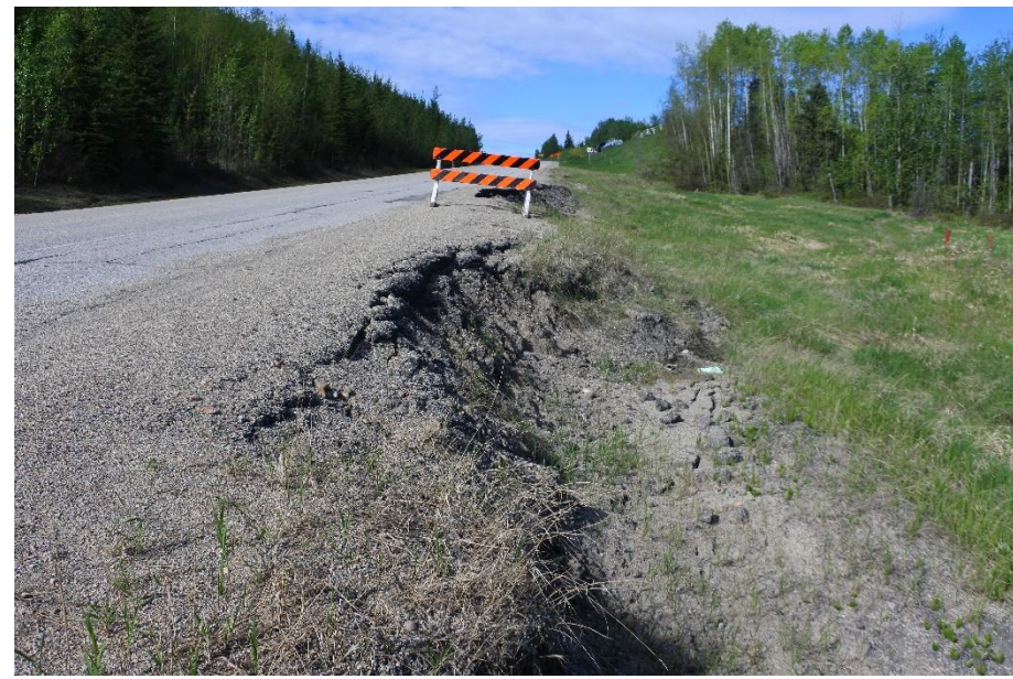
Photo 22. Looking west along backscarp of Valley Top Landslide (Site 3). Backscarp drop in embankment side slope now about 1.6 m
