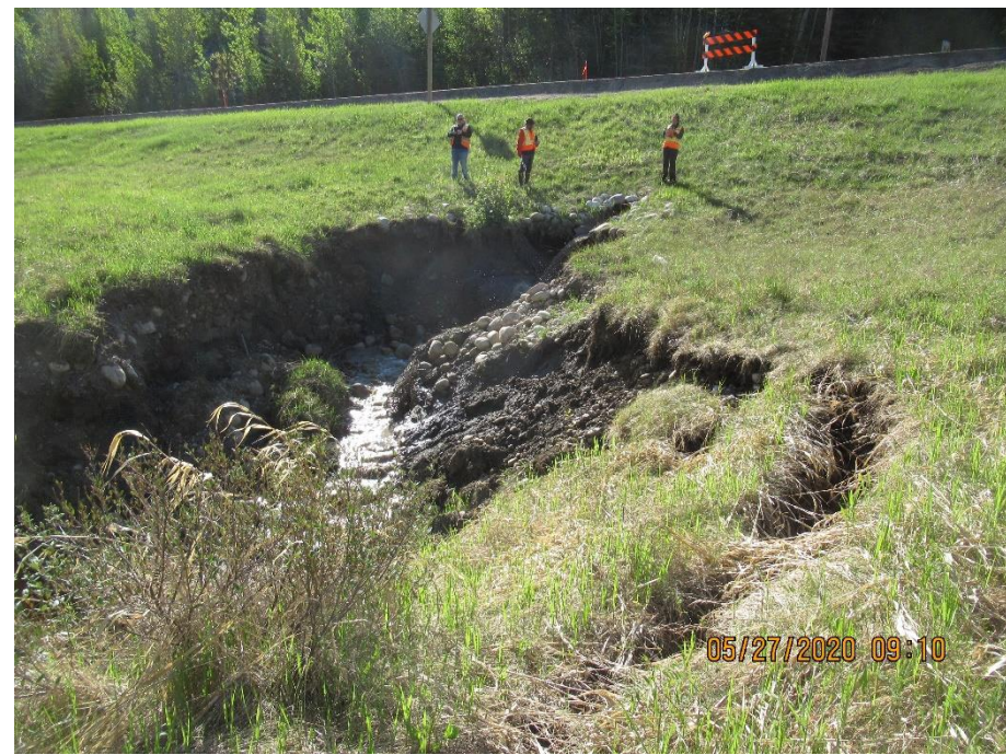
Photo 9. Looking southeast at erosion gully at 600 mm diameter SWSP outlet.
