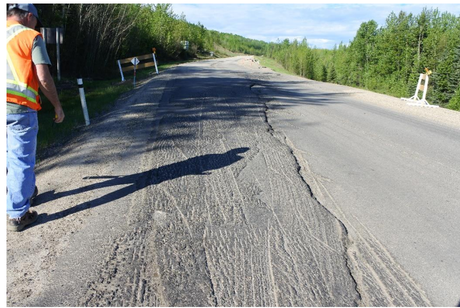
Photo 5. Looking southwest along Hwy 666 near the middle of the Lower Valley Landslide (Site 2). The scarp had asphalt placed and then milled in fall 2019.
