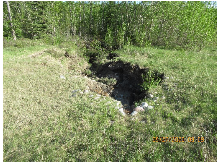
Photo 8. Looking northwest at erosion gully at 600 mm diameter SWSP outlet.
