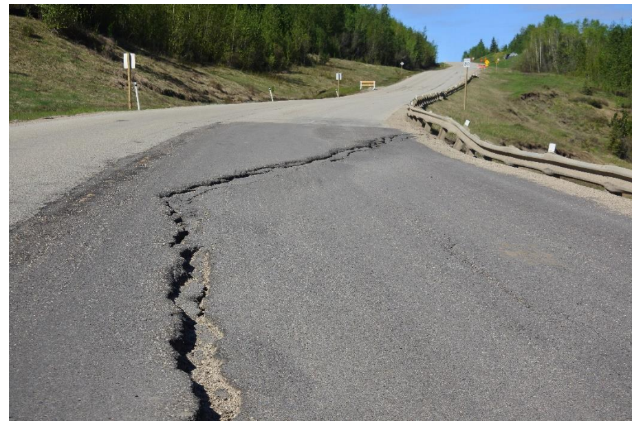
Photo 16. Looking west at the ACP patch in outer WBL at Mid- Valley/" Old Major" Landslide (Site 1). There is a 70 mm drop along the scarp in the ACP and it is open to 100 mm.
