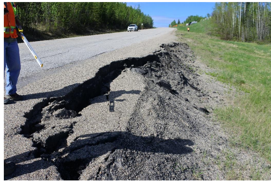
Photo 23. Looking west along backscarp in the west section of the Valley Top Landslide (Site 3). Site was patched in June 2019. Cracks extend past the white line in the WBL and the asphalt has dropped 400 mm.
