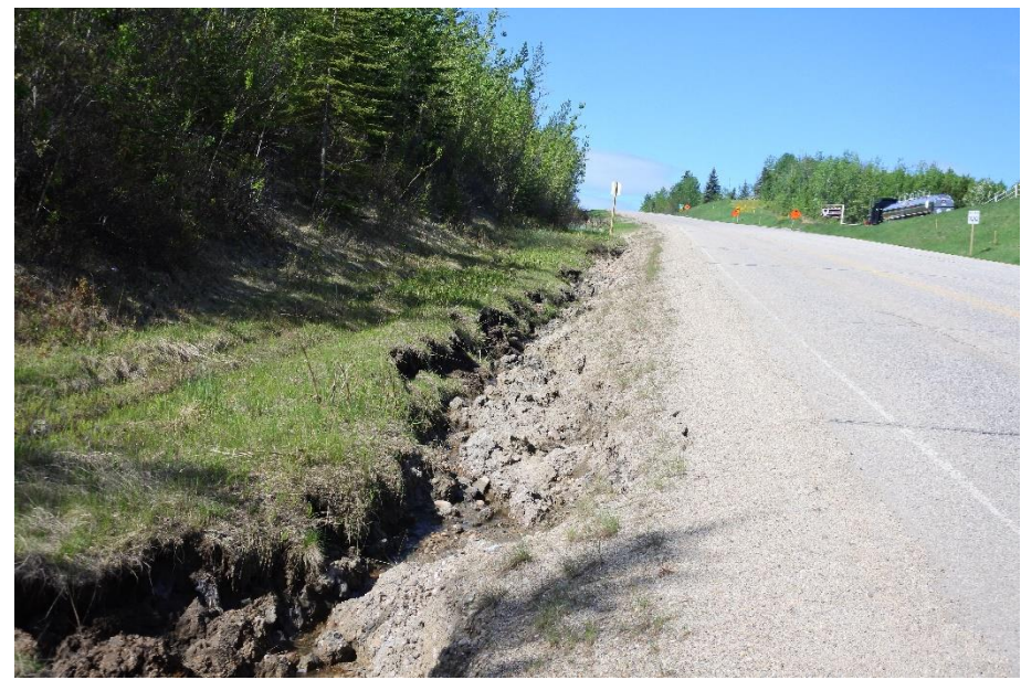
Photo 25. Looking west at erosion in south ditch near the Valley Top Landslide (Site 3).
