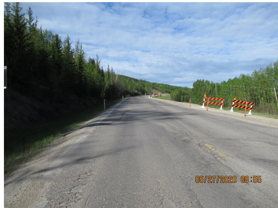
Photo 1. Looking southwest towards the east portion of the Lower Valley Landslide (Site 2).
