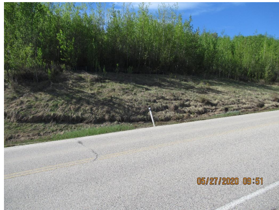
Photo 19. Looking southwest at part of the backslope toe showing recent movement near the Mid-Valley Landslide / "Old Major" (Site 1).
