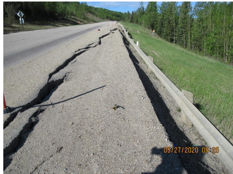
Photo 12. Looking southwest along WBL at the west extent of Lower Valley Landslide (Site 2). The crack is open to 80 mm and drops 90 mm.
