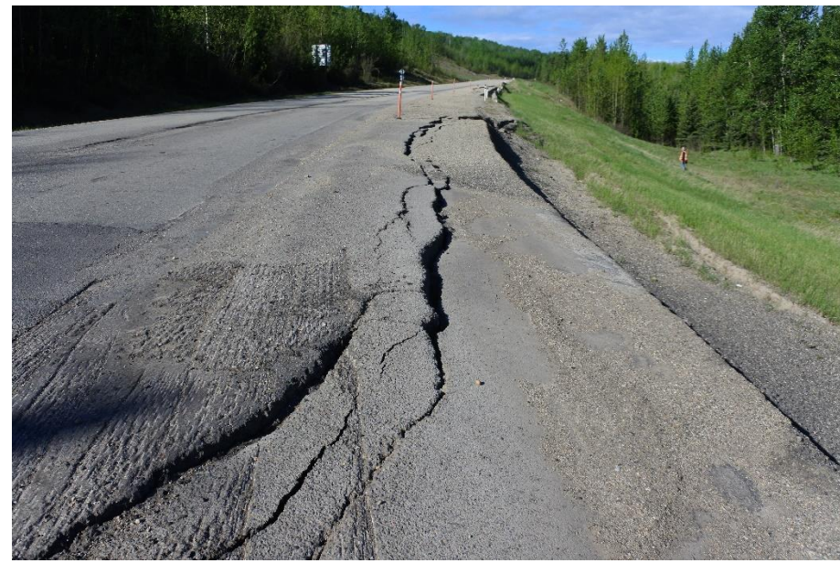
Photo 6. Looking southwest along WBL near middle of the Lower Valley Landslide (Site 2). The scarp has a 90 mm drop in the WBL shoulder.
