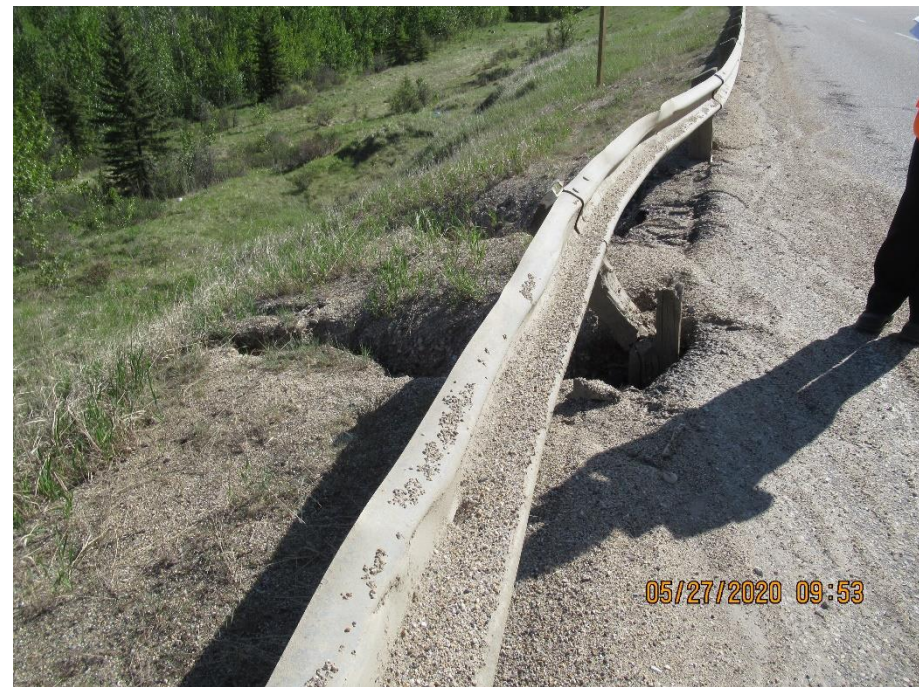
Photo 18. Looking northeast at where guardrail is damaged, and erosion is occurring around the posts and below them.
