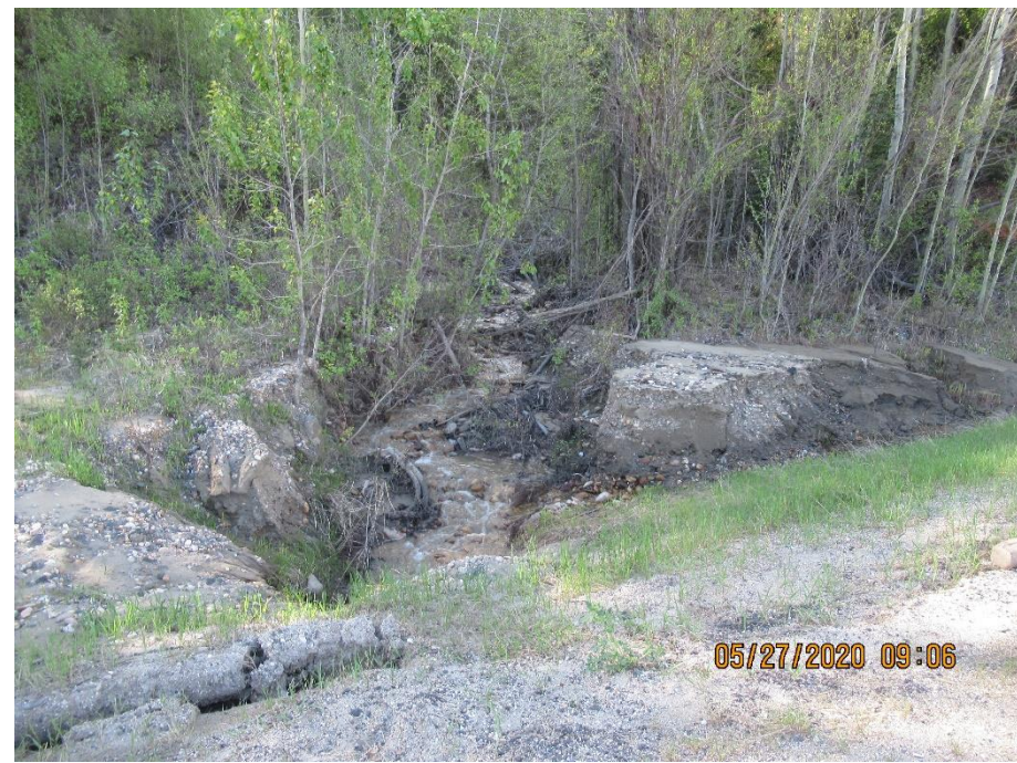
Photo 7. Looking southeast at erosion that has formed in sediment that had accumulating at the 600 mm diameter SWSP inlet, possibly due to the culvert being temporarily frozen.
