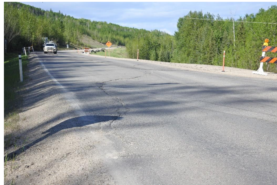
Photo 2. Looking southwest towards the east portion of Lower Valley Landslide (Site 2).
