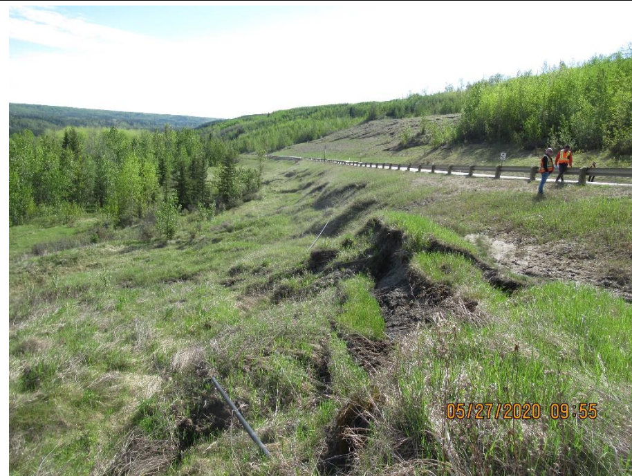
Photo 20. Looking northeast at graben below the highway at the Mid-Valley Landslide / "Old Major" (Site 1) at scarp below the highway and exposed telecommunication cable.
