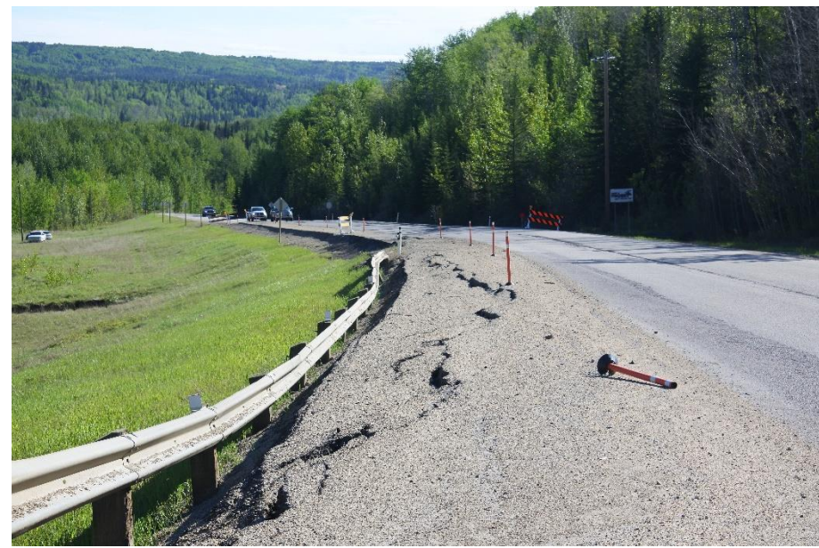
Photo 13. Looking northeast along WBL at the west extent of the Lower Valley Landslide (Site 2).
