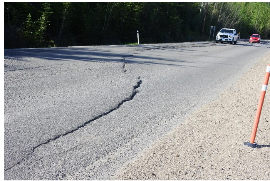
Photo 3. Looking southwest along Hwy 666 at east portion Lower Valley Landslide (Site 2). The drops along the scarp in the ACP in this section in the roadway surface were about 70 mm.
