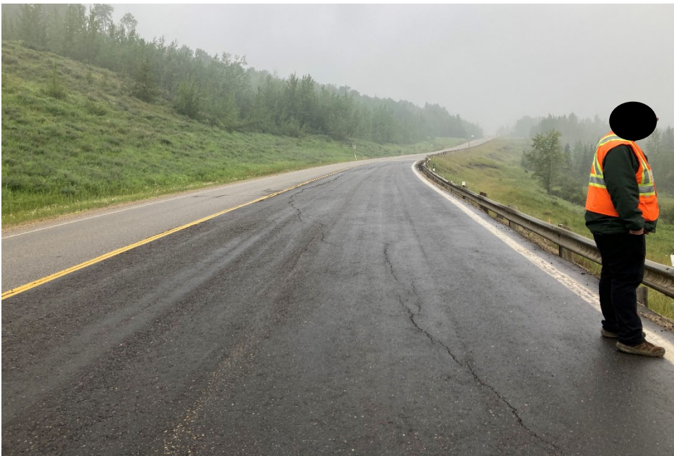
Photo 6 Asphalt cracking observed in the north (westbound) lane of Hwy 666, after the westbound lane was patched in 2020. Photo taken July 20, 2021 facing west.
