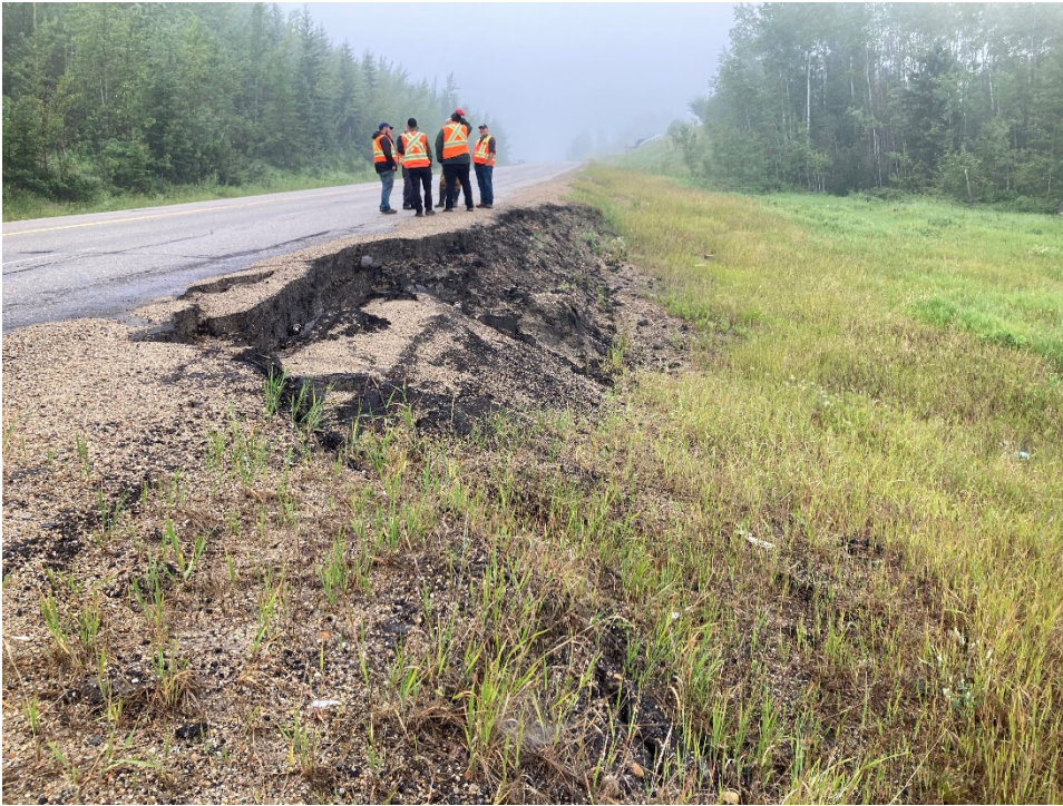
Photo 13 The asphalt of the north (westbound) shoulder is failing. Photo taken July 20, 2021 facing west.
