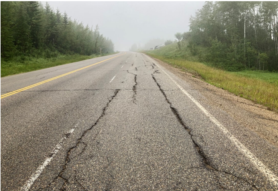
Photo 10 Longitudinal asphalt cracking observed in the north (westbound) travel lane. Photo taken July 20, 2021 facing west.
