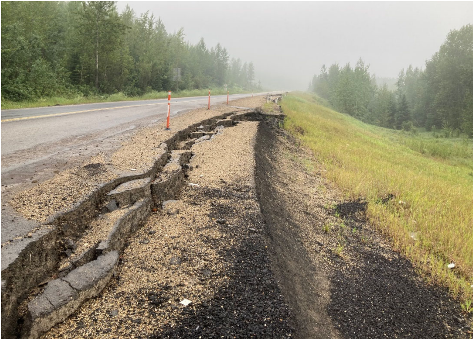
Photo 5 Existing asphalt on the north (westbound) shoulder is breaking away from the highway. Photo taken July 20, 2021 facing west.
