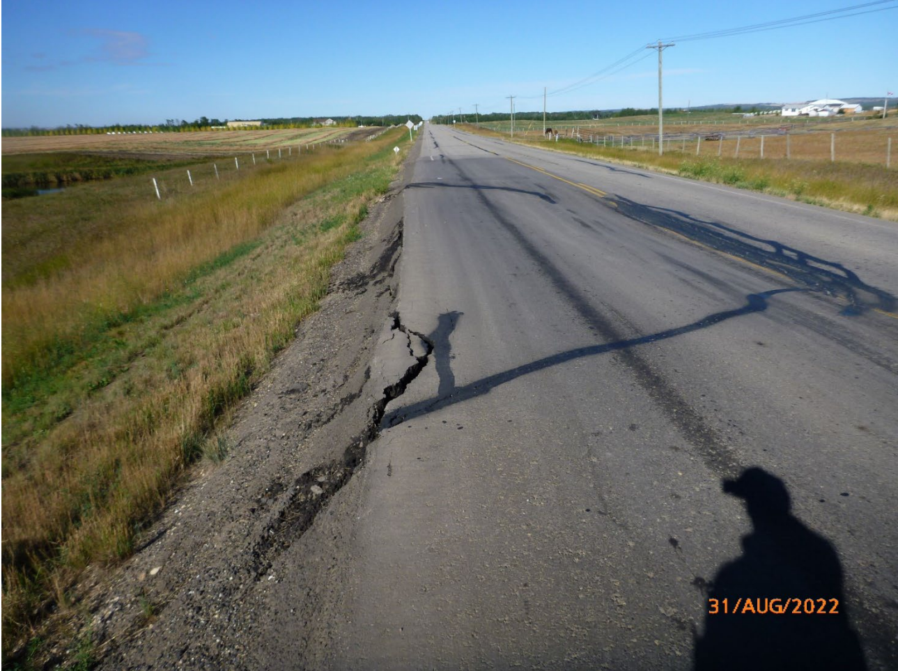
Photo 7 Cracking and separation of asphalt segment at shoulder of eastbound lane. Note that cracking is extending north past centreline. Photo taken August 31, 2022, facing west.
