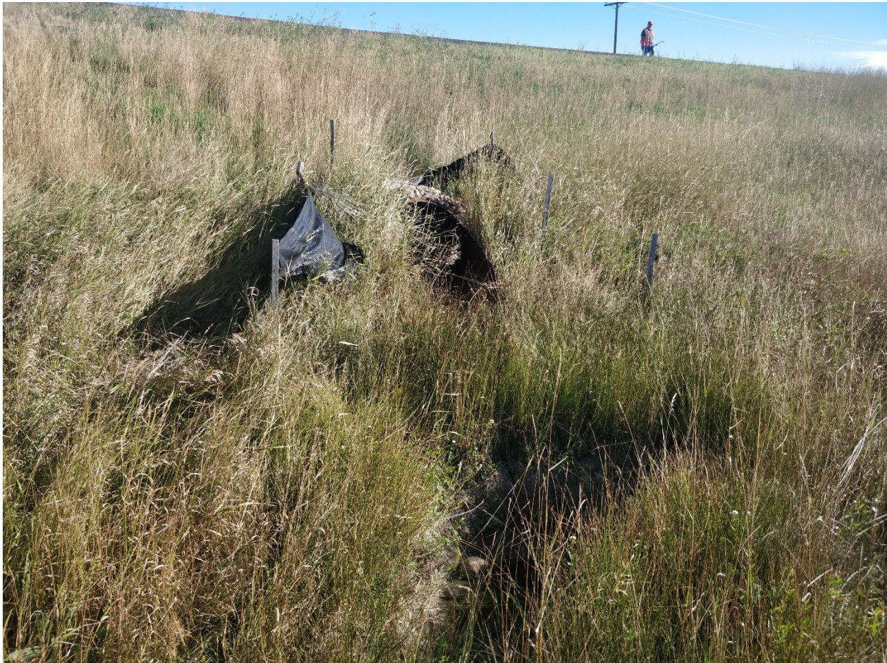
Photo 4 Smooth-wall steel pipe culvert outlet on south embankment, note erosion below point of discharge. Photo taken August 31, 2022, facing northeast.
