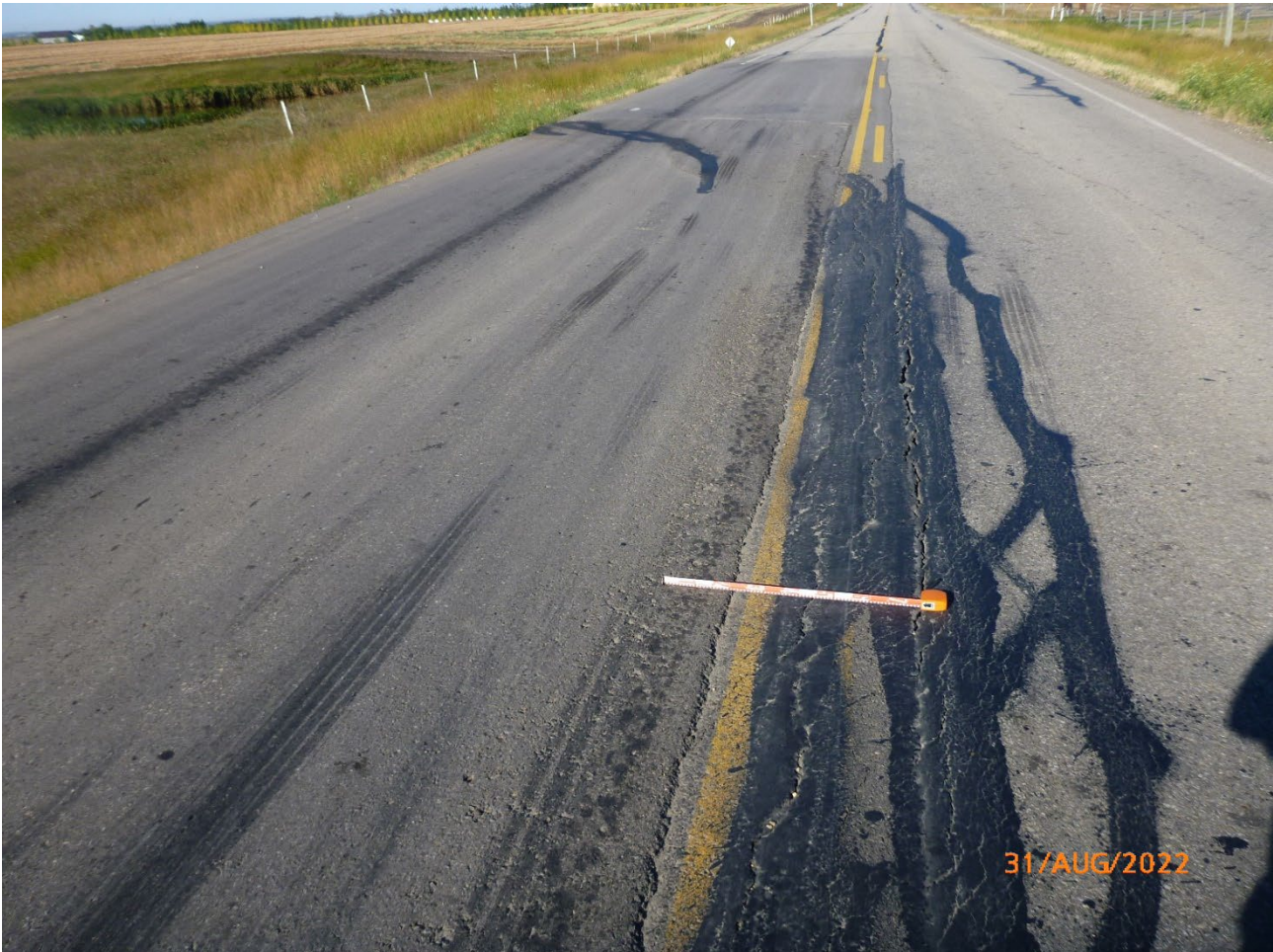
Photo 6 Extent of settlement and cracking observed in east bound lane of highway. Photo taken August 31, 2022, facing west.
