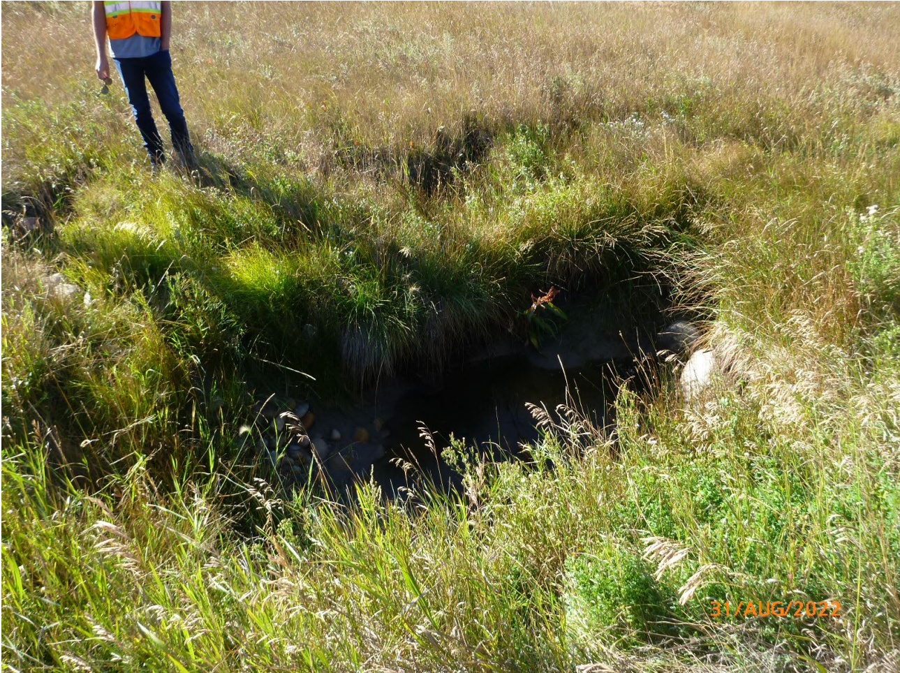
Photo 5 Large depression approximately 5 m away from culvert outlet at toe of south embankment slope. Note eroded rip rap within depression possibly from decommissioned culvert not visible during inspection. Photo taken August 31, 2022, facing southwest
