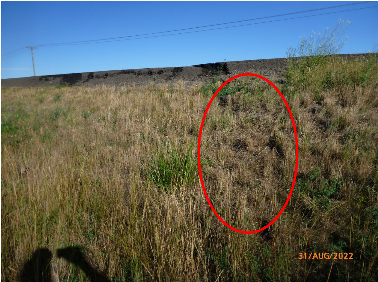
Photo 8 Red circle indicates cracking observed at east side of south embankment slope. Photo taken August 31, 2022, facing north.
