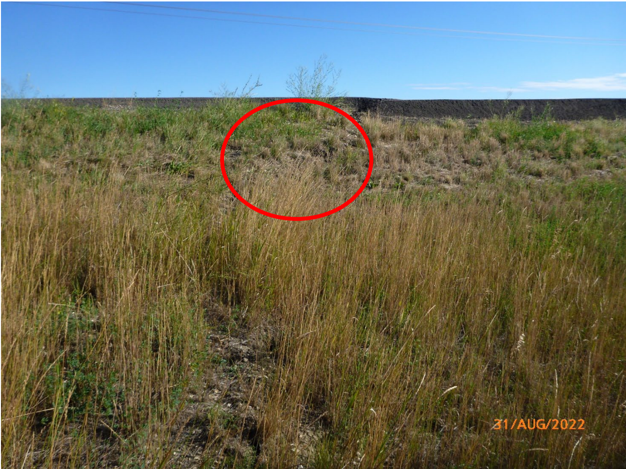
Photo 9 Red circle indicates cracking observed at west side of south embankment. Photo taken August 31, 2022, facing north.
