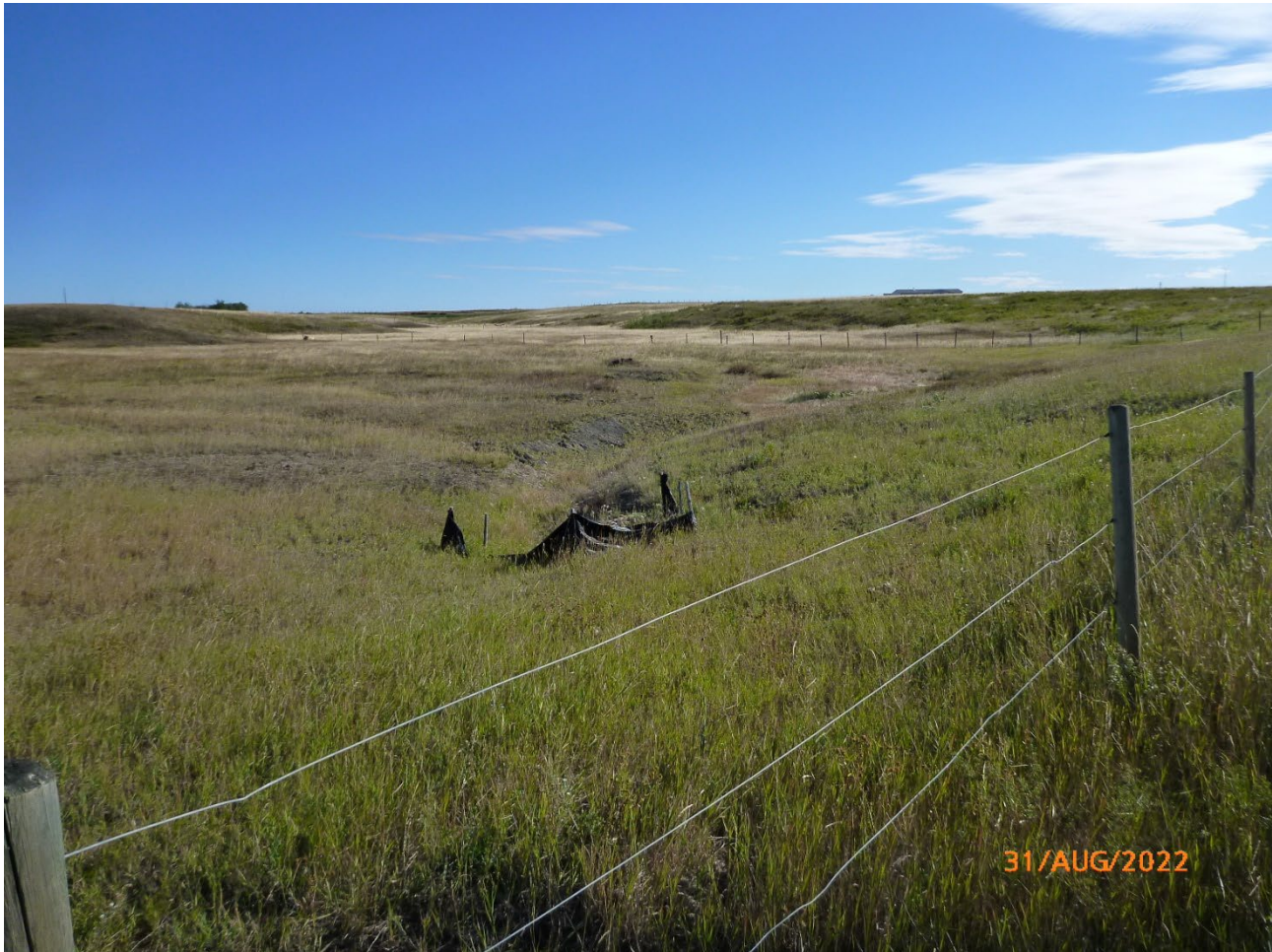
Photo 2 Culvert inlet north of highway and earthworks to direct flow into inlet of smooth-wall steel culvert. Photo taken August 31, 2022, facing northeast.
