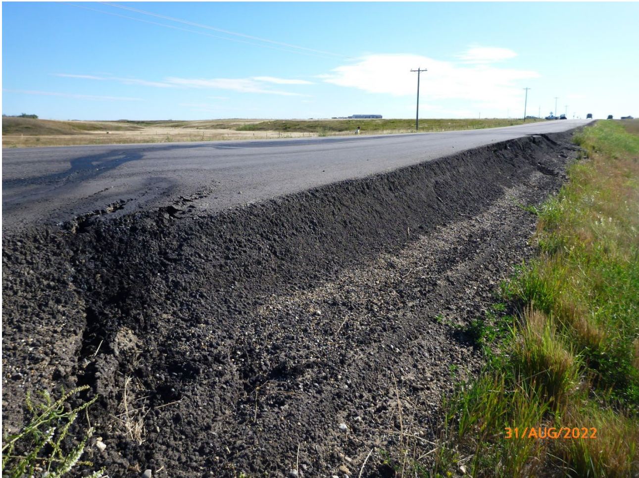
Photo 3 Thickness of asphalt upwards of 1.0 m at western edge of impacted eastbound lane of the highway. Photo taken August 31, 2022, facing northeast.
