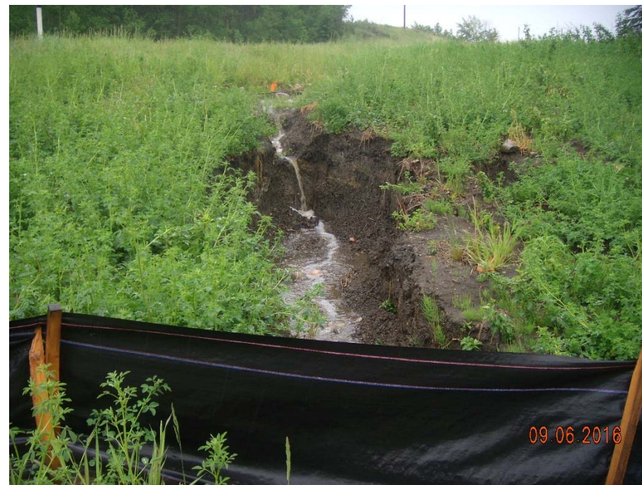
Photo 5. Looking southeast from about 5 m south and 5 m west of the Bear River Bridge south abutment towards the erosion forming at interface between the NBL ditch and the south crest of the Bear River valley slope.
