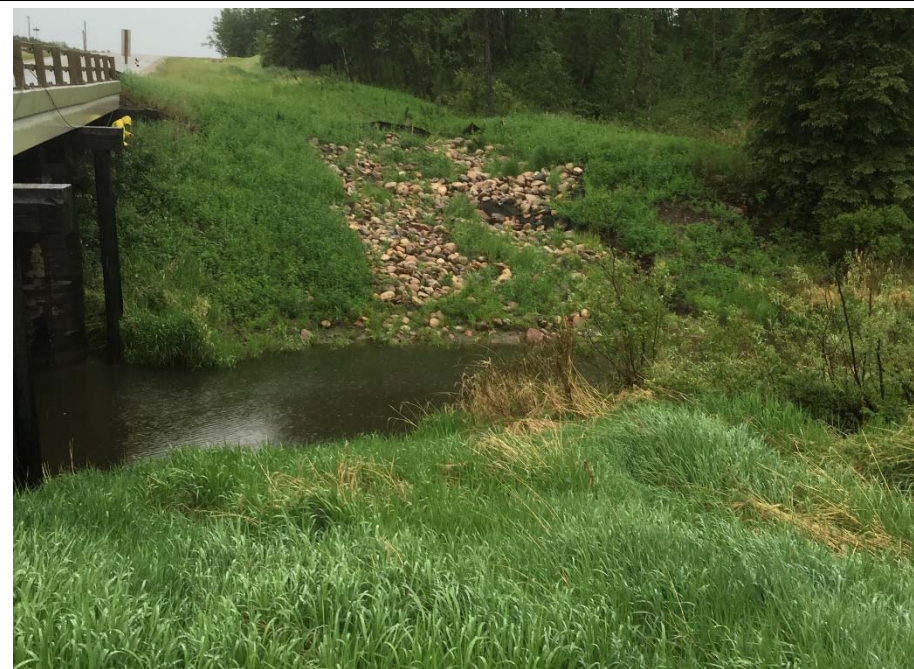
Photo 6. Looking south from about 5m west of the Bear River Bridge north abutment towards the rip rap placed as part of the erosion repair on the south abutment northwest headslope.
