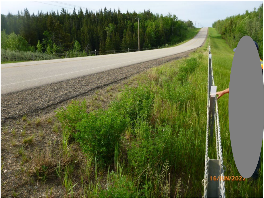
Photo 7 Pavement surface of Hwy 733:02. Note guardrail located downslope from pavement edge. Photo taken June 16, 2022, facing southeast.
