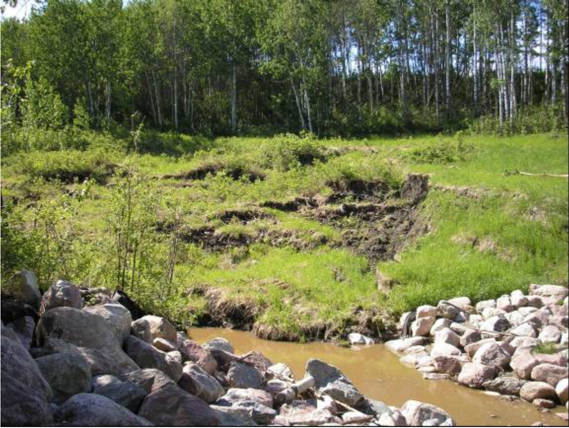
Photo 2 - Southwest view of the slumping at culvert outlet, June 13, 2007.
