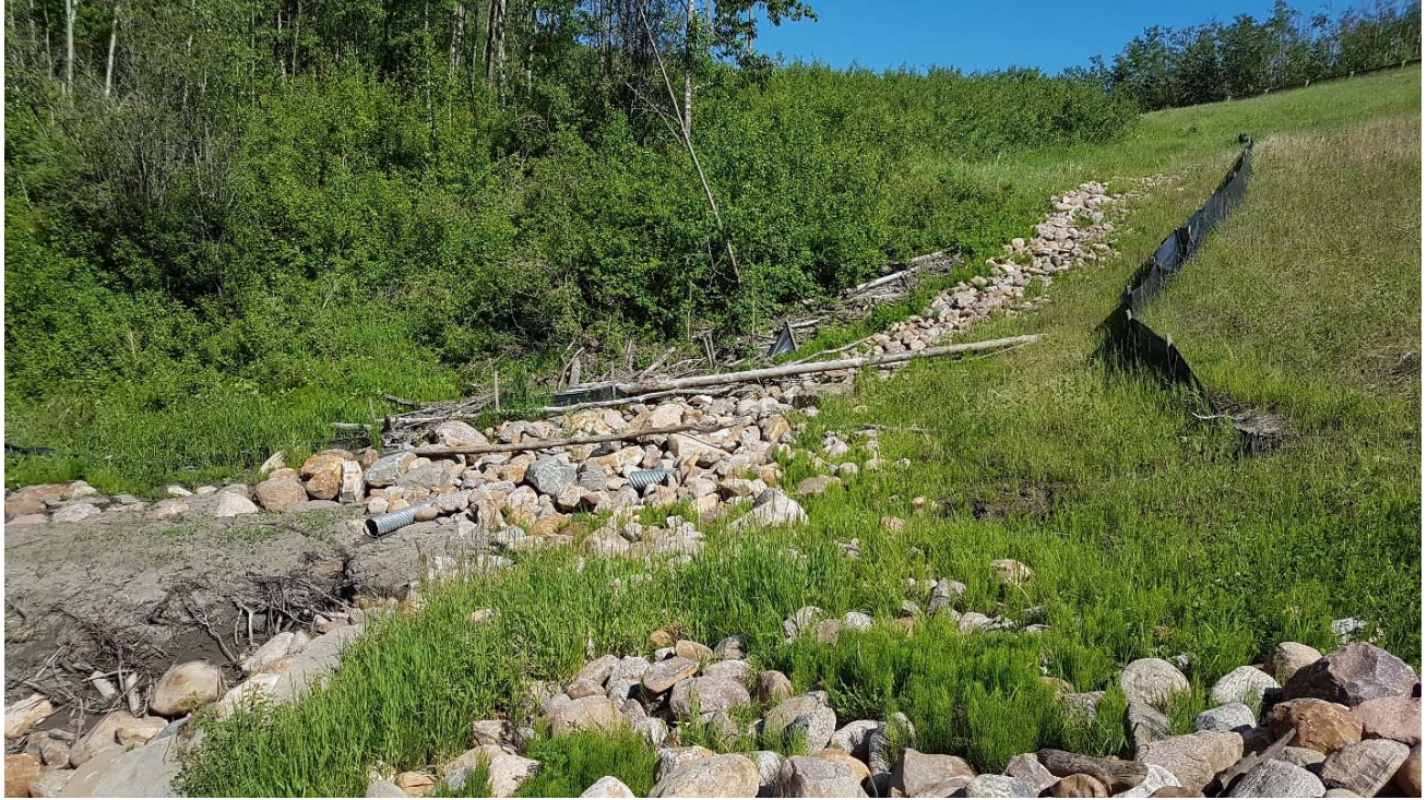
Photo 3 – Looking southeast at riprap-lined ditch channel with two subdrains visible at the toe.
