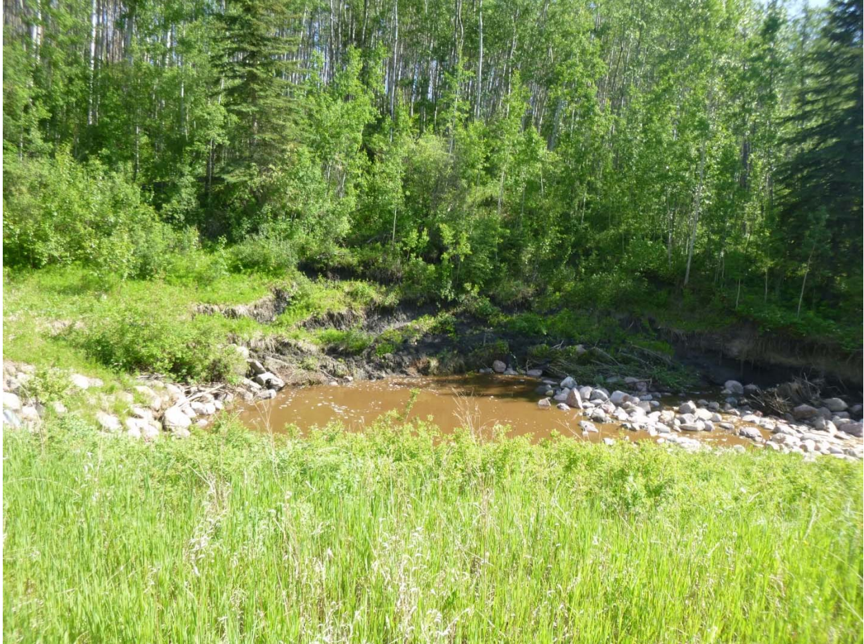
Photo 5 – Looking southeast at eroding bank immediately south of the culvert outlet.
