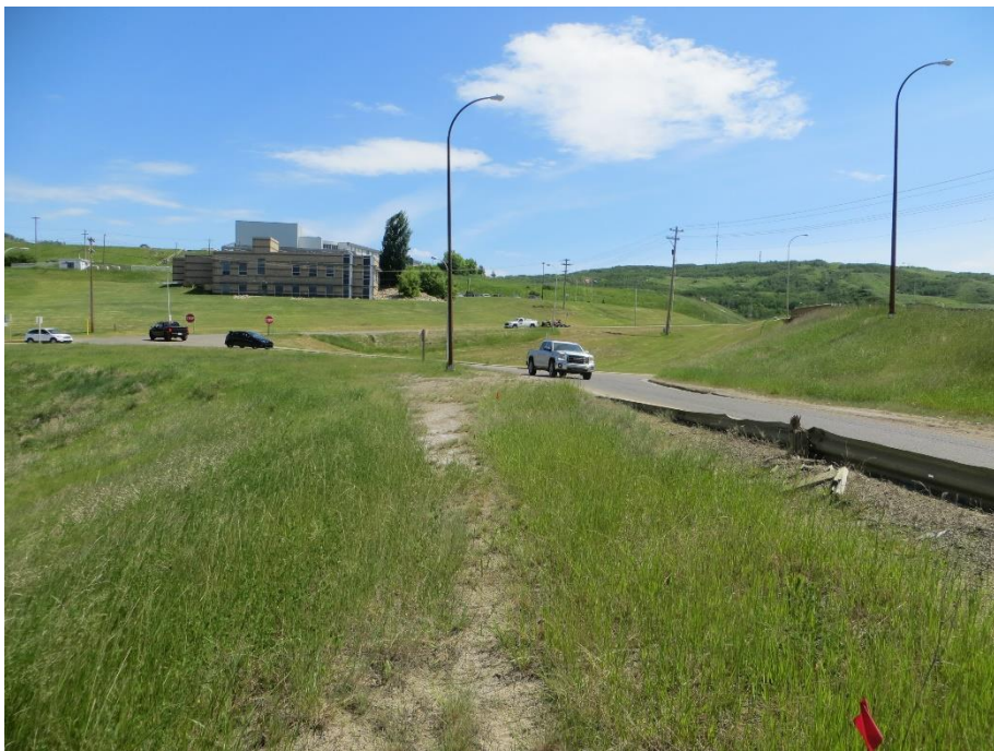
Photo 8. Looking east along the top of bank of the Hwy 2 on-ramp about 120m to the west of 98 Street. There is a slump in the backslope immediately below the cracks in the ACP in the median.
