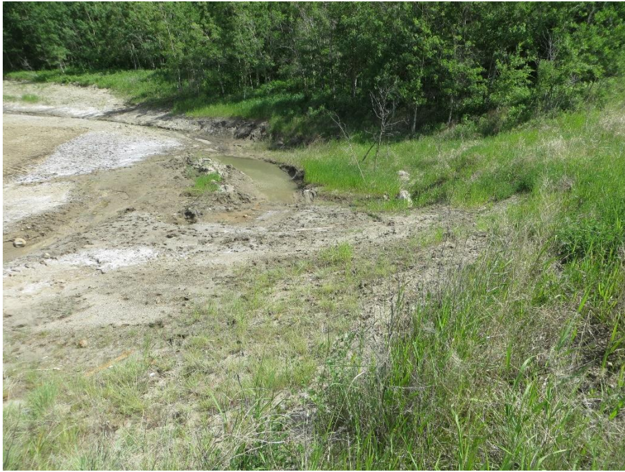
Photo 15. Looking northeast along the toe of the slope below the 98 Street/Hwy 2:60 on-ramp intersection. Some water has ponded at the toe possibly from the culvert discharge immediately upslope of the toe, as well as the seepage from the toe of the slope.
