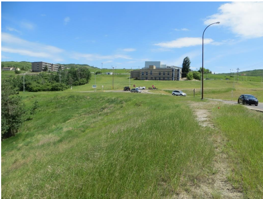
Photo 9. Looking east along the top of bank of the Hwy 2 on-ramp about 90m west of 98 Street. There is a slump in the backslope immediately below the cracks in the ACP in the median.
