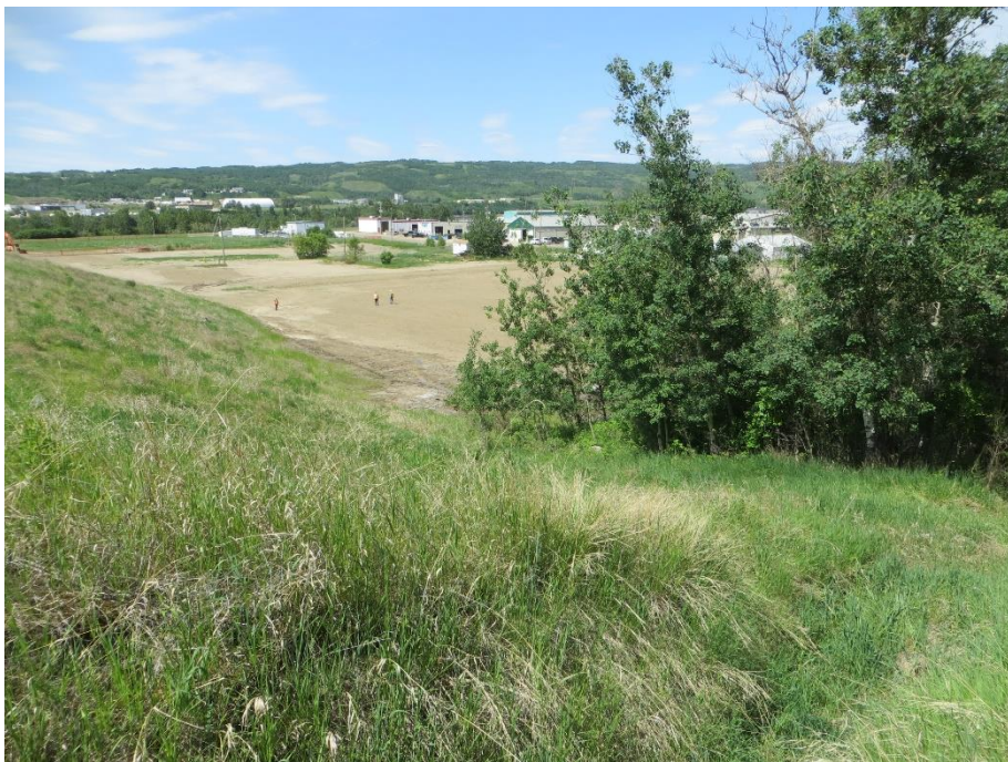
Photo 16. Looking northwest from the crest of the slope above the slump in the sideslope.
