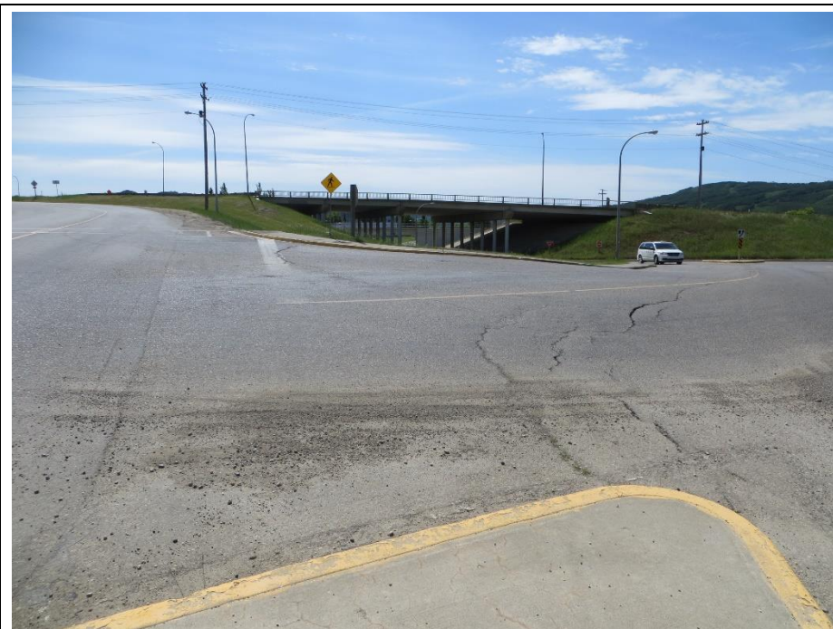
Photo 5. Looking south from the median at the 98 Street/Hwy 2 on-ramp intersection. The cracks in the pavement (ACP) are open from 50mm to 80mm and there is a distinct dip in the pavement about 9.5m from the edge of the curb on the west side of 98 Street.
