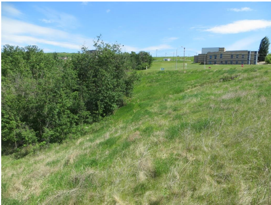
Photo 7. Looking east from the Hwy 2 on-ramp sideslope about 120m to the west of 98 Street. There is a slump in the backslope immediately below the cracks in the ACP in the median.
