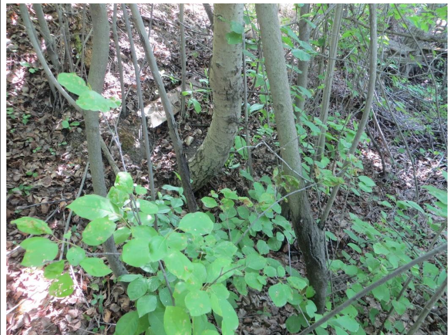
Photo 19. Looking at a bent tree trunk at the lower mid-slope in the area assessed to be within the landslide.
