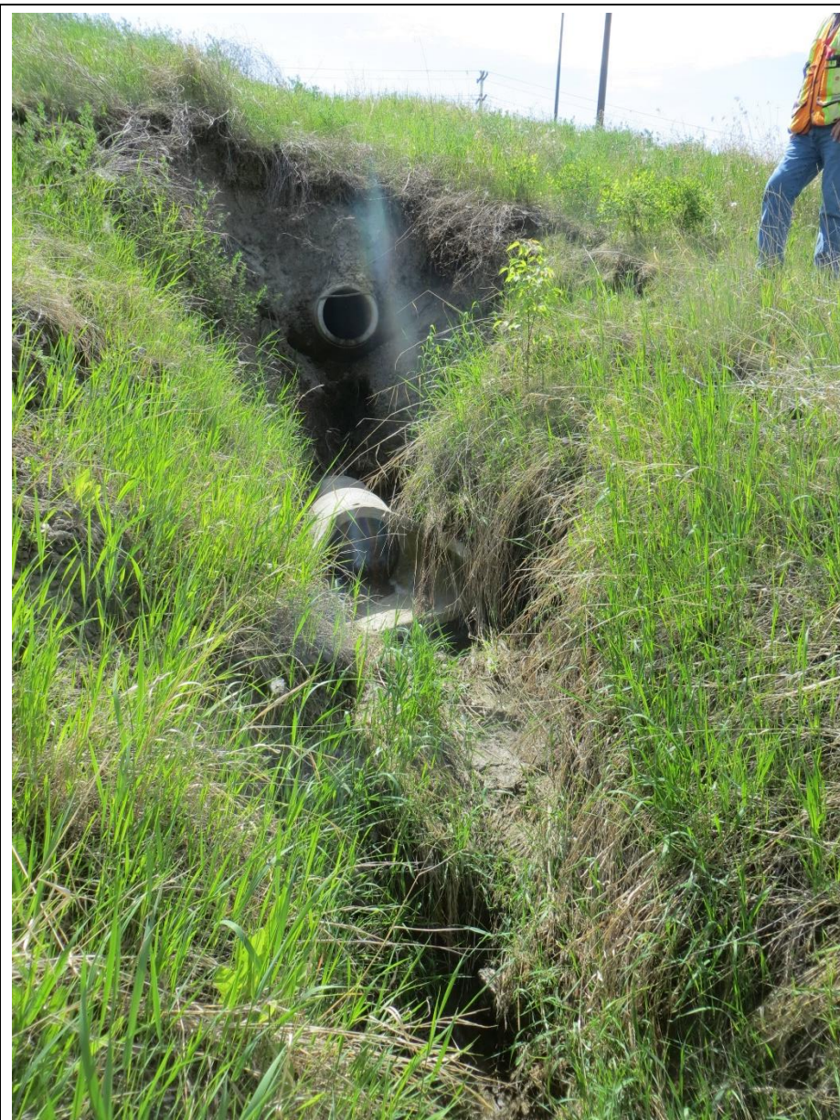
Photo 17. Looking south at the disconnected 460 mm OD drain pipe in the backslope below the 98 Street/Hwy 2:60 on-ramp intersection and the scour channel that has developed below.
