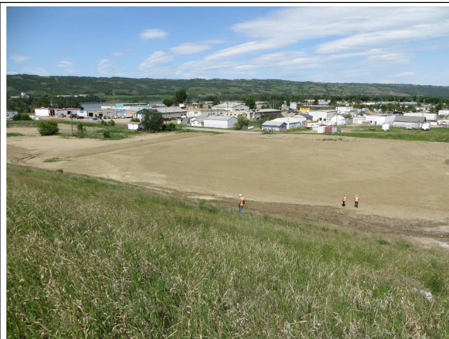
Photo 11. Looking northwest from the 98 Street/Hwy 2:60 on-ramp shoulder towards the former Alberta Transportation yard that has been regraded as part of the salt contamination remediation in the spring of 2017.
