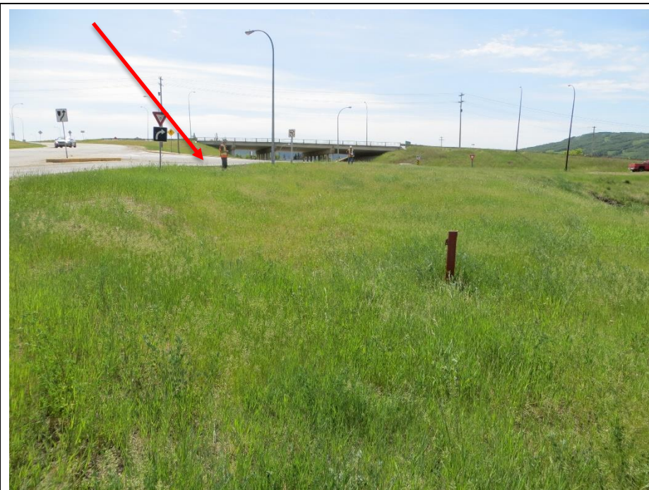
Photo 3. Looking southeast towards the 98 Street/Hwy 2 on-ramp intersection. There is a distinct dip in the curb along the projection of the cracks observed in the pavement on 98 Street.
