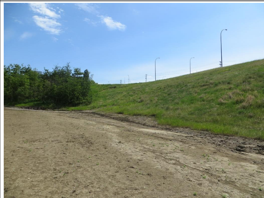
Photo 14. Looking east along the toe of the slope of the Hwy 2:60 on-ramp. The slope is about 13m in height. There are signs of seeping, flowing and ponding water along the toe of the slope. This area was regraded as part of the salt contamination remediation in the spring of 2017.
