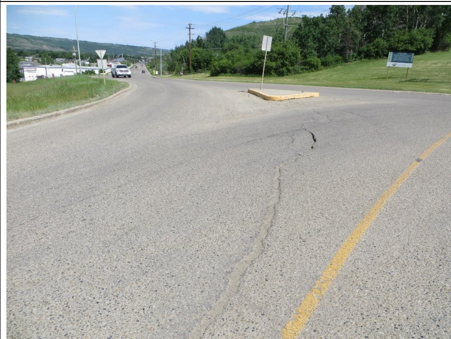
Photo 6. Looking northeast towards the median at the 98 Street/Hwy 2 on-ramp intersection. The cracks in the ACP are open from 50mm to 80mm and there is a distinct dip in the ACP about 9.5m from the edge of the curb on the west side of 98 Street.
