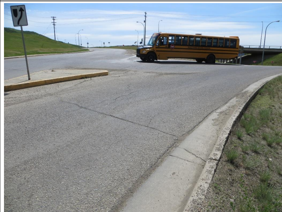
Photo 4. Looking southeast along the cracks in the pavement at the 98 Street/Hwy 2 on-ramp intersection.
