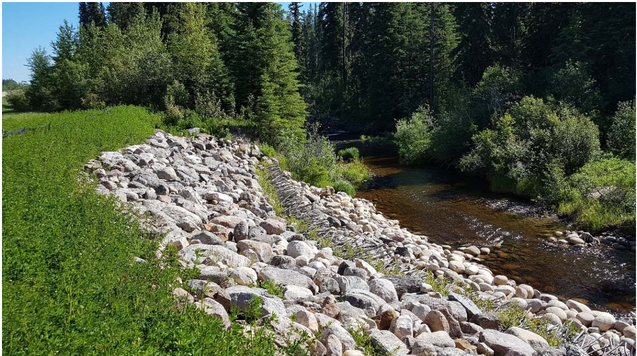
Photo 2 – Looking north at rebuilt left creek bank. Note willow growth from base of plantings in the brush layering at midslope.
