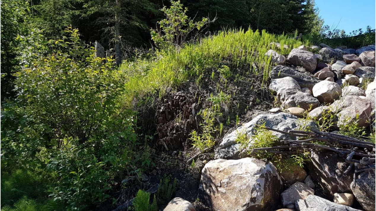
Photo 3 – Looking at minor erosion at south tie-in of riprap protection.
