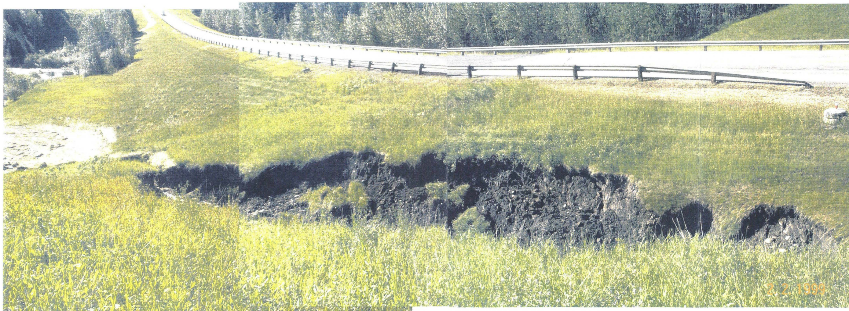
VIEW OF ERODED SECTION OF EMBANKMENT ON NORTH SIDE OF HIGHWAY 33
