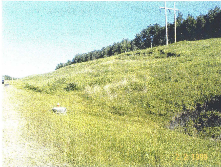
VIEW OF NORTH EMBANKMENT SLIDE AREA LOOKING WEST
