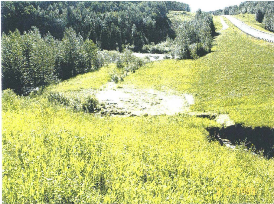
VIEW OF MATERIAL ERODED FROM EMBANKMENT AT BASE OF SLOPE LOOKING EAST
