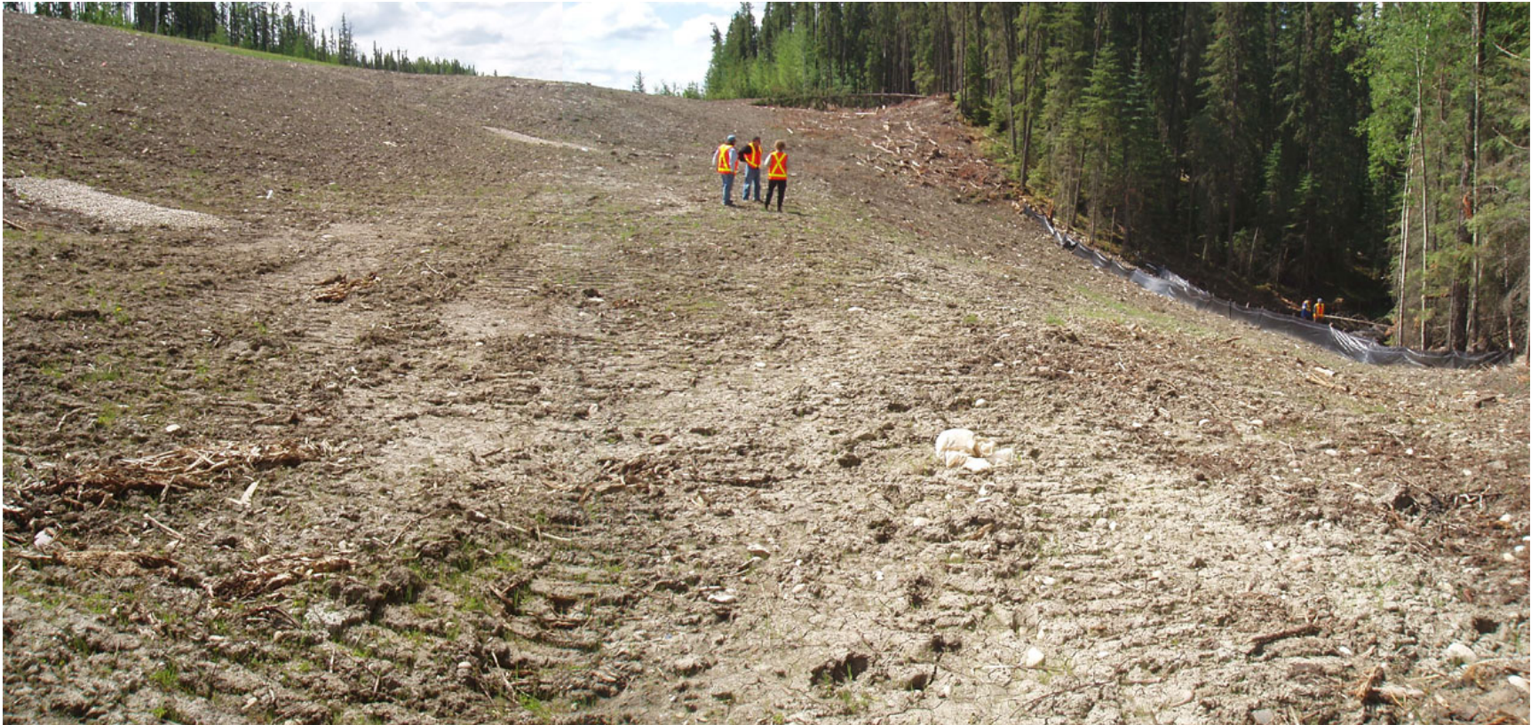
Photo 1: Looking south to southwest along slope at gravel drains and culvert outlet.
