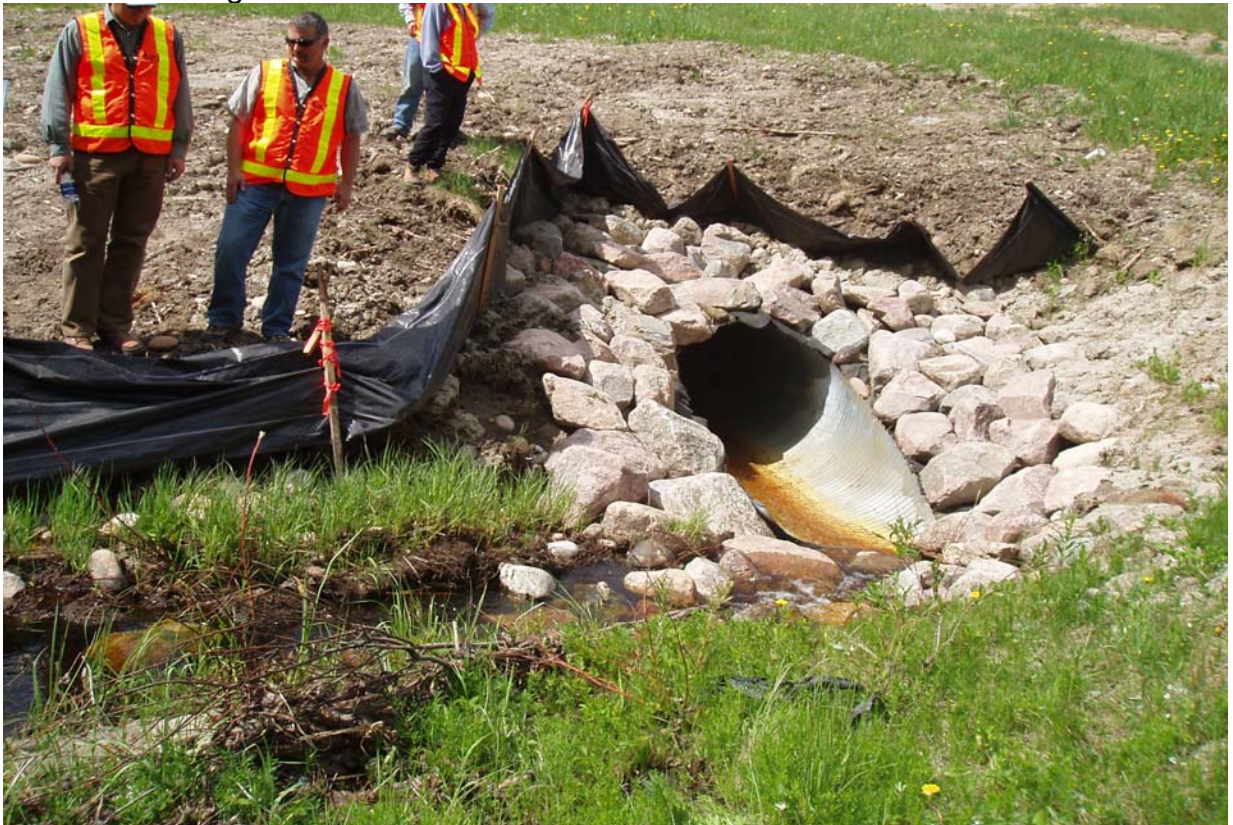
Photo 3: Looking west at culvert inlet. Note sharp channel bend in front of culvert and riprap higher than inlet.
