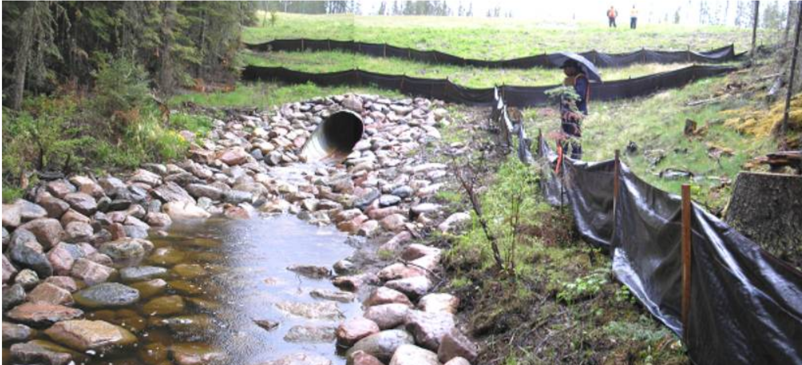
Photo 2 - Looking northeast at culvert outlet. Note loose silt fence south of creek, May 23, 2006.
