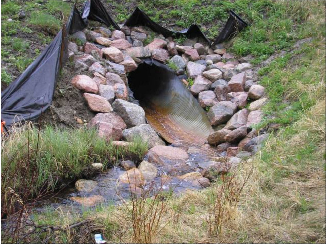
Photo 3 - Looking west at culvert inlet. Note sharp channel bend in front of culvert and riprap higher than inlet, May 23, 2006.
