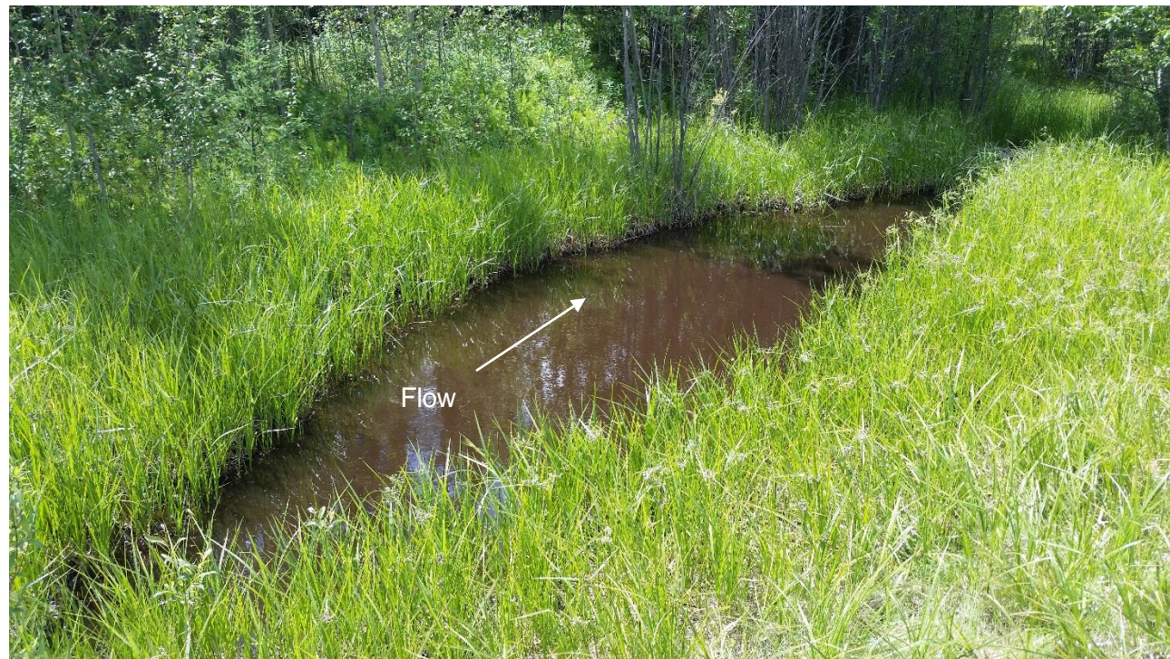
Photo 2: (looking west) Looking at pond downstream of culvert inlet west of Highway 33. Culvert outlet is completely submerged. Similar conditions have been observed since the 2012 inspection.
