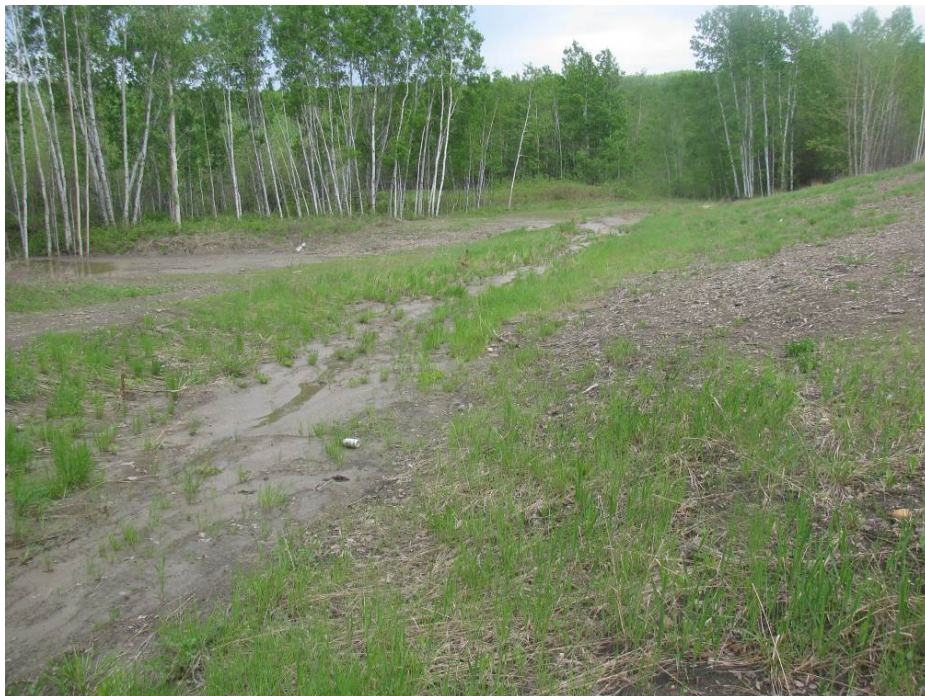
Photo 4 – Erosion control soil covering at the toe of the slope, looking northeast.
