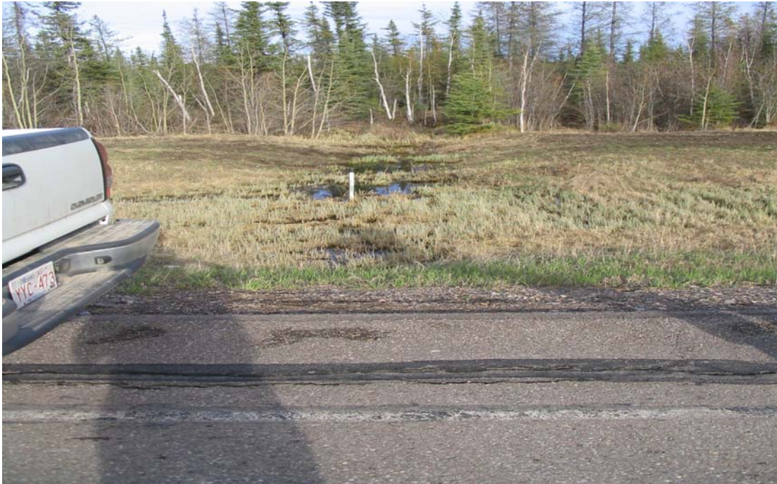
PHOTO 9: Longitudinal cracks and incoming creek on east side of road at Site B.
