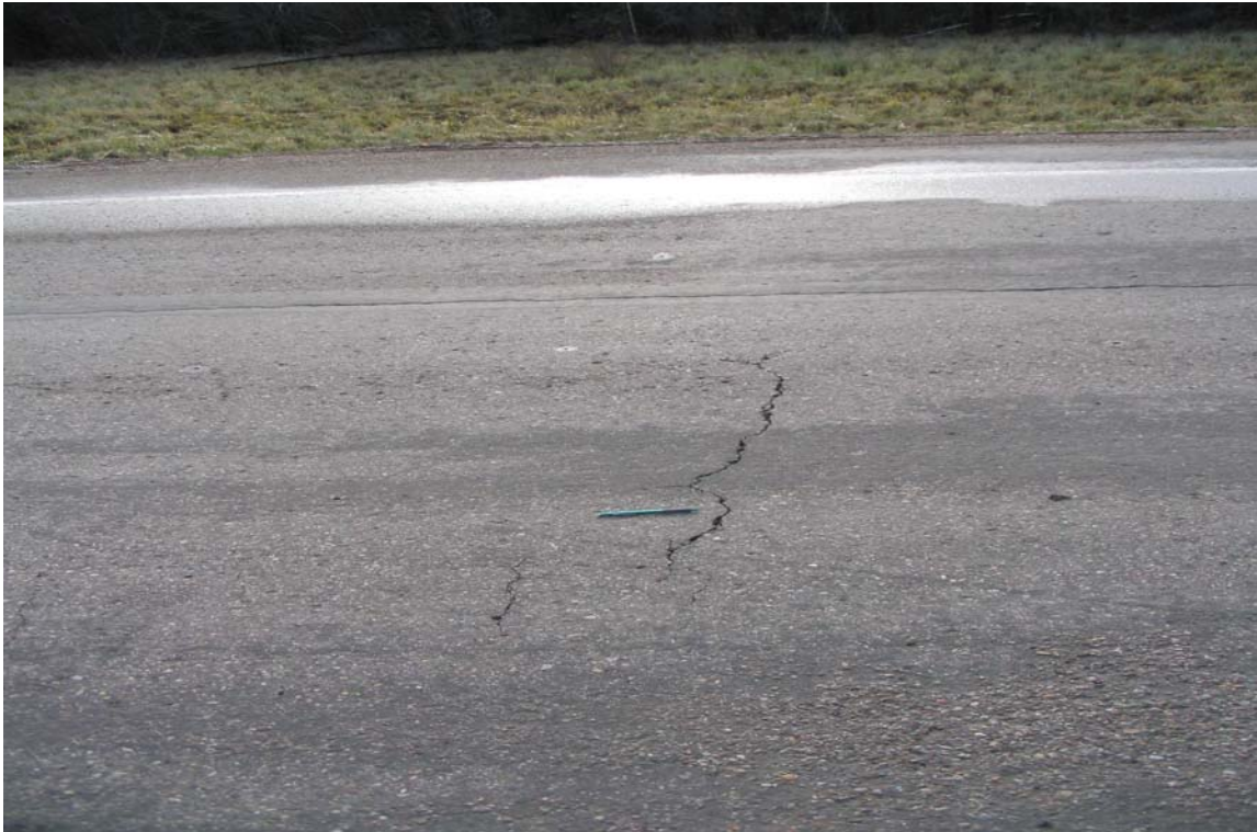
PHOTO 5: New transverse cracks in pavement at Site A.
