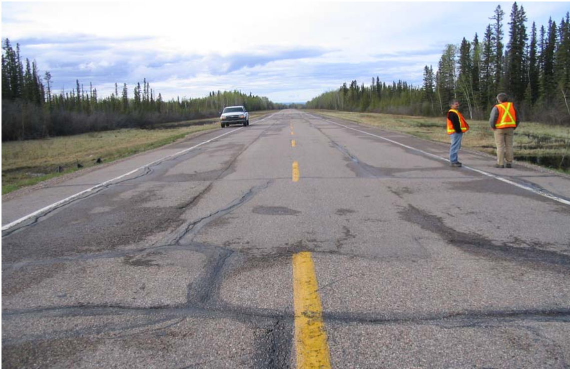
PHOTO 1: View of Site A facing north. Reopening of cracks previously patched on the pavement.
