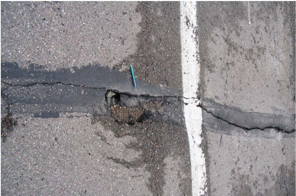
PHOTO 4: Hole on the roadway and transverse cracks at Site A.
