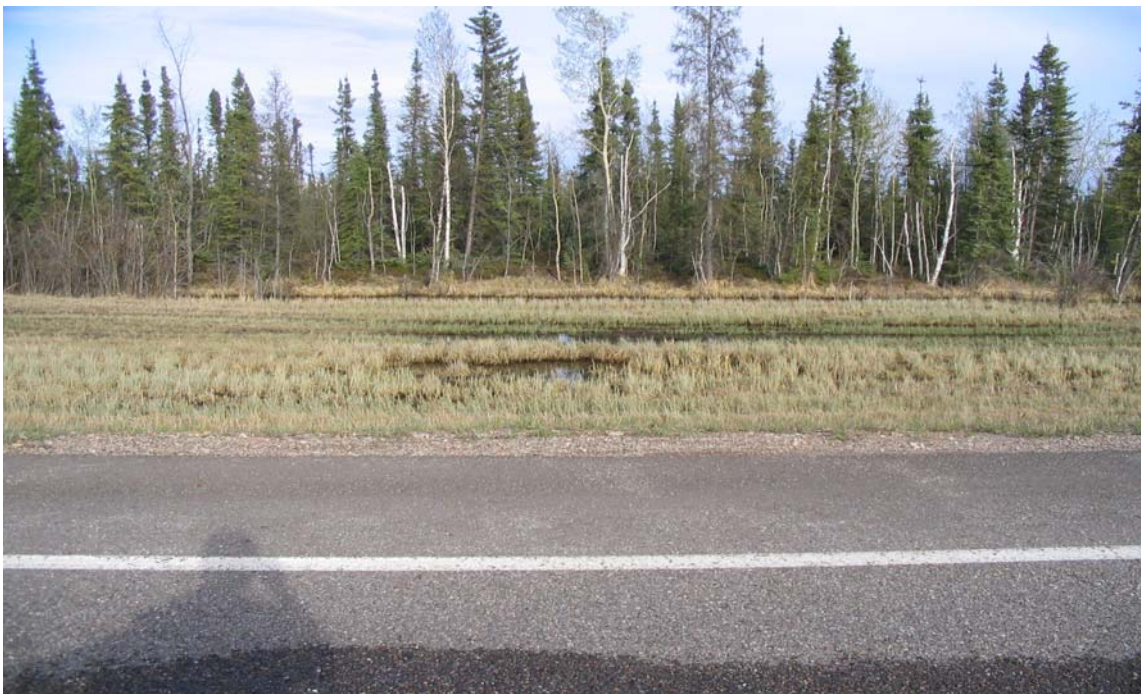
PHOTO 8: Ponded water and dip on right of way over the east side of the road at Site B.
