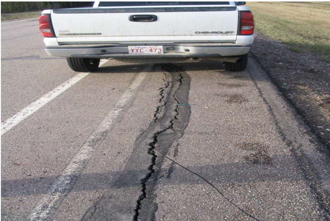
PHOTO 10: New longitudinal crack and reopening of a crack previously patched at Site B.
