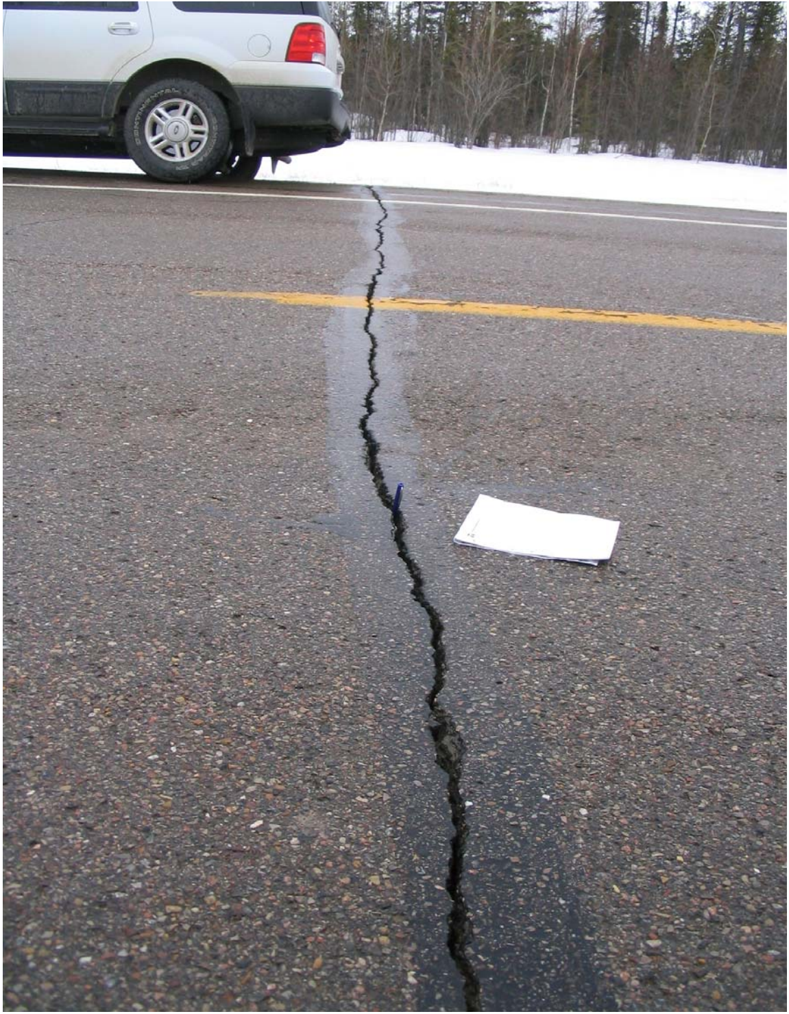
Photo 8 - Transverse crack 20 mm wide in Site B.
