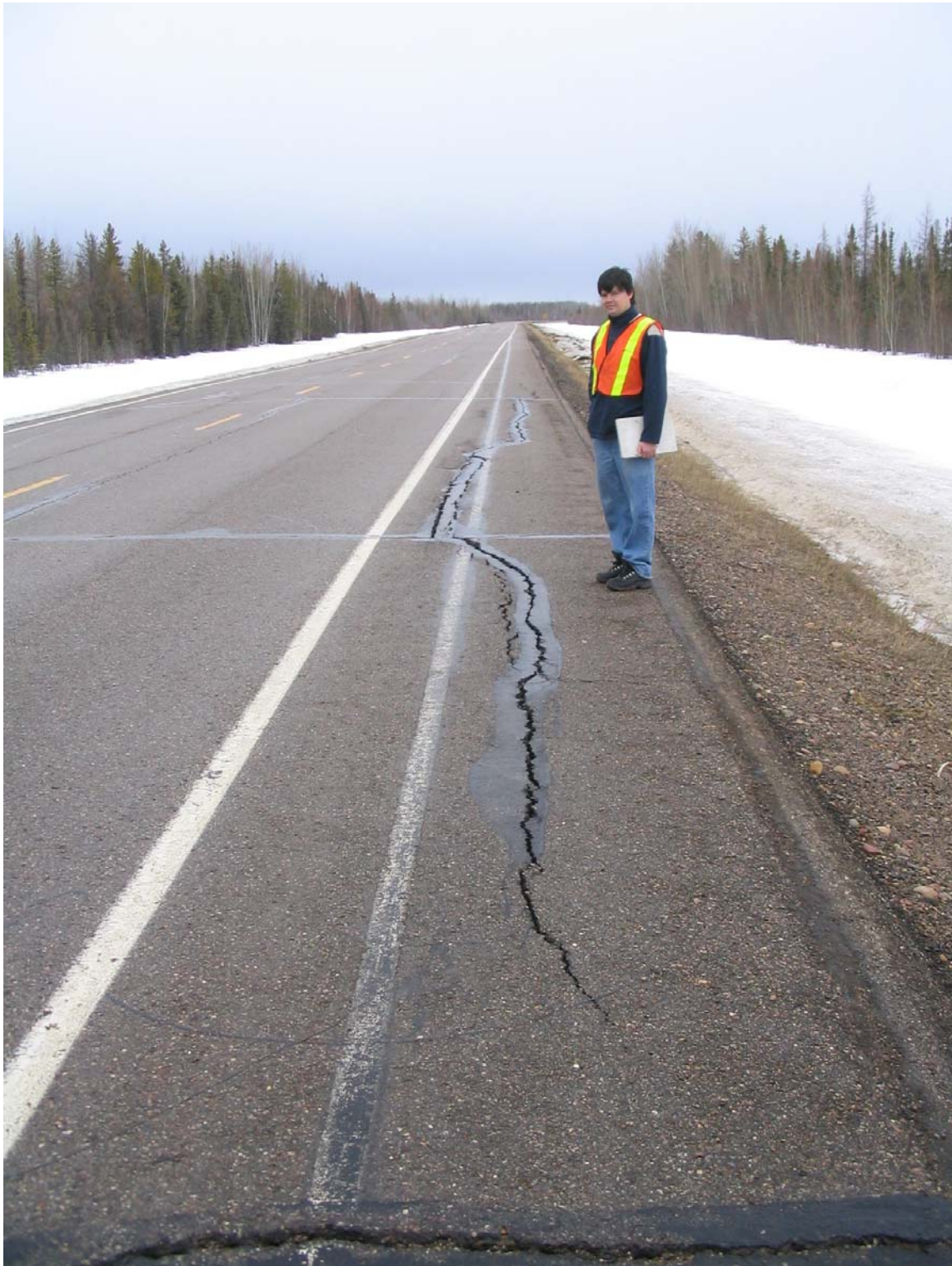
Photo 1 - Graben type crack at Site A.
