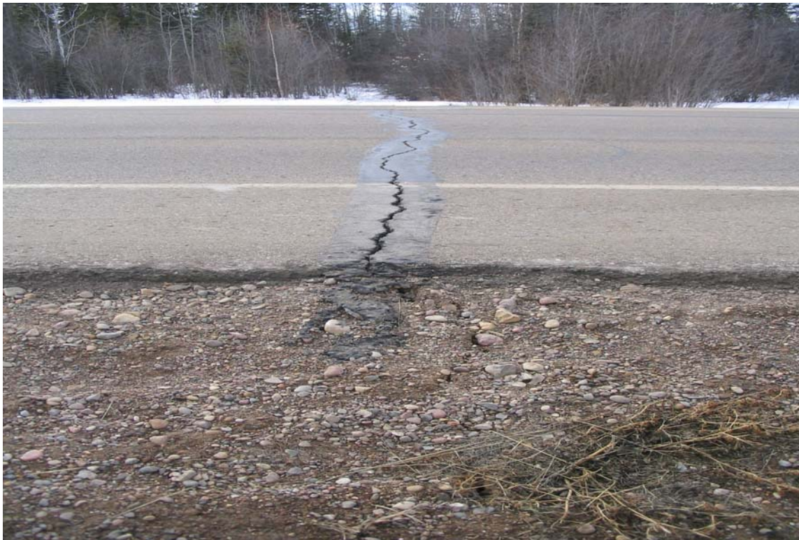
Photo 5 - Transverse crack above culvert in Site A, looking west.
