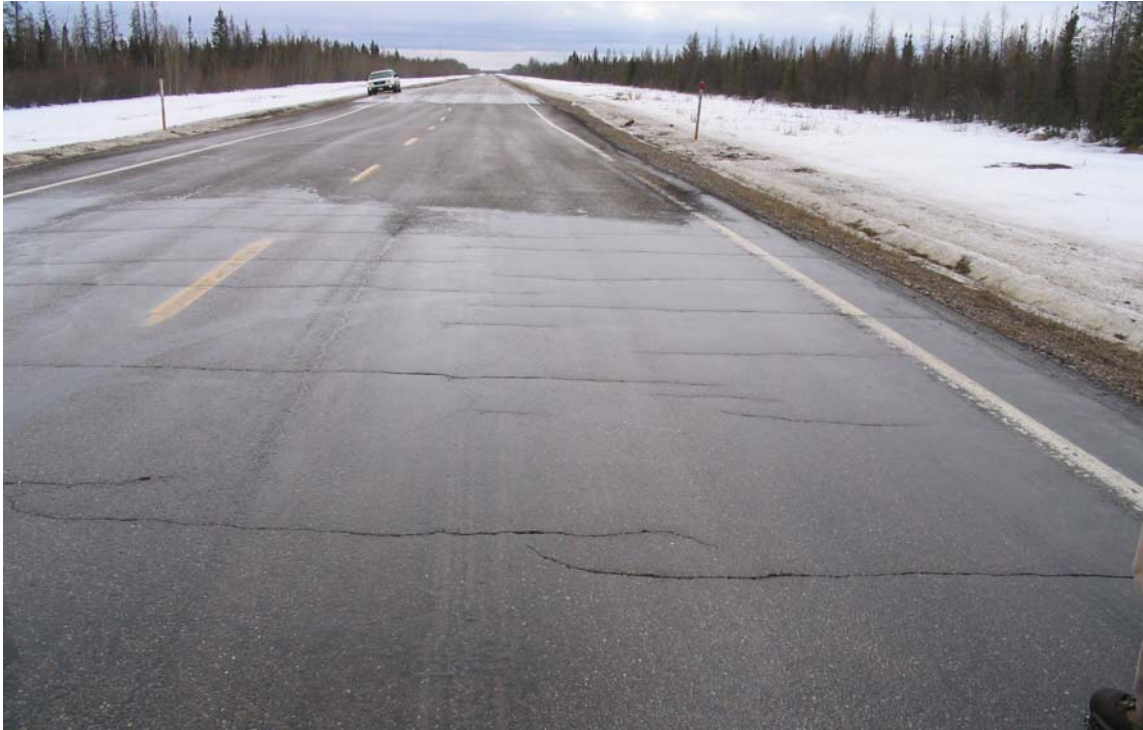
Photo 4 - Flexural cracks in old ACP patch at south end of Site A, looking south.
