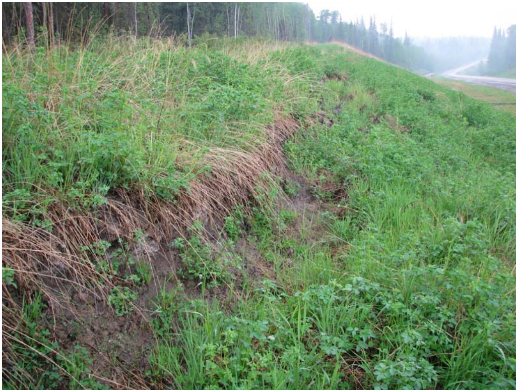
Photo 3 – Clay material along backscarp on east sideslope, looking south.
