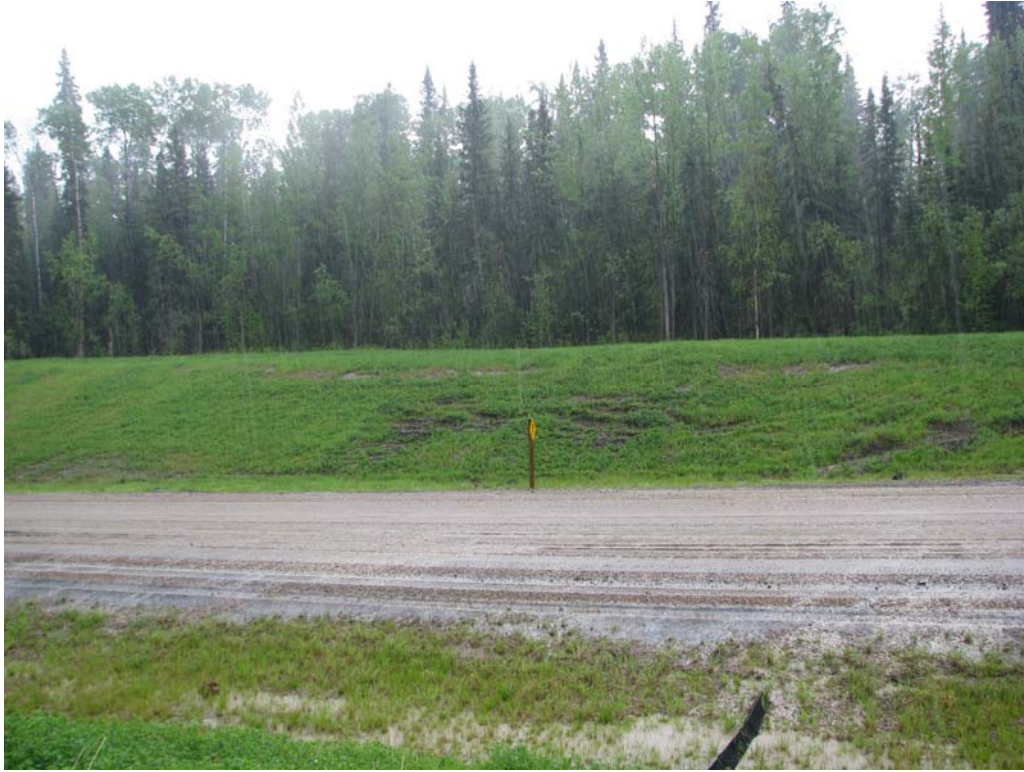
Photo 5 – Wet areas and surficial slope failures on west backslope, looking southwest.
