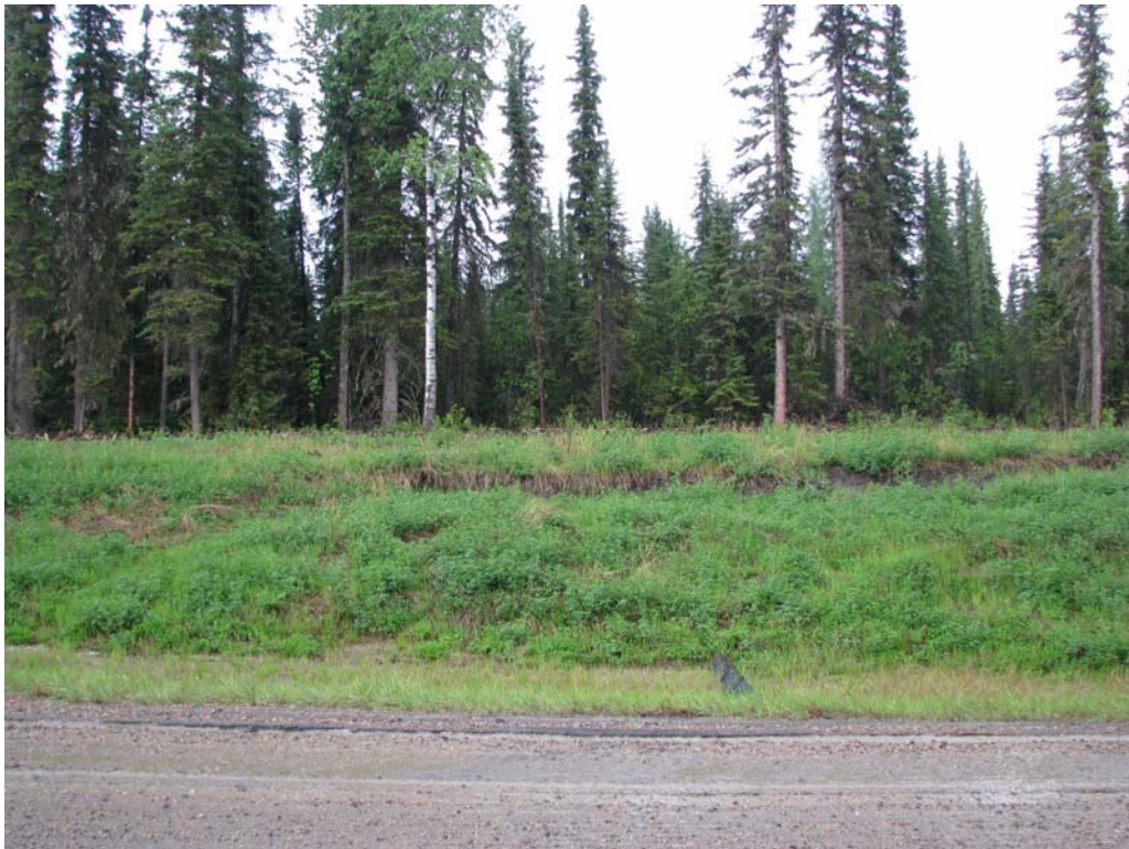
Photo 2 – Slope failure on east backslope, looking east.
