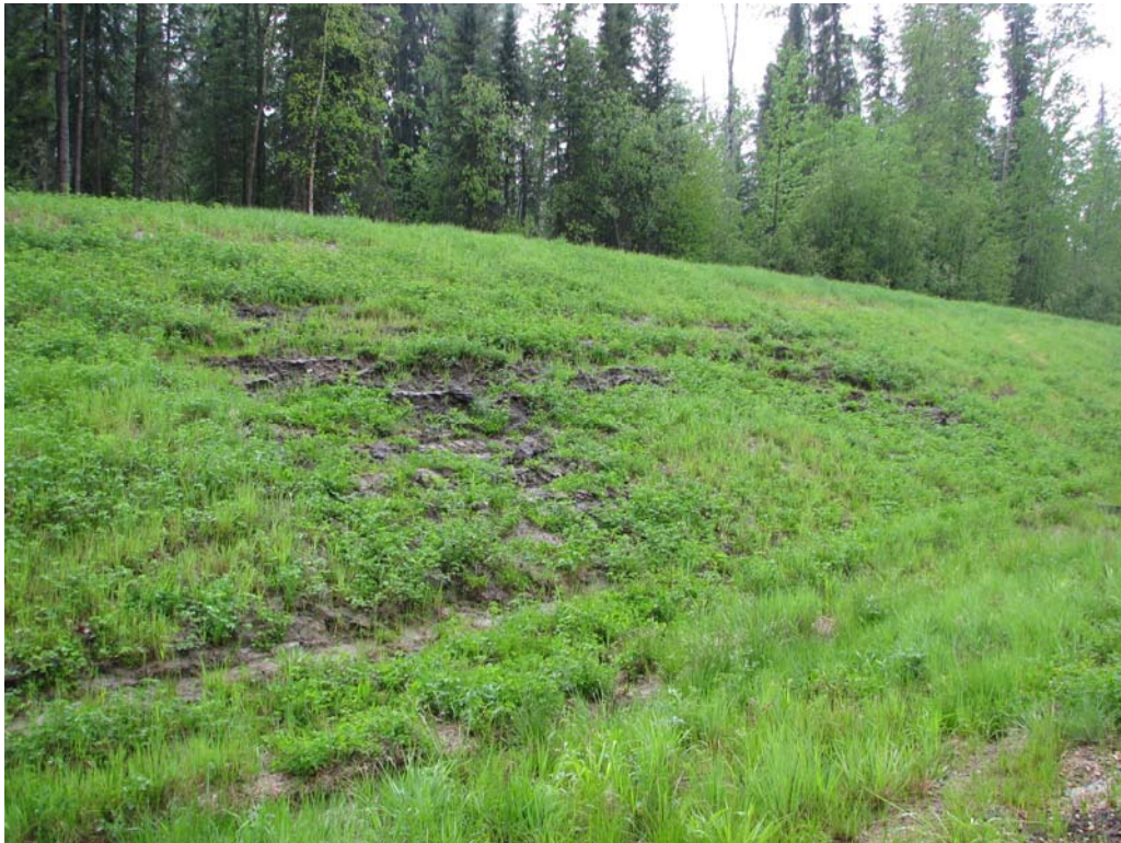
Photo 6 – Wet area and surficial slope failure on west backslope, looking west.
