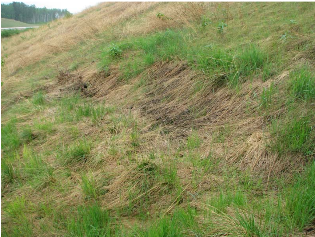
Photo 4 - View of cracks east of the site, looking east.
