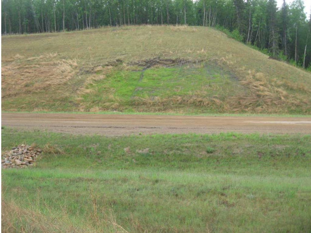
Photo 1 - View of slope failure on south backslope, looking south.
