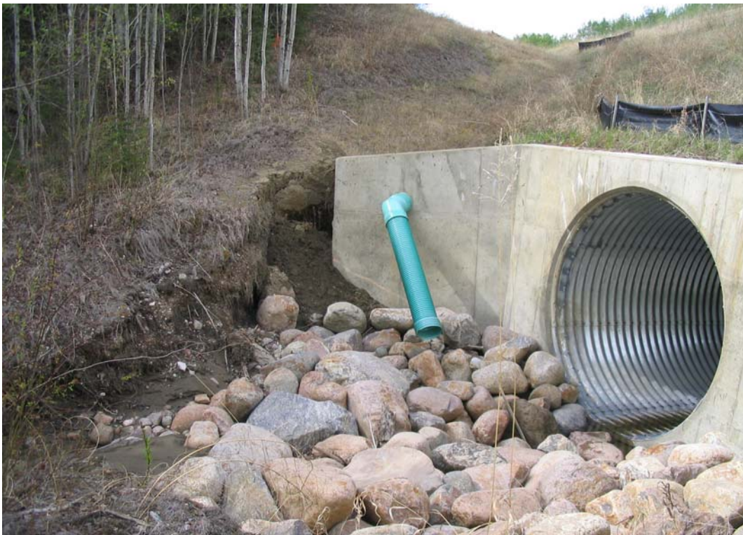
PHOTO 6: Erosion slump at the culvert inlet.
