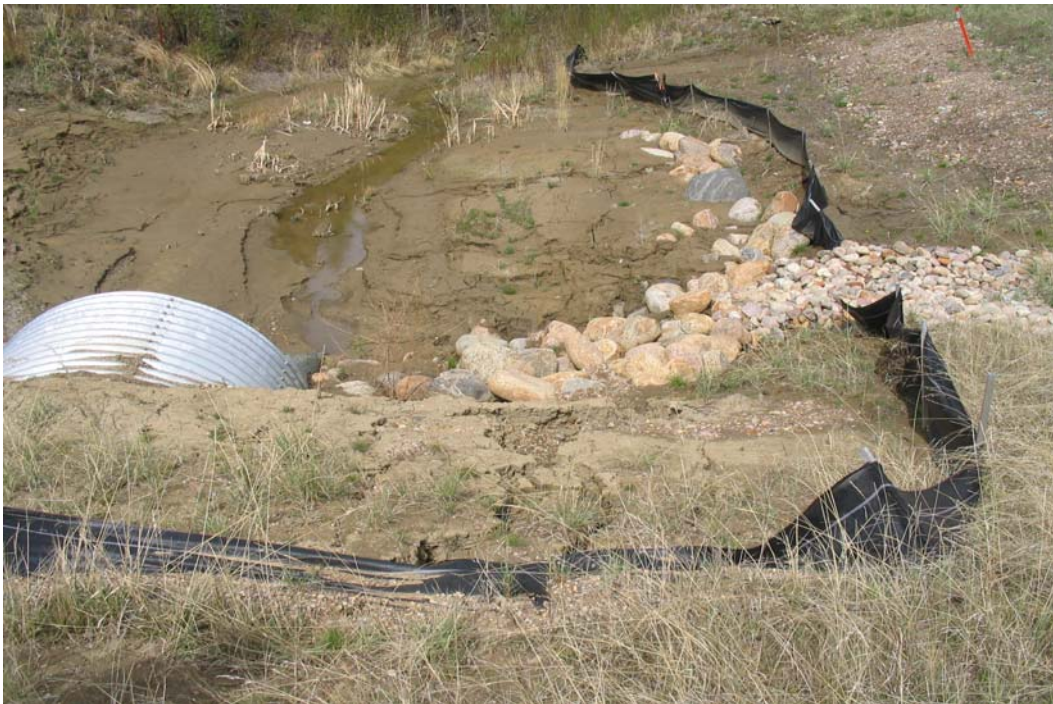
PHOTO 4: Erosion gullies above culvert outlet and accumulation of silt.
