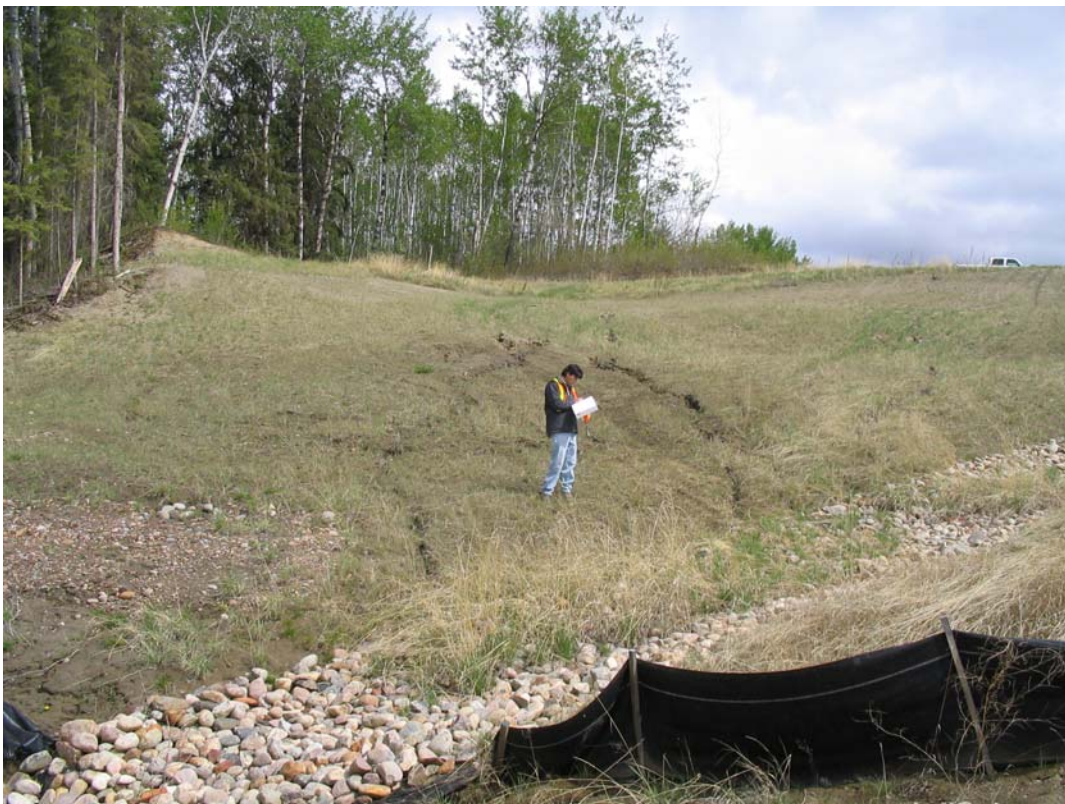
PHOTO 2: Erosion gullies on the east slope.
