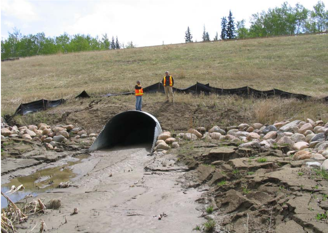
PHOTO 3: Erosion gullies above culvert outlet, damaged silt fence and accumulation of silt.
