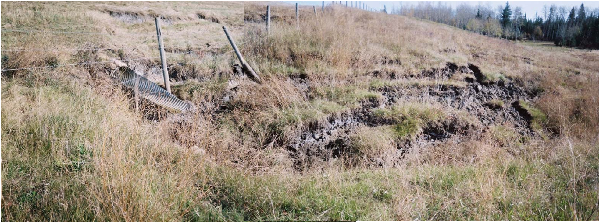
PHOTO 3 - LOOKING NORTHEAST AT EROSION / SLUMPING ADJACENT TO 800mm Ø CULVERT OUTLET
