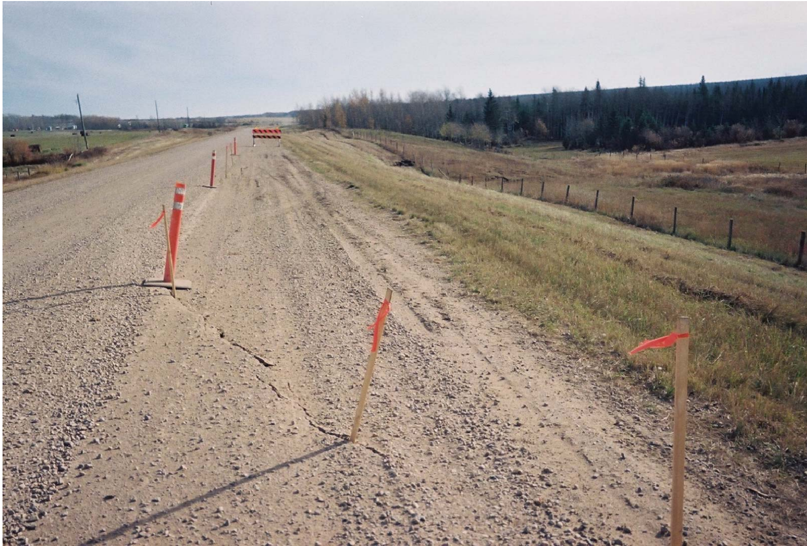
PHOTO 2 - LOOKING EAST ALONG ROAD AT CRACK IN HIGHWAY. THE PILONS MARK THE SLIDE SCARP BOUNDARY
