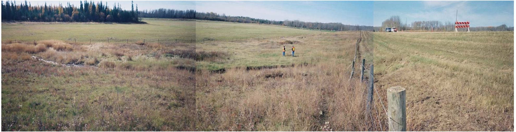
PHOTO 4 - LOOKING SOUTH TO WEST ACROSS SLIDE AREA FROM EAST END OF SLIDE. NOTE BOWED FENCE AND TWO DEBRIS PILES
