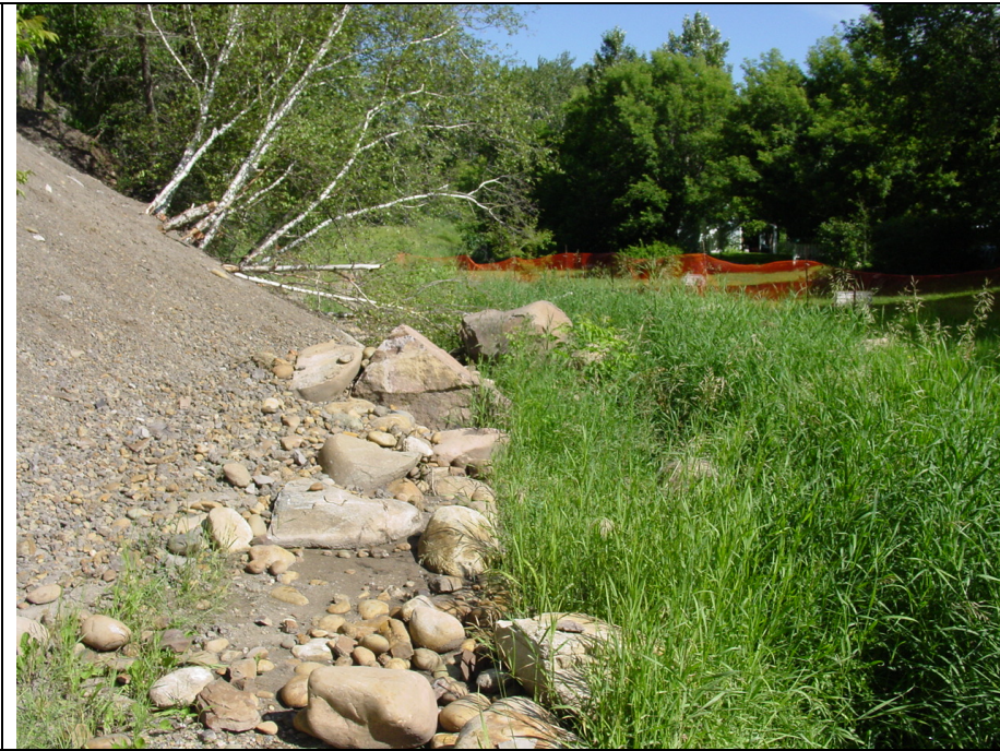
Photo 6. Debris at toe of slide area.
