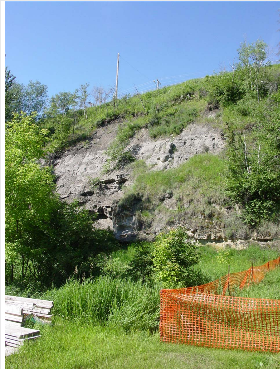
Photo 9. Typical slopes south of the slide area. There have been past failures in this area, and there is cracking near the crest of the slope.
