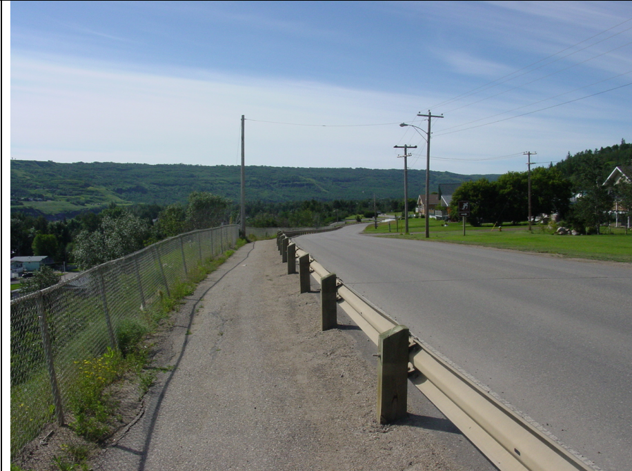
Photo 7. Tilted fence and cracks in the path immediately south of the slide area. The telegraph pole in the middle distance doesn't show signs of tilting (the support wire isn't taut).
