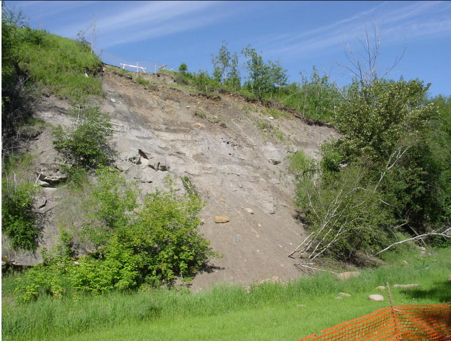
Photo 5. Slope in failed area. Note the stratigraphy is silty sandy clay with up to boulder sizes overlying sandstone, which forms the cliffs in the lower portion of the slope. Overall slope height is ~20 m. Note the surface failure just above the soil-rock interface to the north of the slide (right of picture)
