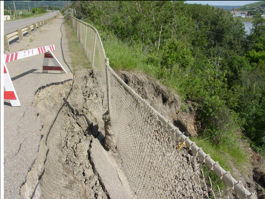
Photo 2. Looking north at scarp in the path along Shaftsbury Trail.
