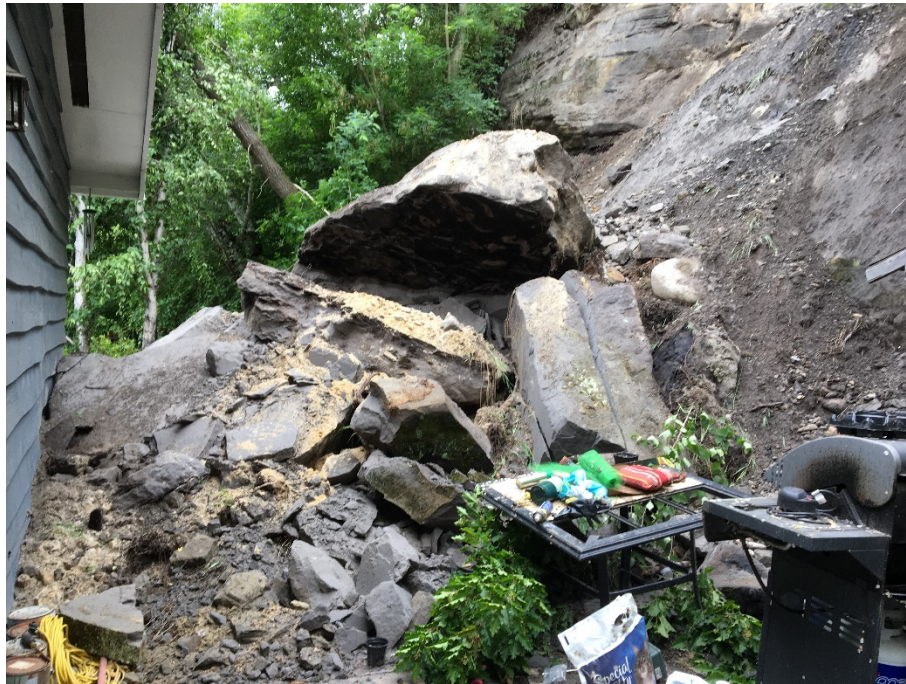
Photo 8: Looking south at sandstone slabs at the toe of the slide.
