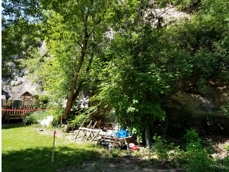
Photo 7: Looking southwest towards the toe of the slide
