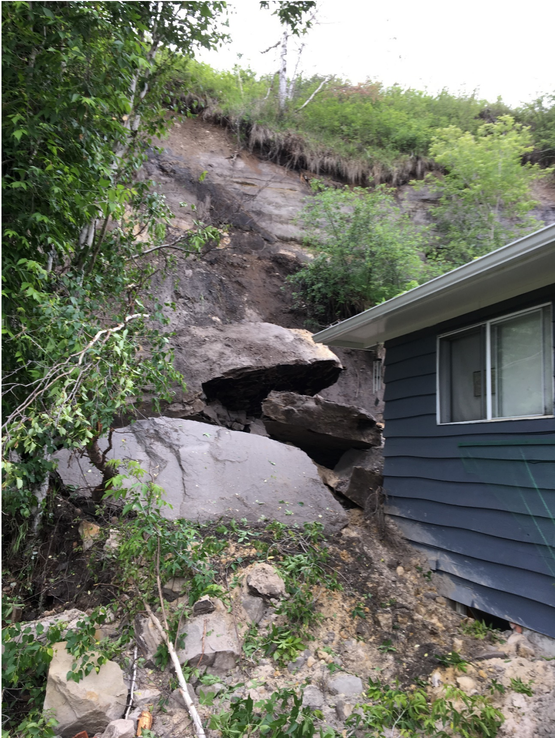
Photo 9: Looking northwest at the slide from the toe
