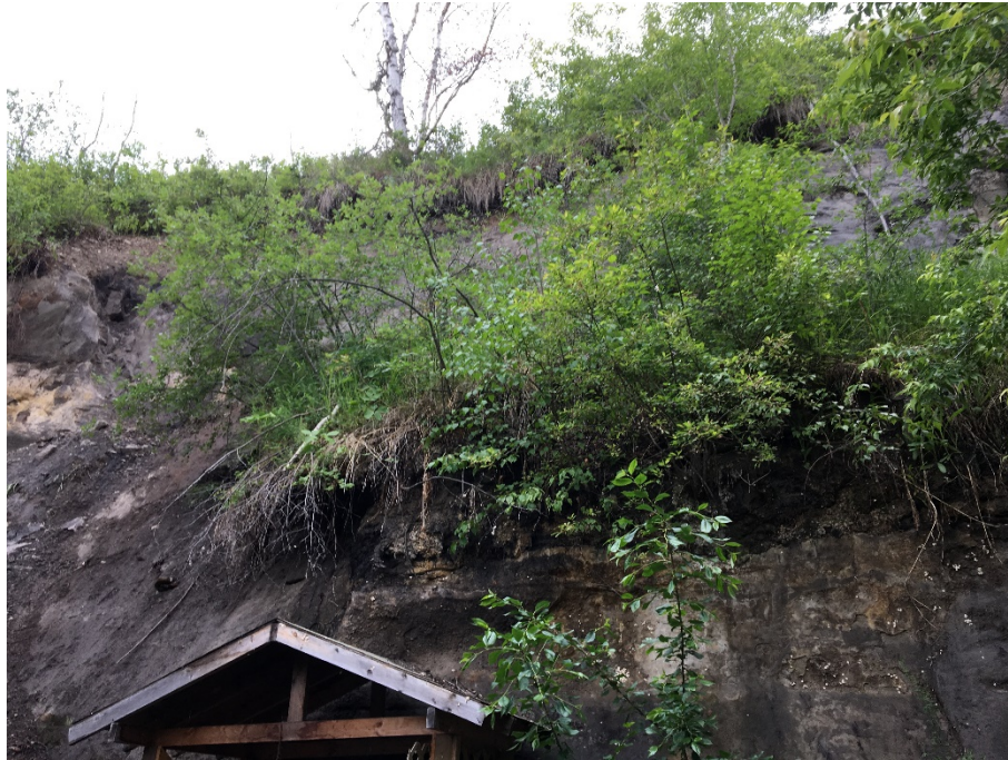
Photo 10: Looking west at upper weathered sandstone layer that did not shear and fall
