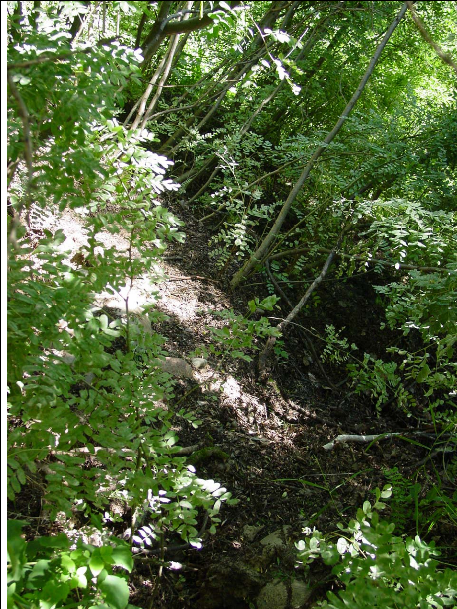
Photo 3. Crest of the slope above the Cartier residence slide.
