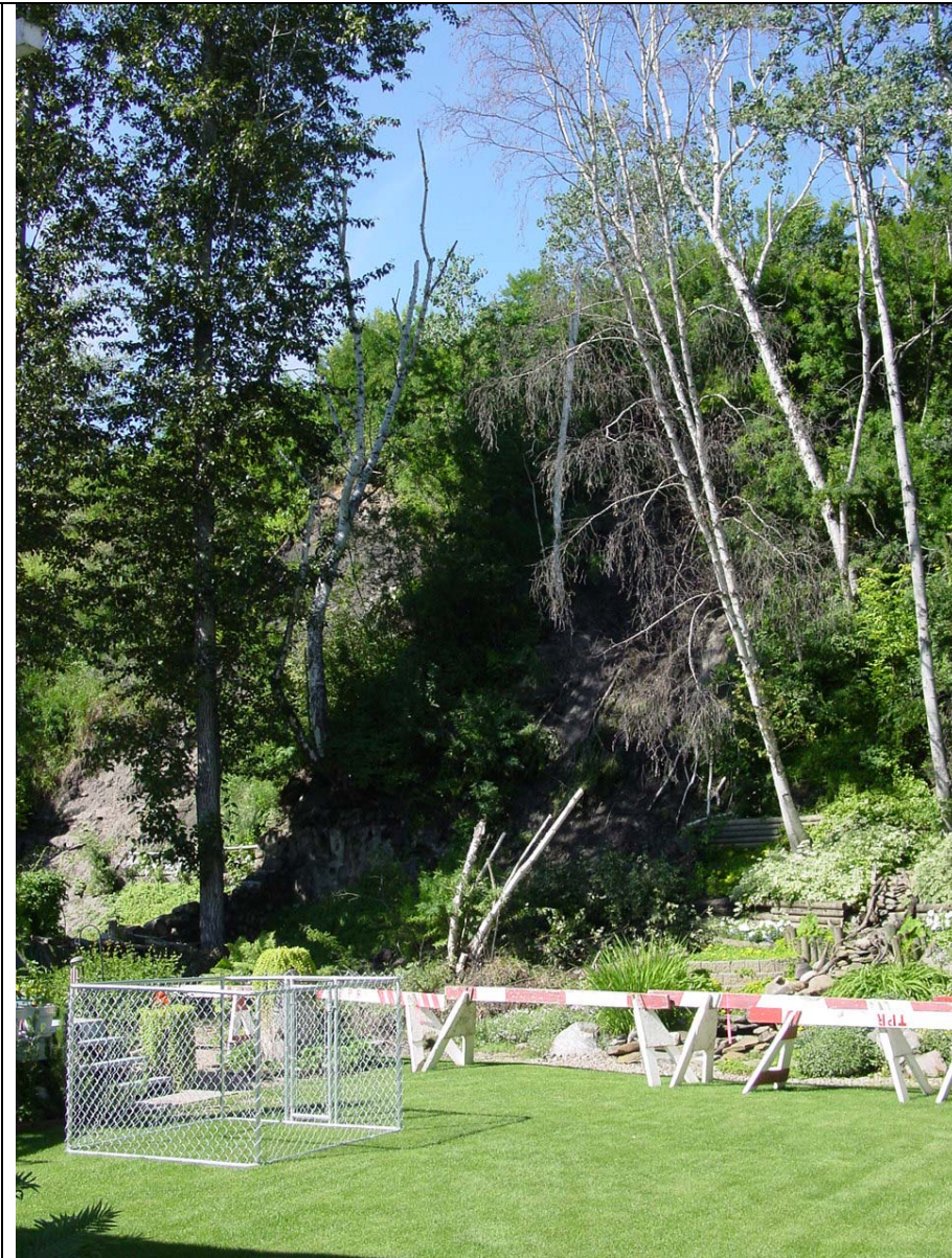
Photo 1. Cartier residence slide. Debris from the slope has entered the developed area below. Note some apparently dead trees on the slope.
