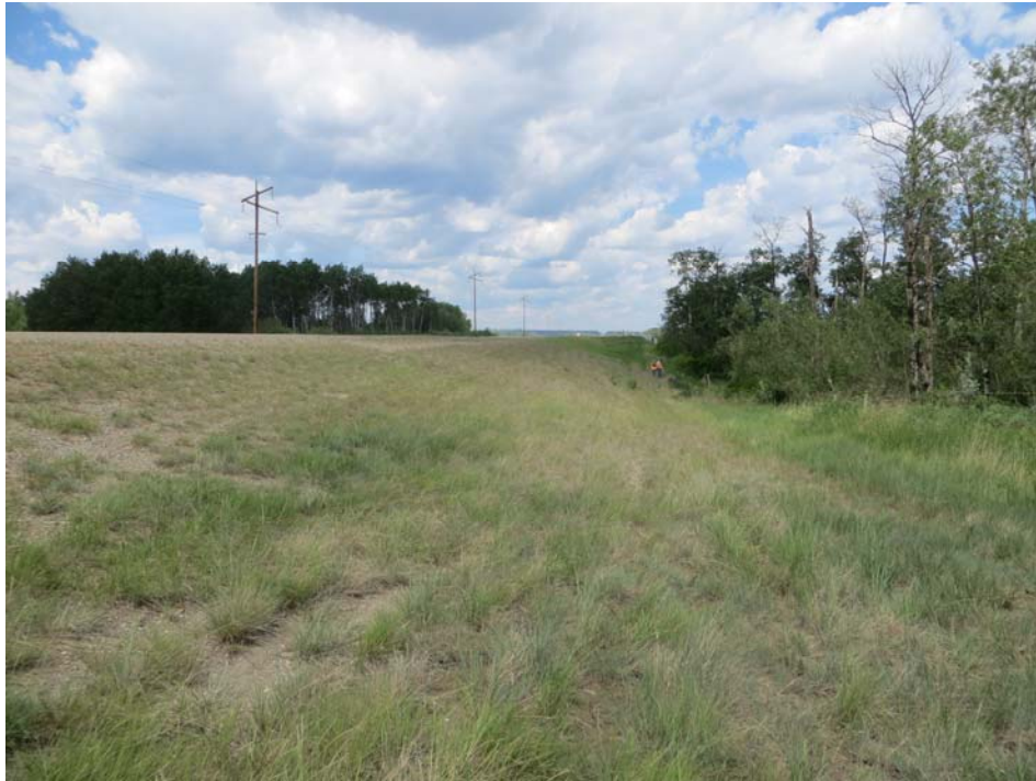
Photo 5 - Looking north at the sideslope of the highway embankment at the former Bogey Slide
