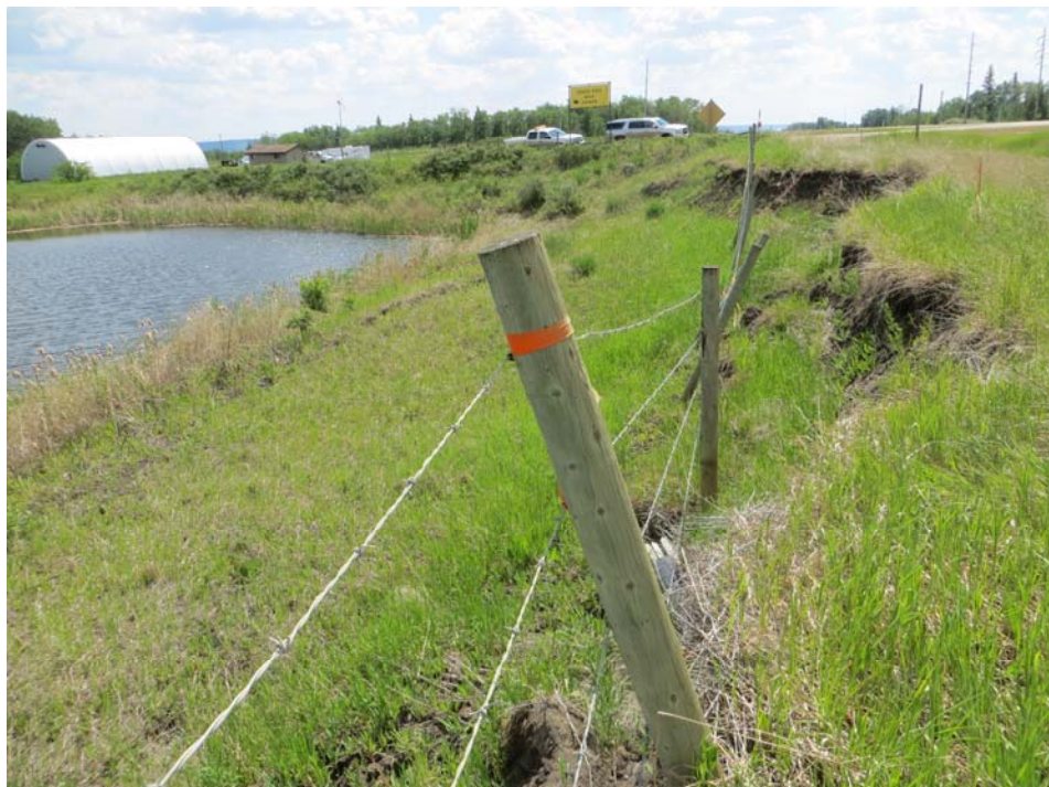
Photo 2 - Looking south at the failed pond slope (Double Bogey Slide).
