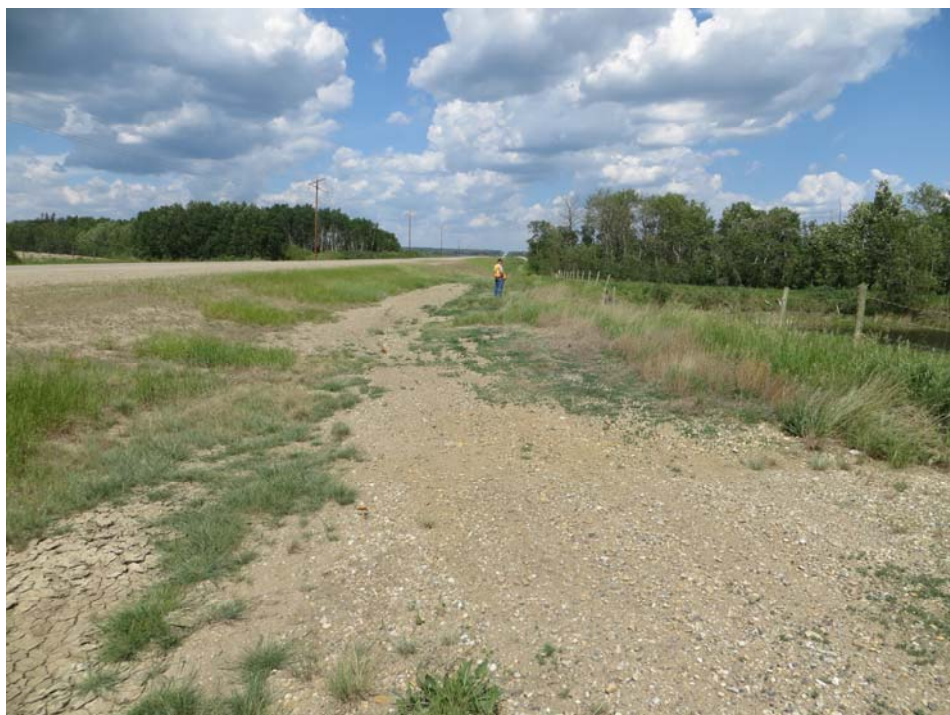
Photo 4 - Looking north at the bench between the highway and failed pond slope (Double Bogey Slide).
