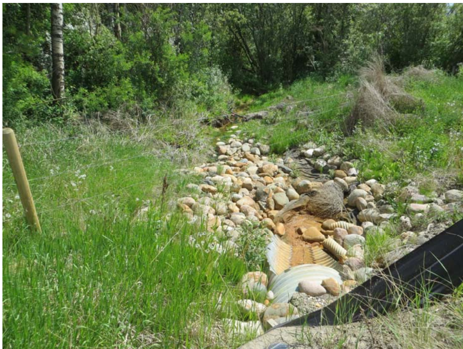
Photo 6 - Looking east at the culvert and subdrain outlets at the Bogey Slide Repair
