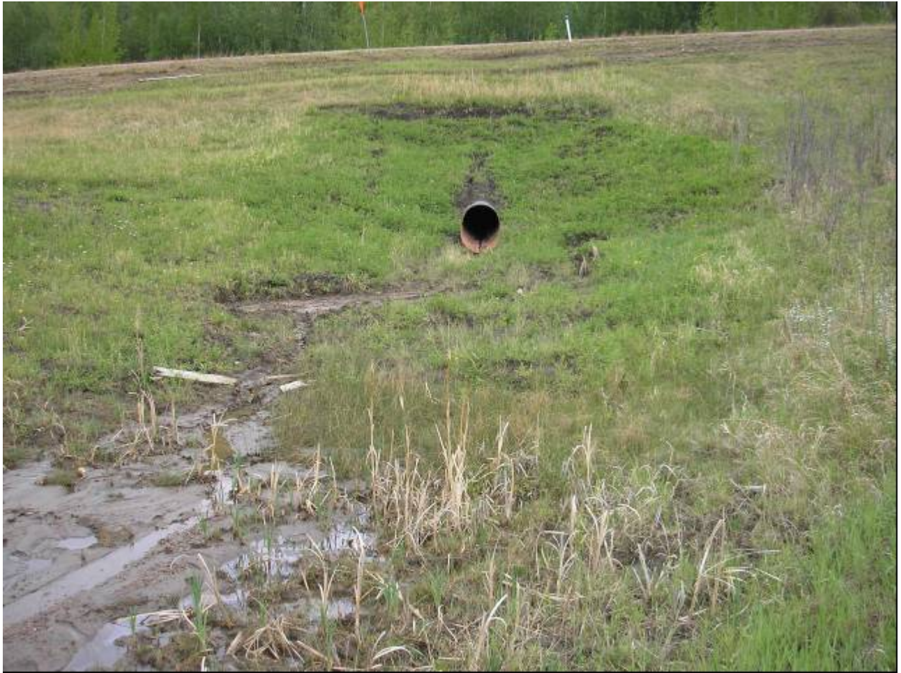
Photo 2 - Looking east at minor erosion in downslope of the new 900 mm dia. culvert outlet area. Note the open hole to right of culvert that marks improperly grouted old culvert (seepage emanating from open hole), May 24, 2006.
