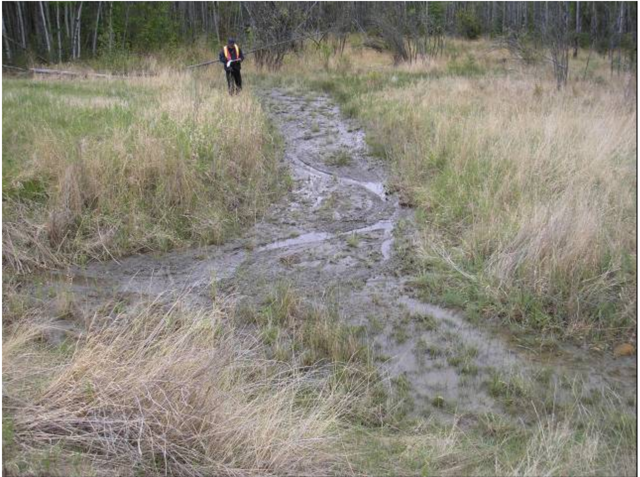
Photo 5 - Looking west at enlarged silt buildup area, May 24, 2006.
