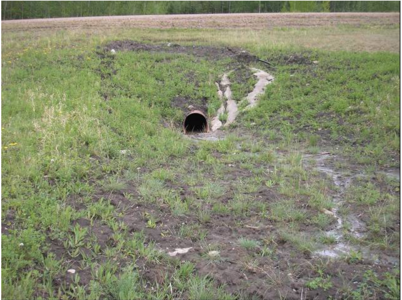
Photo 1 - Looking east at a small slump above the new 750 mm diameter culvert outlet area and minor erosion in unvegetated area further downslope, May 24, 2006.
