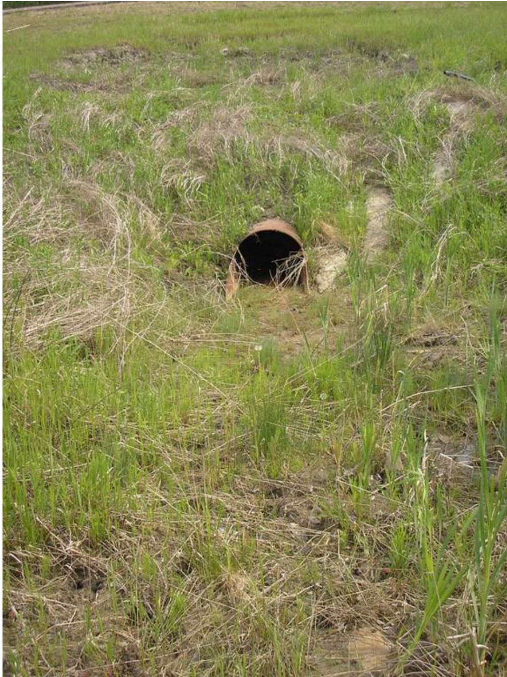
Photo 1 - Looking southeast at a small slump above the new 750 mm diameter culvert outlet area, June 14, 2007.
