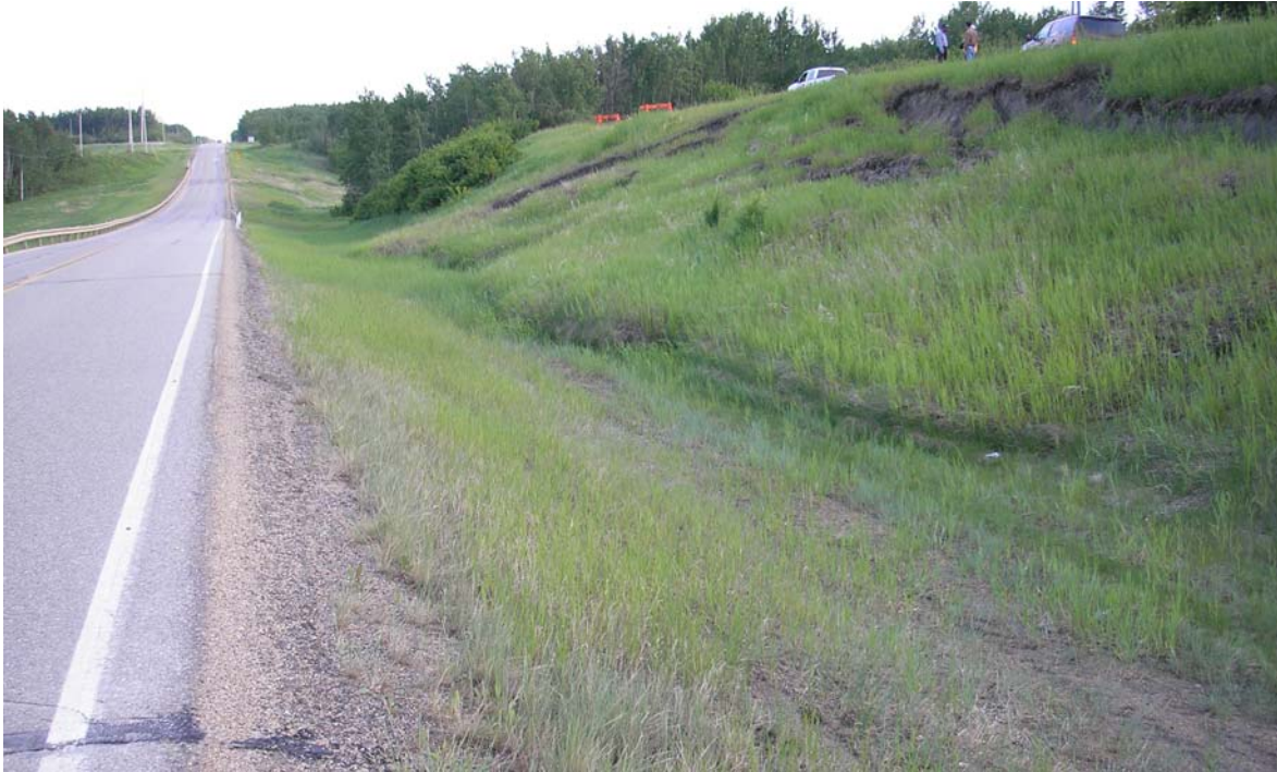
Photo 3 – Looking south along highway ditch at slide area.
