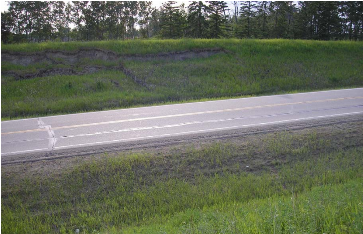
Photo 4 – Looking west at north end of Slide 2.
