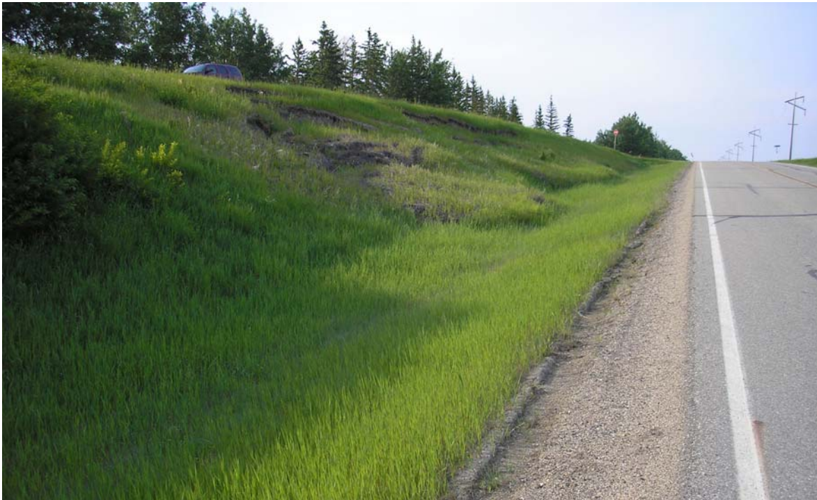
Photo 2 – Looking north along highway ditch and toe of Slide 2.
