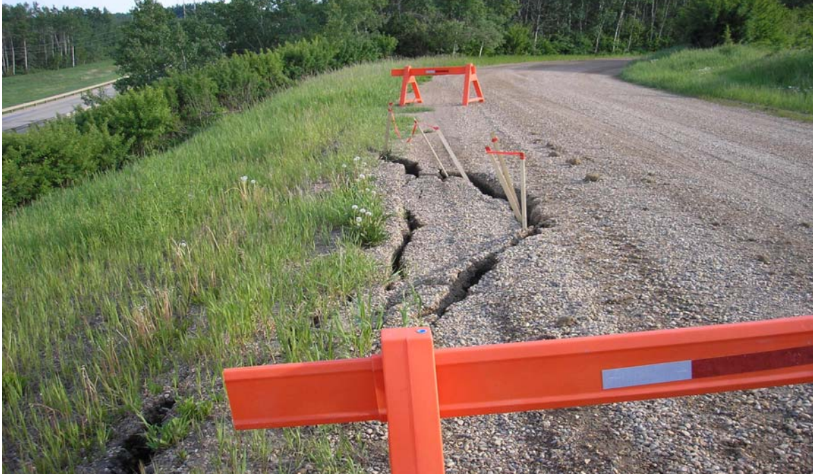
Photo 1 – Looking south at Slide 1 along edge of Twp. Road 822.
