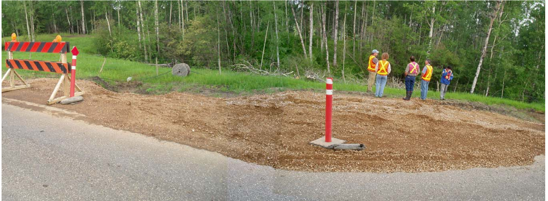
Photo 2: Looking northwest at slumped area from edge of highway embankment.
